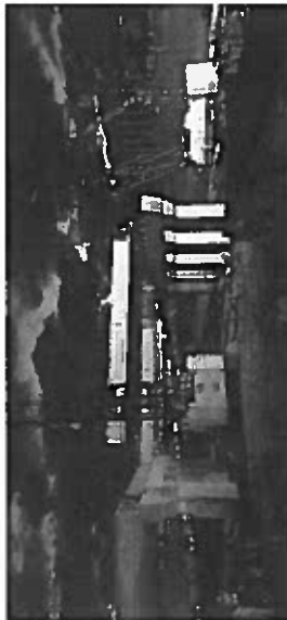
The Wisconsin Zoo Interchange Project is a large scale project with significant impacts of alleviating traffic congestion. The 5th Street bridge is rebuilt in the photo above. Source: WisDOT
