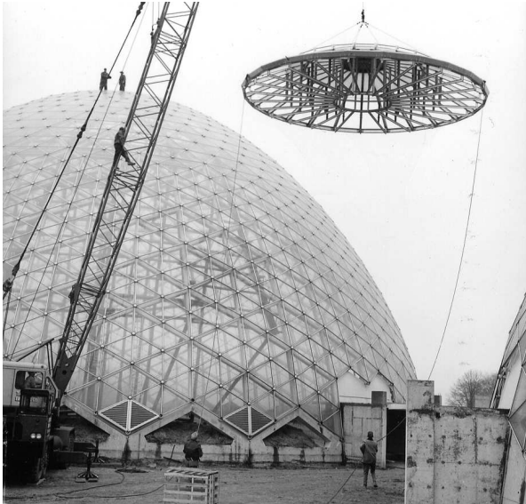
Figure 3 Photograph of the apex installation at the top of a dome. (Milwaukee County Parks Historic Photograph Collection)
