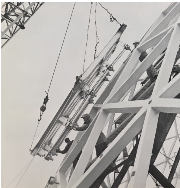
Figure 4 Photograph showing a pre-assembled glass panel being lifted into place. The hubs connect the glass to the concrete at designated points (dark squares). (Printed in Mitchell Park Horticultural Center guidebook ca. 1968)
