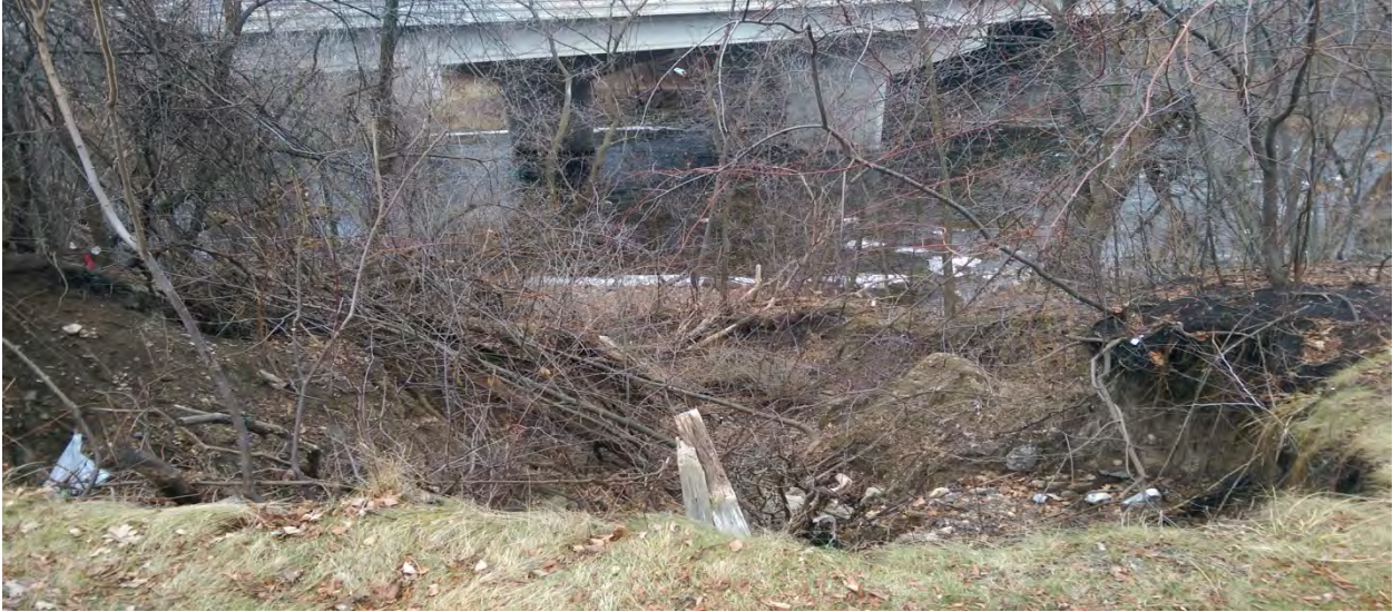
Image 2: Main erosion slump caused by 2010 severe storm.
