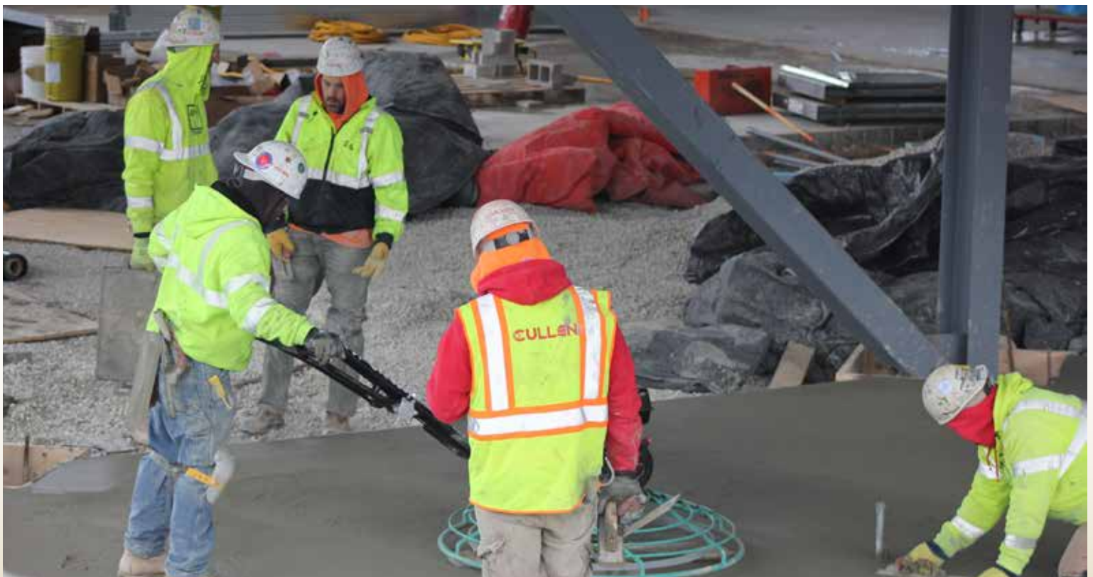
J. P. Cullen & Sons, Inc. workers laying concrete on the McKinley Health Center project.
