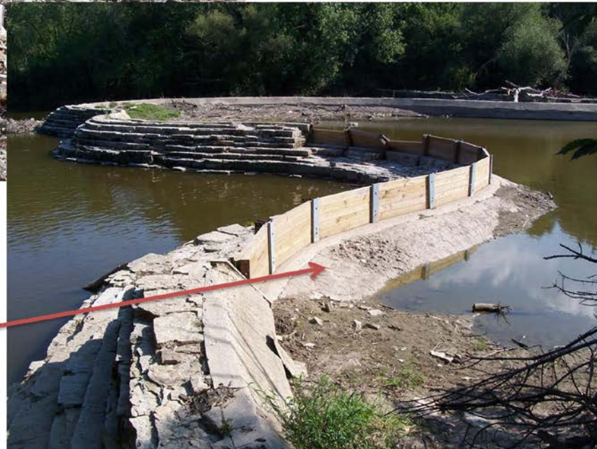
Spillway After July 22, 2010 (Taken 8/12/10)
