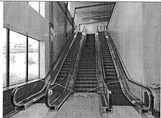
Escalators to Second Floor
