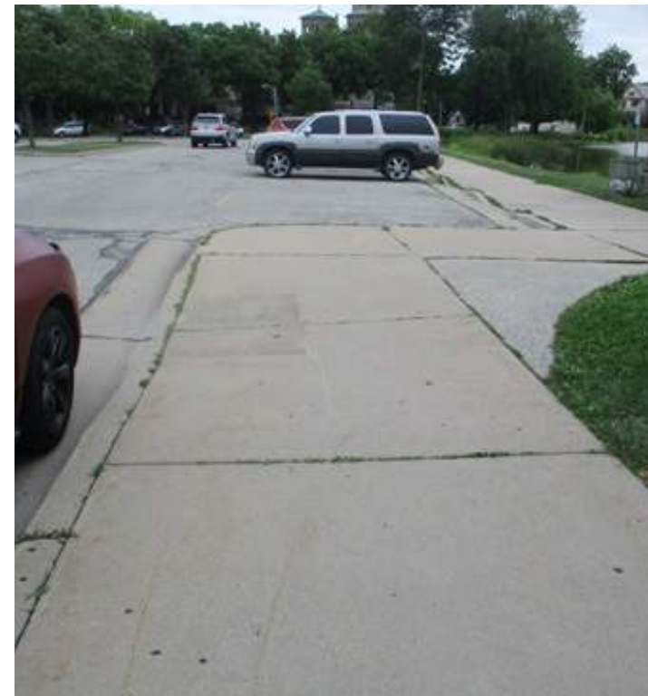
Typical non-compliant handicap sidewalk ramp
