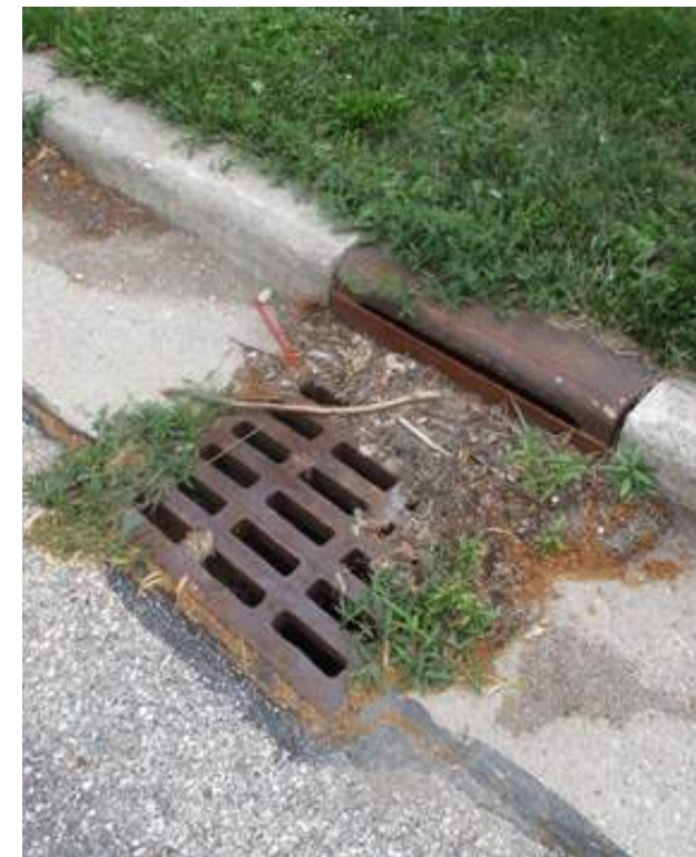
Typical storm inlet in need of cleaning
