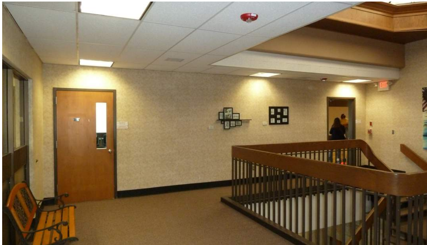
Existing lighting original to the 1980 design
