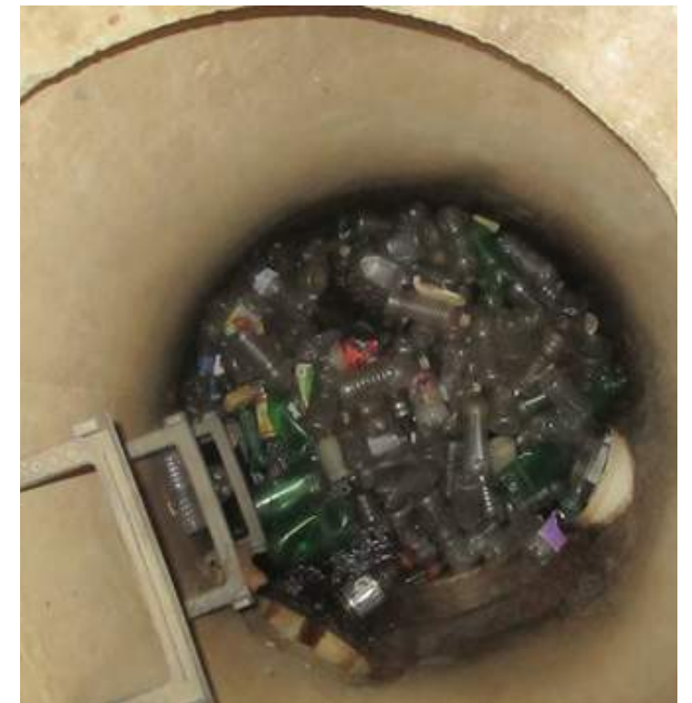
Typical storm manhole in need of cleaning
