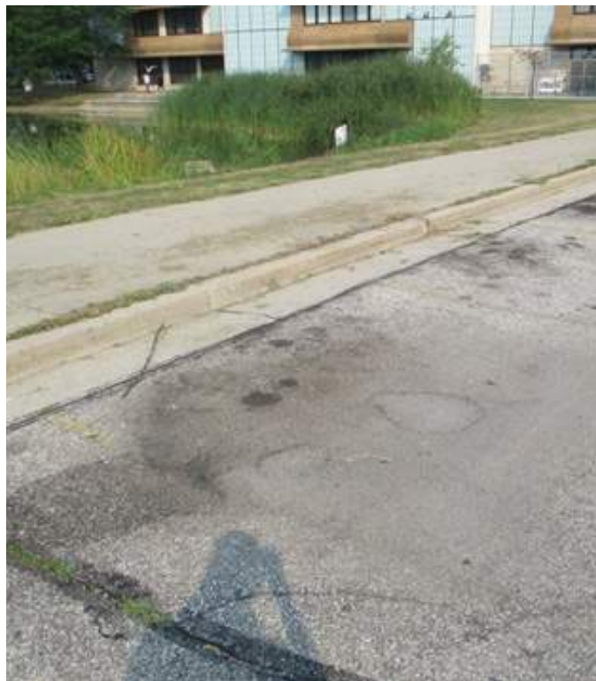
Area of localized ponding
