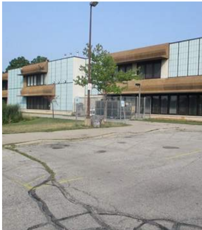
Handicapped parking stalls – note lack of signage and markings; non-compliant handicapped ramps
