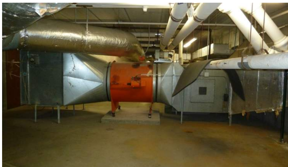
Existing air handling unit in the basement
