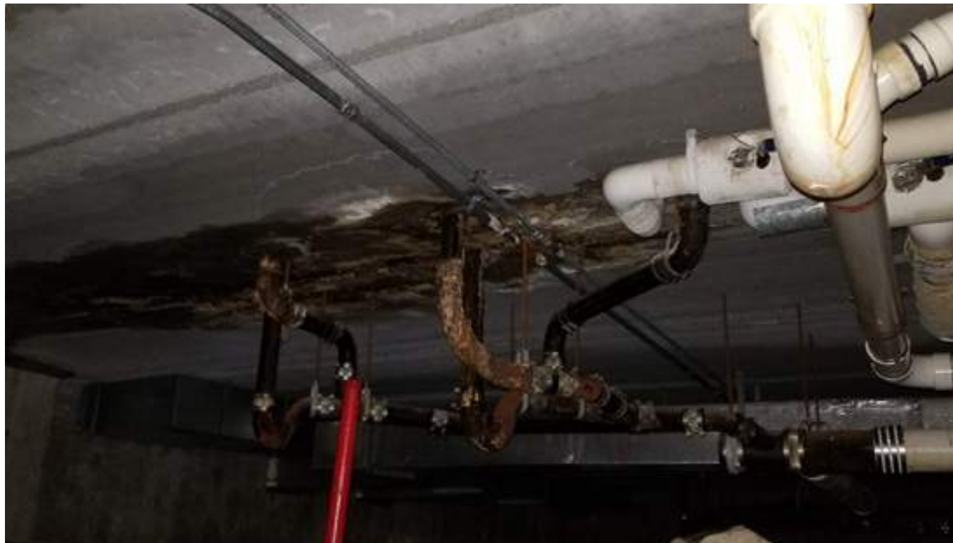
Photo 3: Precast Panel Cracking
