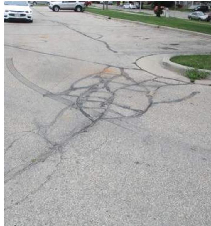
Typical area of cracked asphalt pavement
