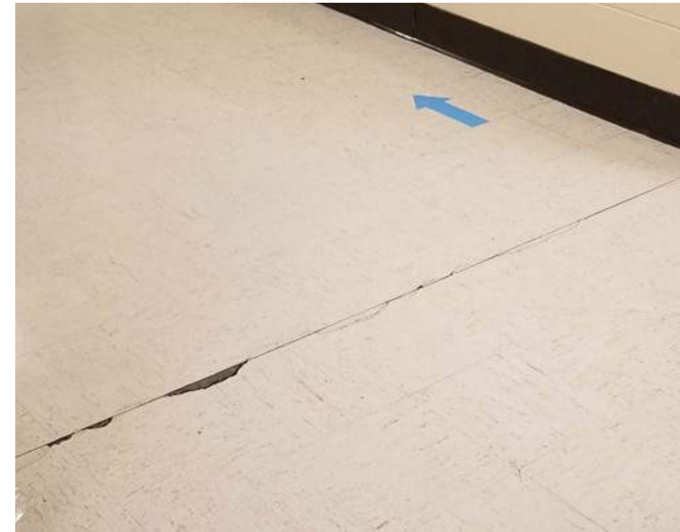
Photo 4: Floor cracking in Ground Level Corridor
