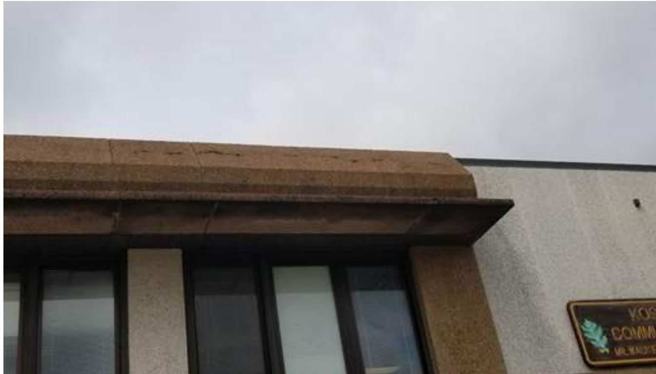
Photo 1: Precast Panel Cracking
