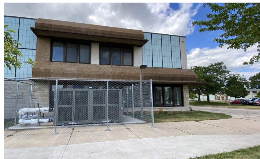
Replacement air-cooled water chiller installed in 2018 on the exterior
