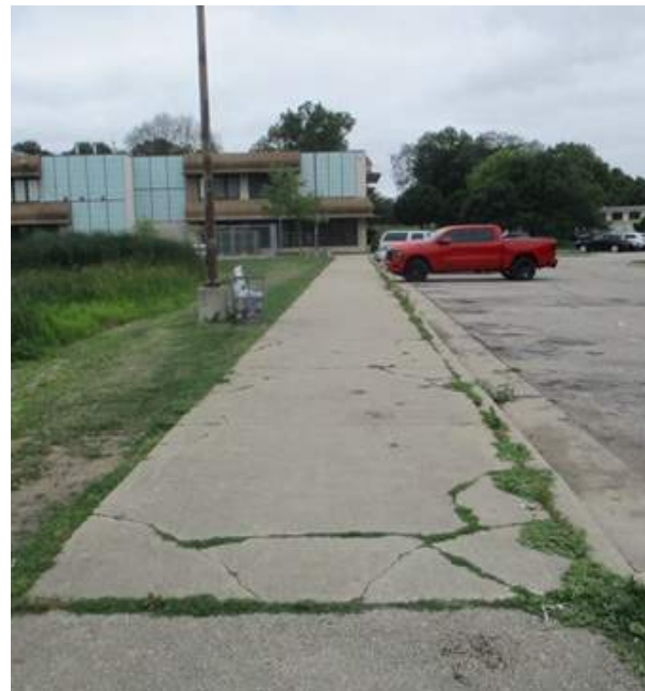
Cracked sidewalk squares
