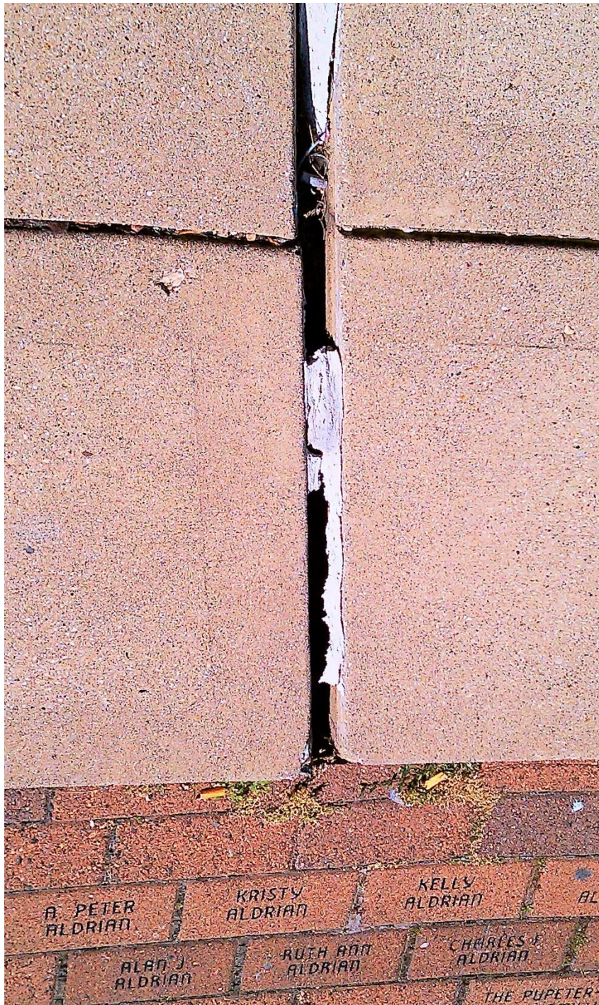
Shifting and expansion of the property left large gaps in the plaza level walkway, like the one shown above, which are potential tripping hazards.
