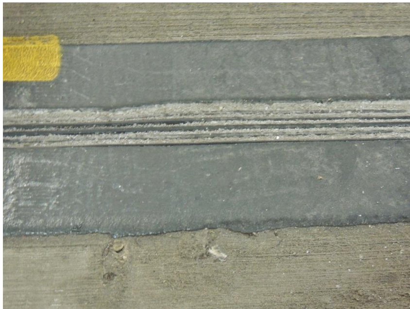
Expansion joints throughout the garage were repaired or replaced in 2011, and remain in good shape.
