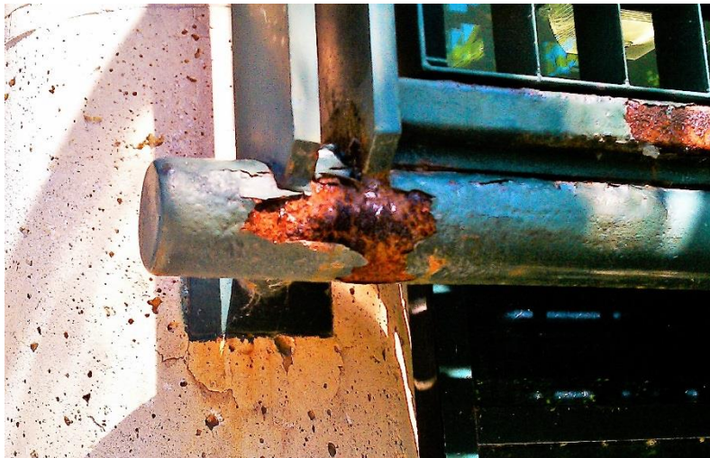
Another railing along the plaza was rusting out.
