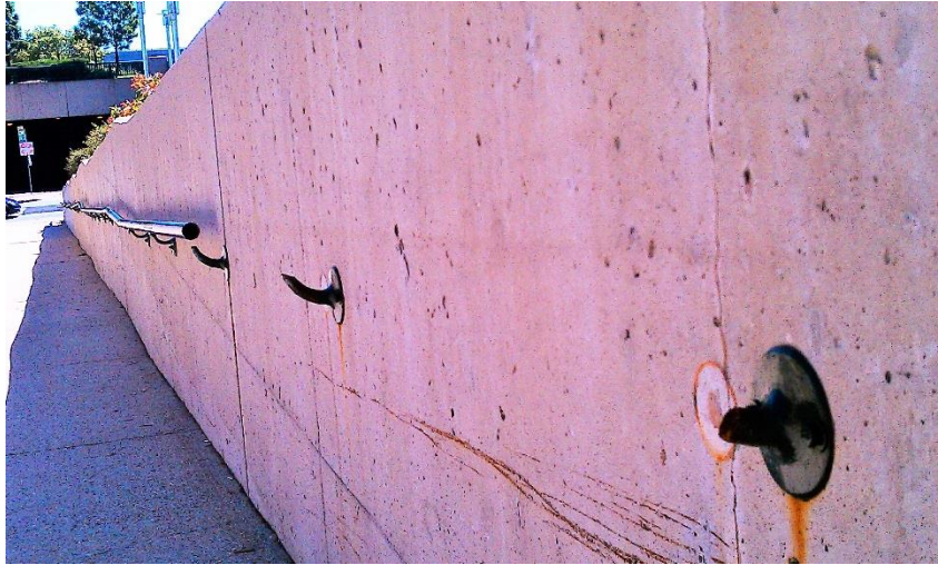
One of the property's ramps was missing a large portion of the hand-rail.
