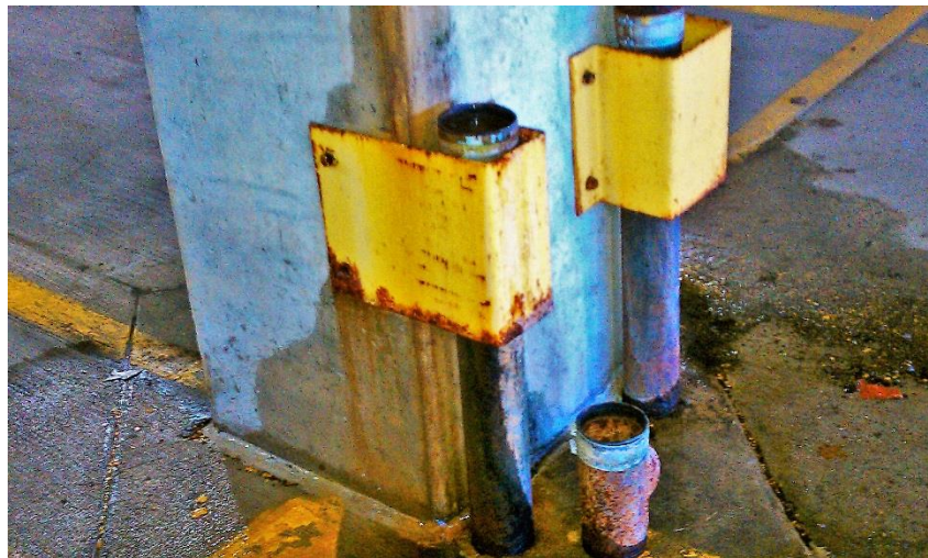
Pipes were disconnected and missing sections, which resulted in visible water damage.
