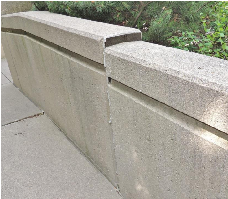
Significant settling on the property has caused part of a ramp wall, leading to the Mason Street Bridge, to separate and sink.
