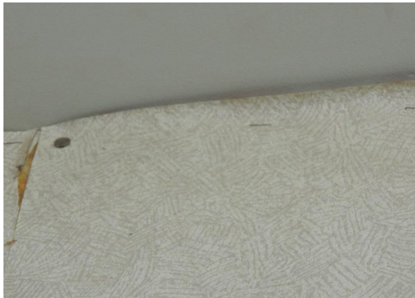
Upon closer examination, we observed that the wallpaper seam along the ceiling was being held up by thumbtacks and staples.
