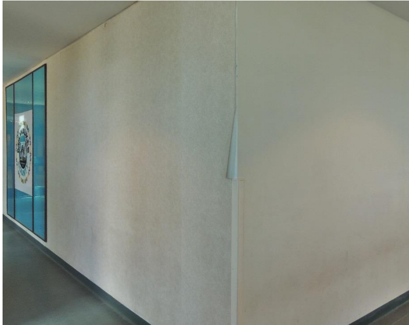
Wallpaper is peeling along a wall in the Miller Brewing Company Pavilion hallway leading to the atrium.
