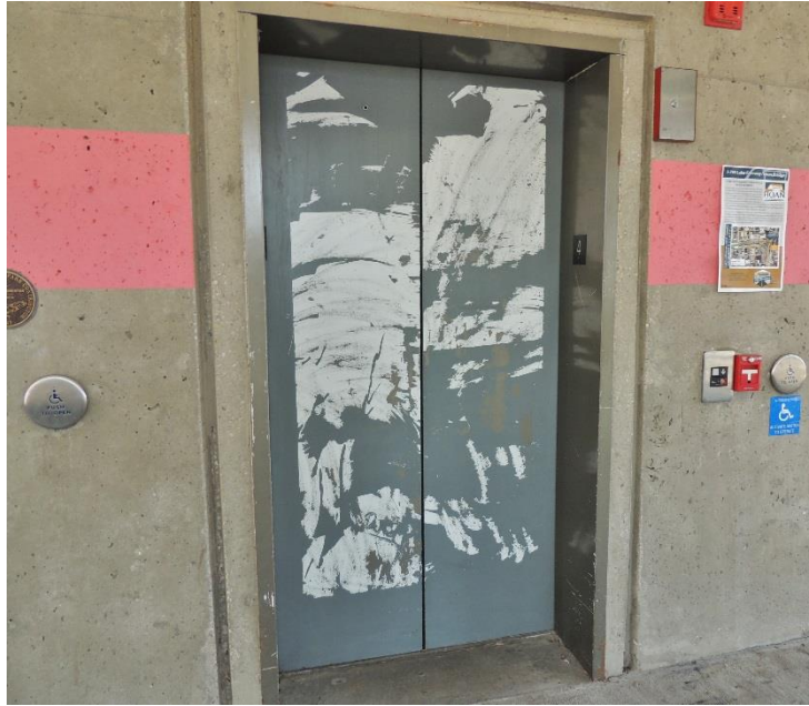
An unsightly and uninviting elevator on the property shows signs of wear.
