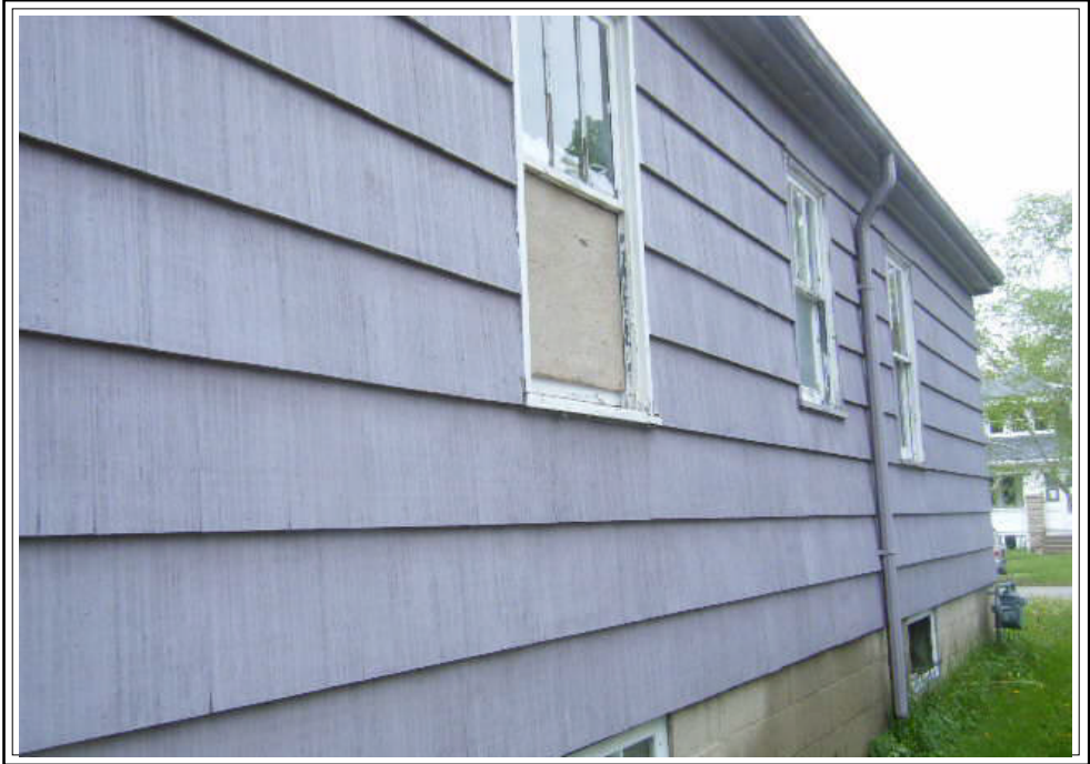
Side of house and missing windows
