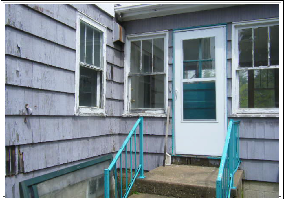
Trim paint needed and siding repair needed
