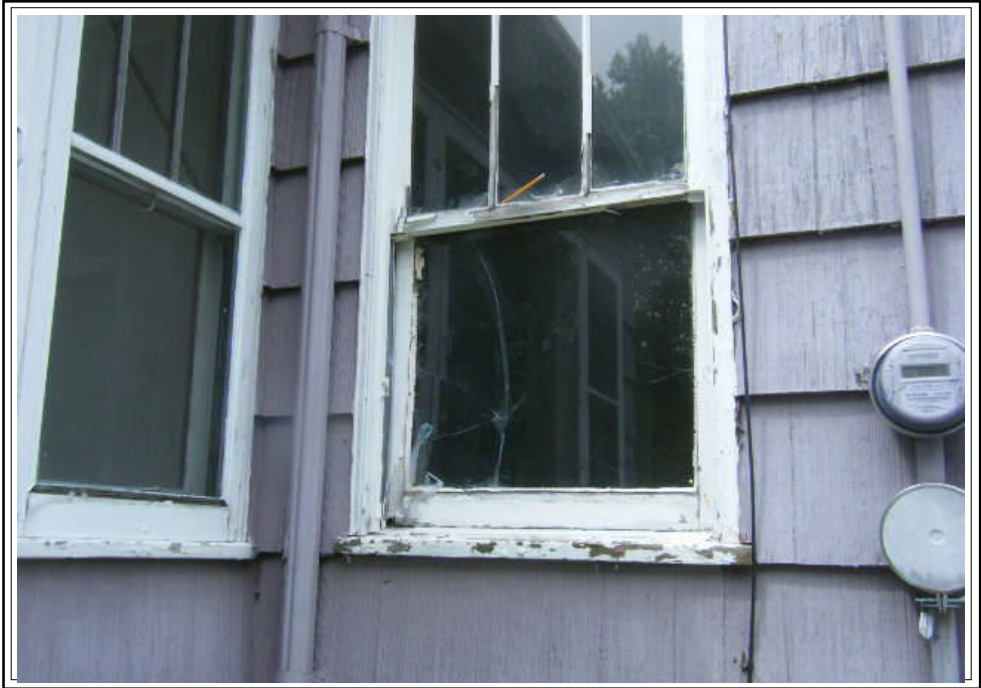
Trim Paint Needed
