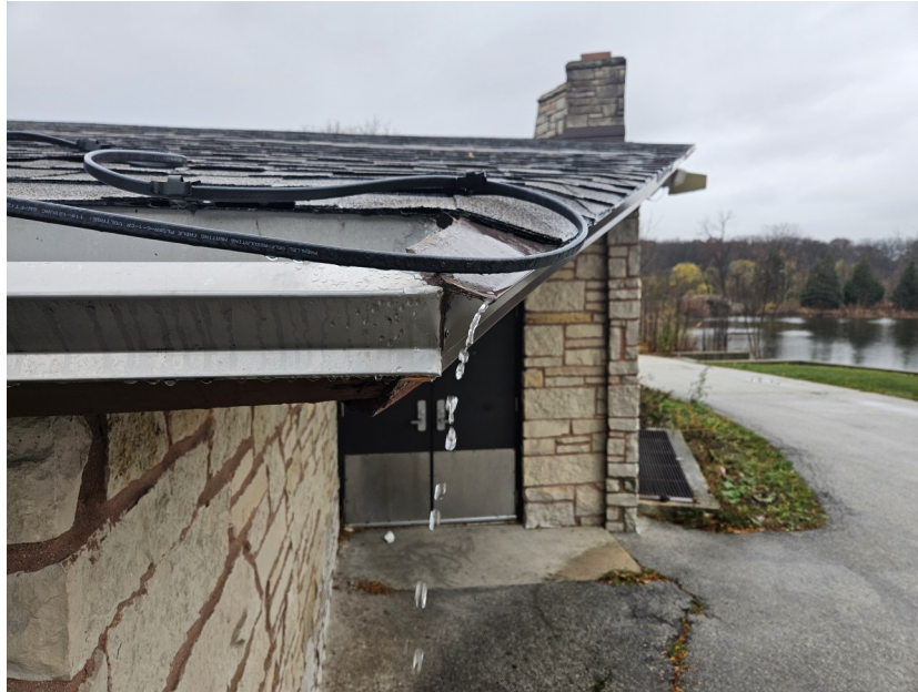
Photo 13: Needed Trim Where There is No Gutter
