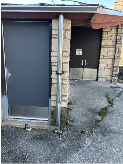
Photo 13: Deteriorating and settling asphalt on north side of building.
