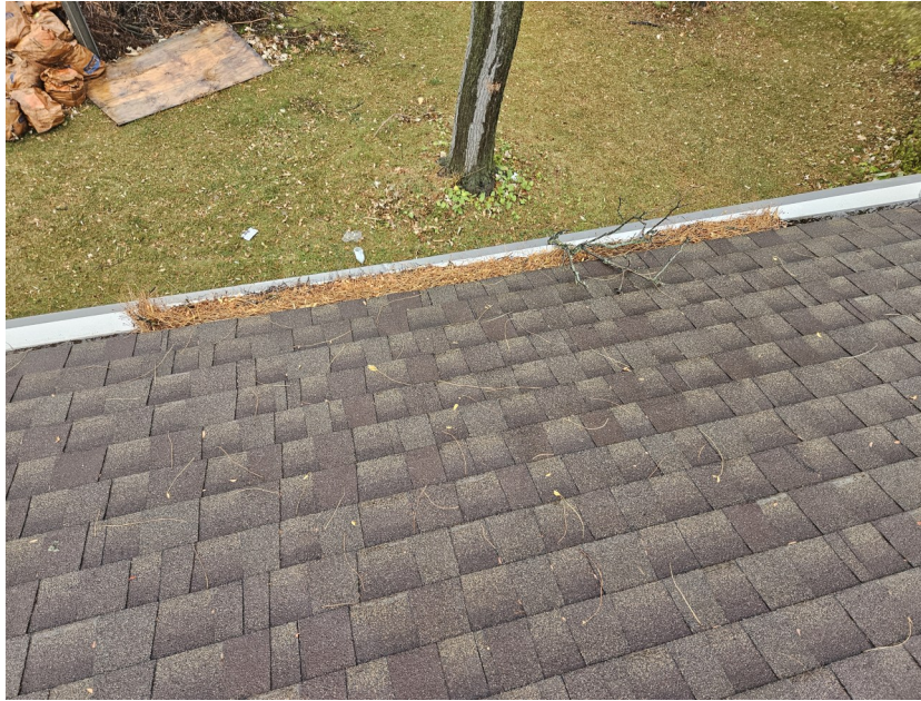
Photo 11: Blocked Gutter Inlet
