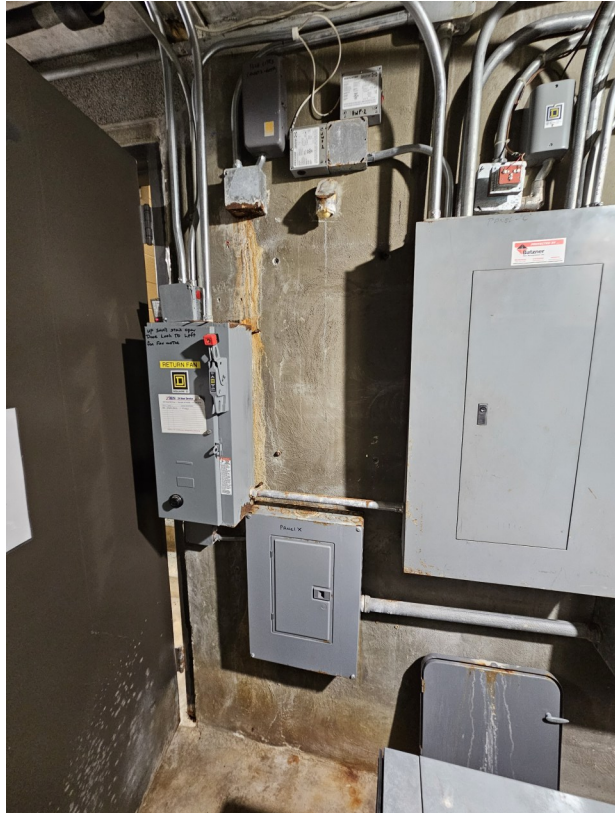
Photo 5: Foundation Wall Penetration Leaks
