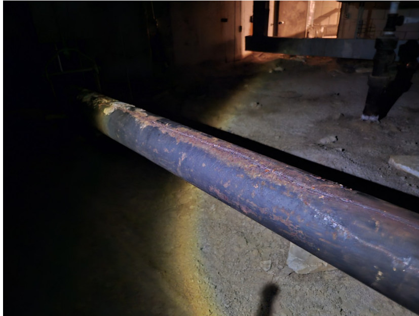
Photo 1: Damaged Storm Pipe
