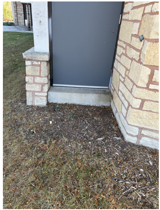
Photo 2: Unpaved area adjacent to door on west side of building.
