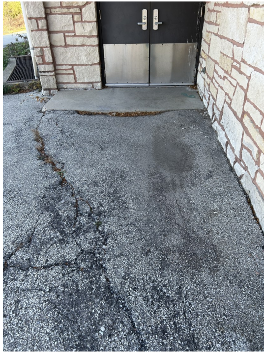
Photo 16: Deteriorating and settling asphalt on northwest side of building.
