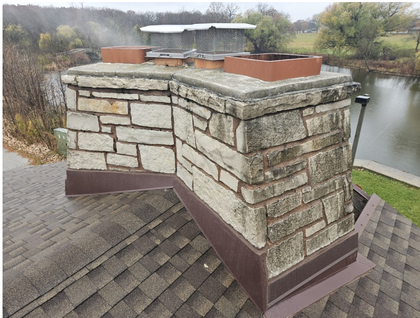
Photo 12: Missing Flue Cap
