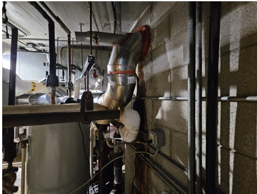
Photo 6: Boiler Exhaust Leak
