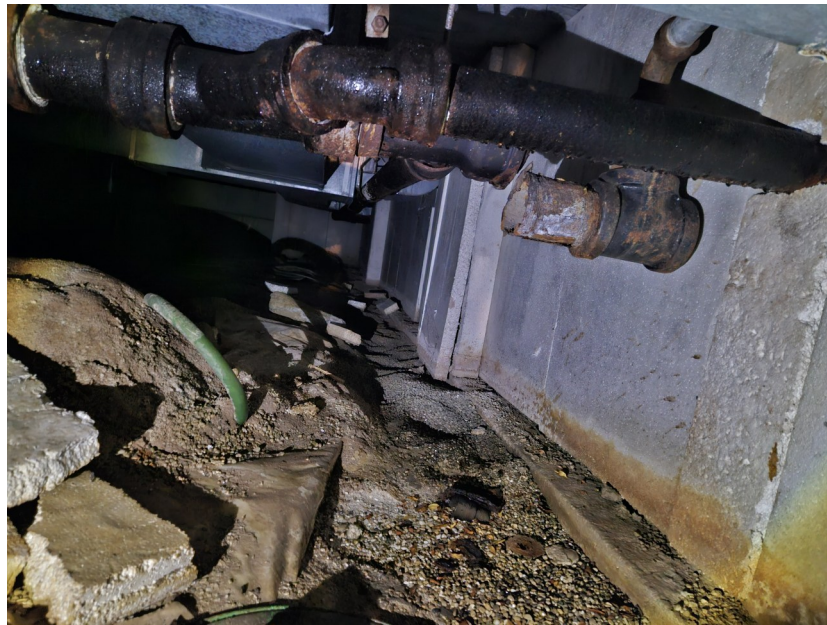
Photo 2: Broken Sprinkler Pipe
