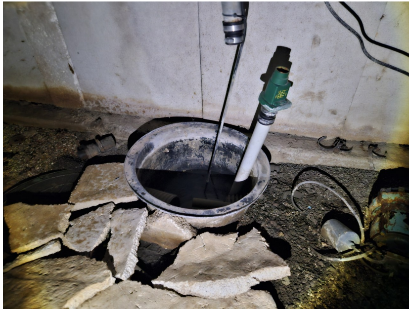
Photo 3: Disconnected Sump Pump
