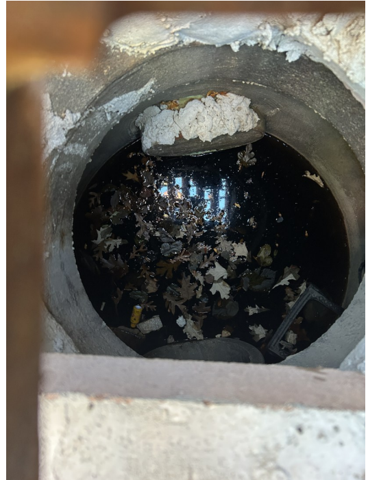
Photo 10: Inlet in parking lot with concrete filled pipe connection.
