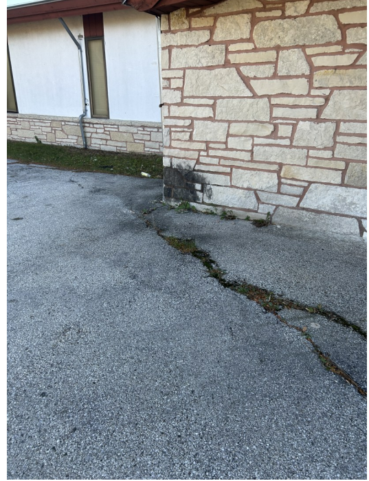
Photo 14: Cracked and settling asphalt on north side of building.
