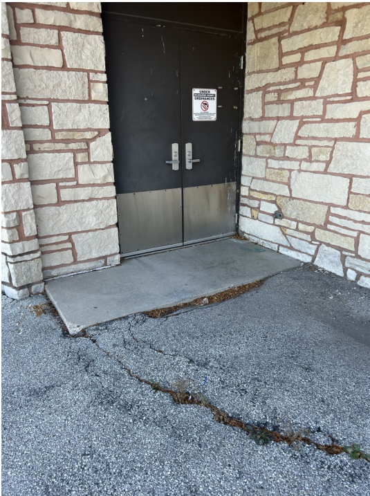
Photo 15: Settling asphalt near entrance on northwest side of building.
