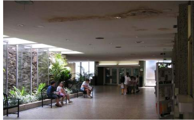
Commons with Water Damage
