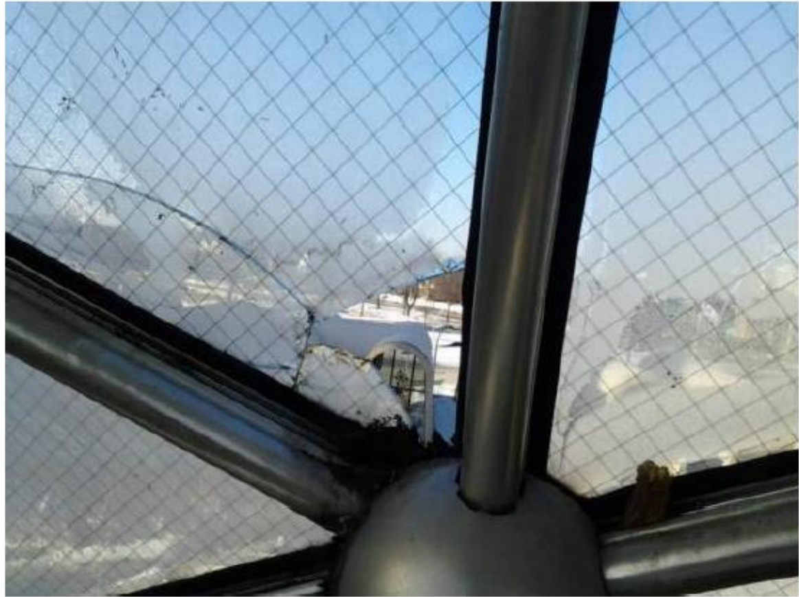
Photo F11: BROKEN GLASS LETS IN AIR AND MOISTURE.
