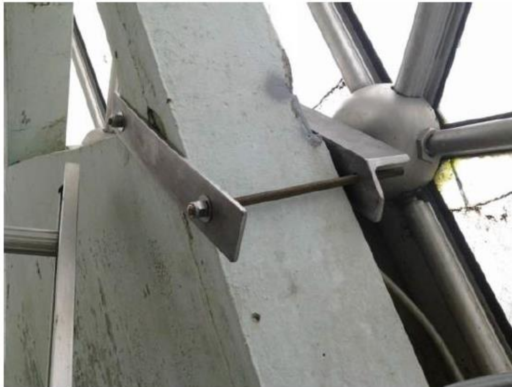
Photo F04: STAINLESS STEEL CLAMPS PULL MISALIGNED CONNECTIONS TIGHT TO SUPPORTING REINFORCED CONCRETE STRUCTURE.
