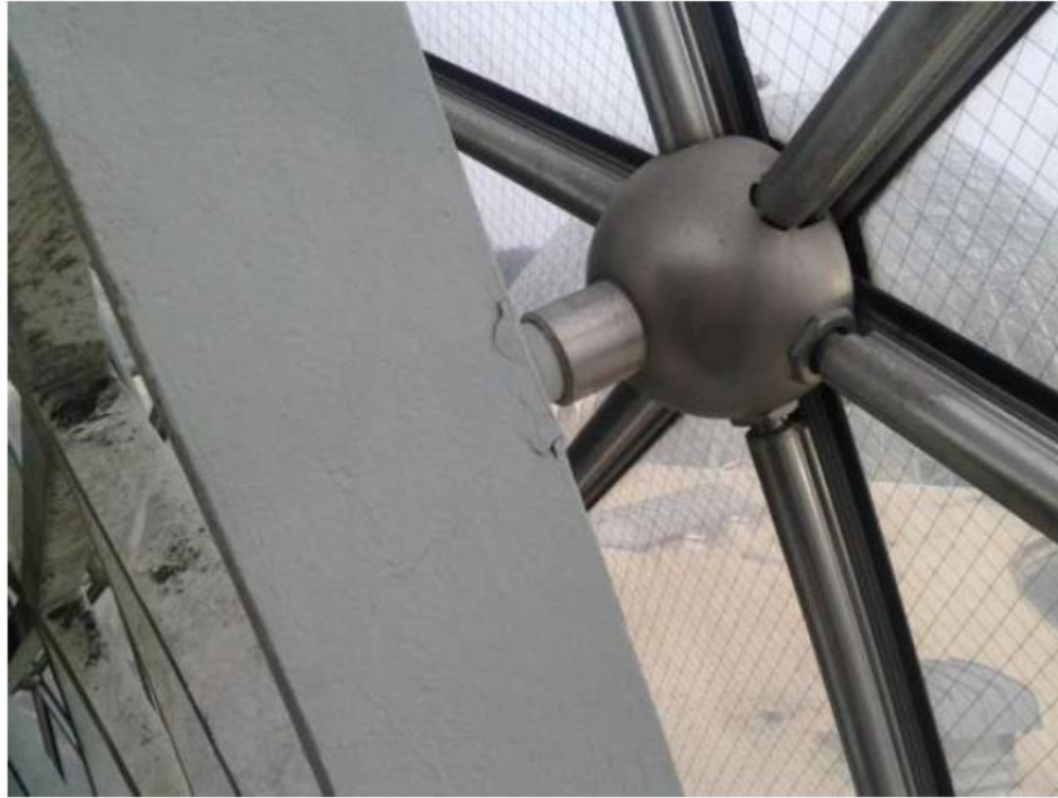
Photo F01: VISIBLE CONCRETE CRACKING AT CONNECTION OF GLAZING STANDOFF PIPE TO STRUCTURAL SPACE FRAME.
