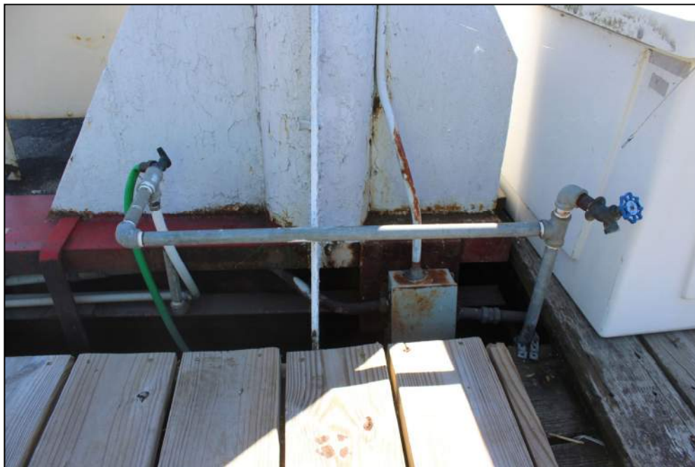
Photo 14 – Electrical box located near waterline on east channel wall.
