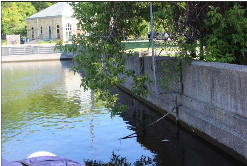
Photo 12 – View of the most northern portion of the east channel wall with concrete pile cap and rail, facing north.
