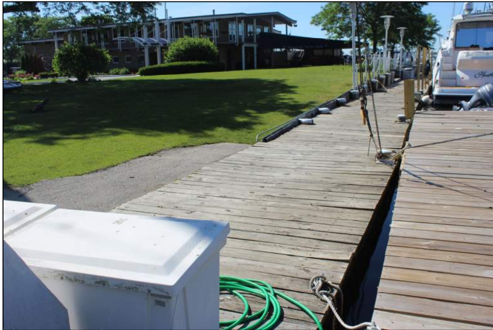
Photo 17 – View of the southern most portion of the east channel wall, facing south. Note the timber pile supported boardwalk along the length.
