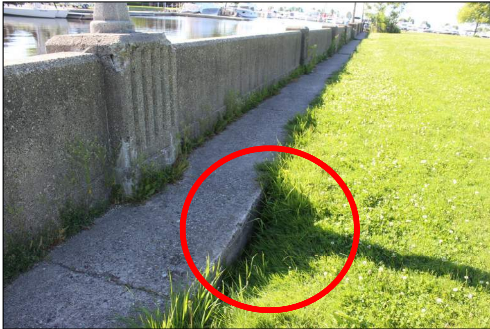
Photo 3 – Area of subsidence located along the topside of the west wall.
