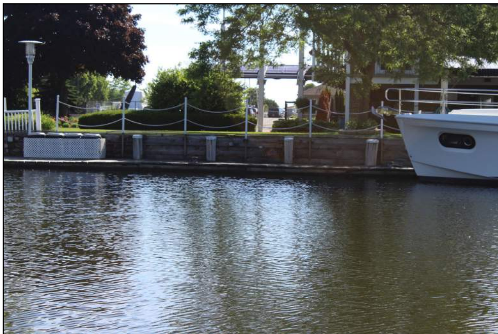
Photo 16 – View of the east channel wall facing east. Note the high water level compared to the timber pile supported pier and small retaining structure.
