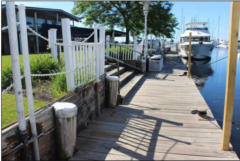
Photo 19 – View of the southern most portion of the east channel wall, facing south. Note the small retaining structure and patio area.
