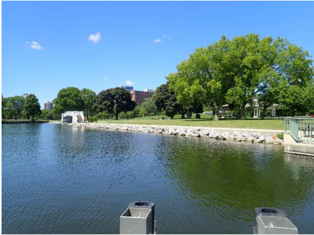
Photograph 1: Typ. condition riprap revetment with concrete wall, west of Flushing Channel (Wall Section 1), looking west.
