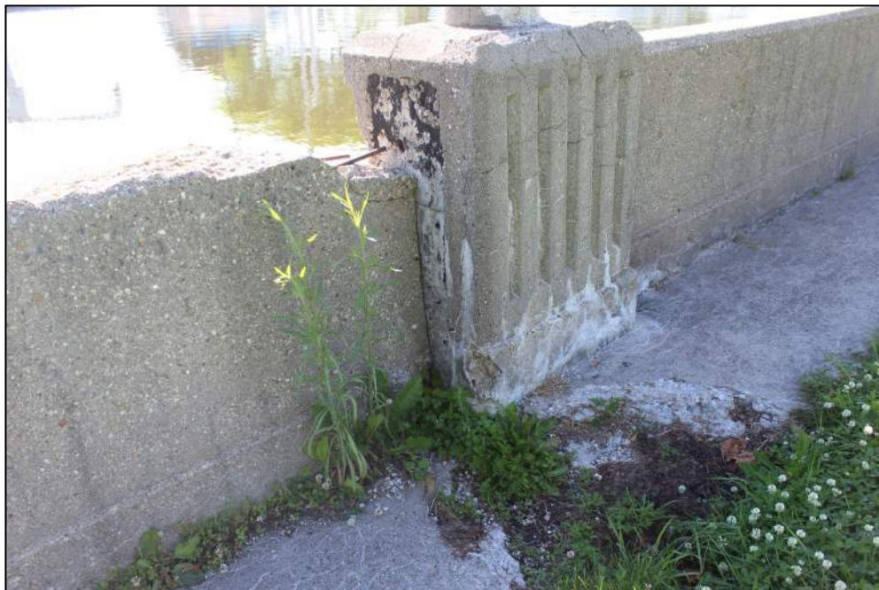
Photo 4 – Deteriorated concrete rail system along west channel wall.
