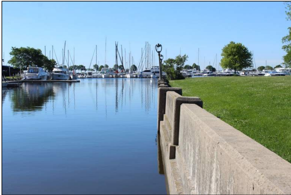
Photo 1 – View of the west channel wall facing south. Note the differential settlement of the concrete pile cap.
