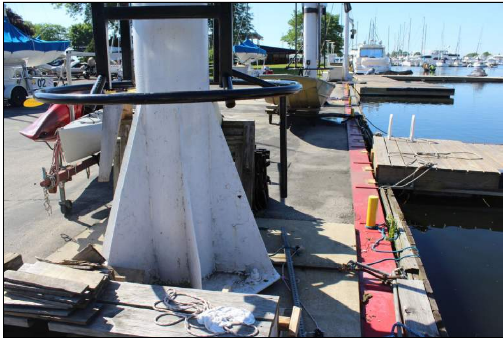
Photo 13 – View of middle section of east channel wall consisting of steel sheet pile. Note the davits located on the topside of the wall.
