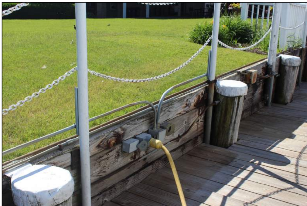
Photo 18 – Electrical outlet located near the water line along the east channel wall.
