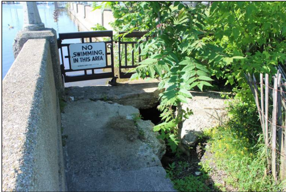
Photo 5 – Area of subsidence with unsupported concrete and exposed rebar near existing boat ramp along west channel wall.
