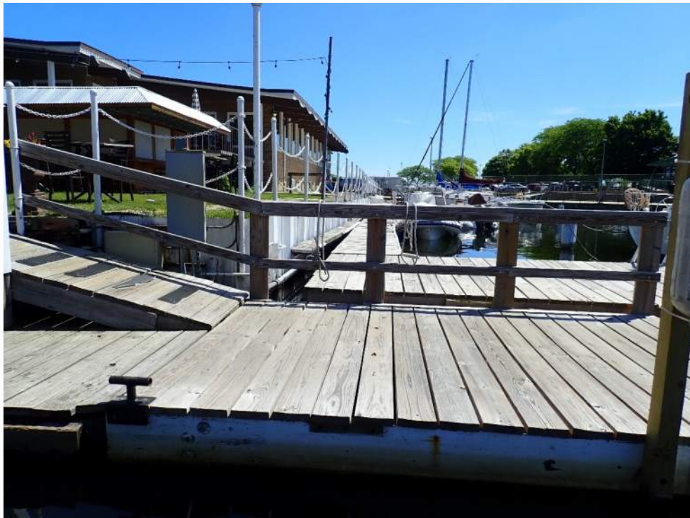
Photograph 8: View of wall located to east of flushing channel (Wall Section 7), looking northeast.
