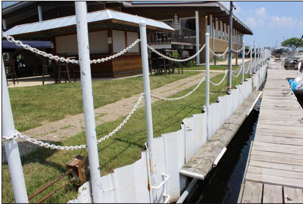
Photo 21 – Existing steel sheet pile wall that abuts the channel to the east.
