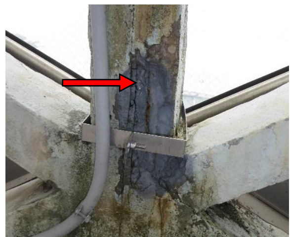
Figure 17. Removed spall within the body of the precast element. Note missing grout between precast members.
