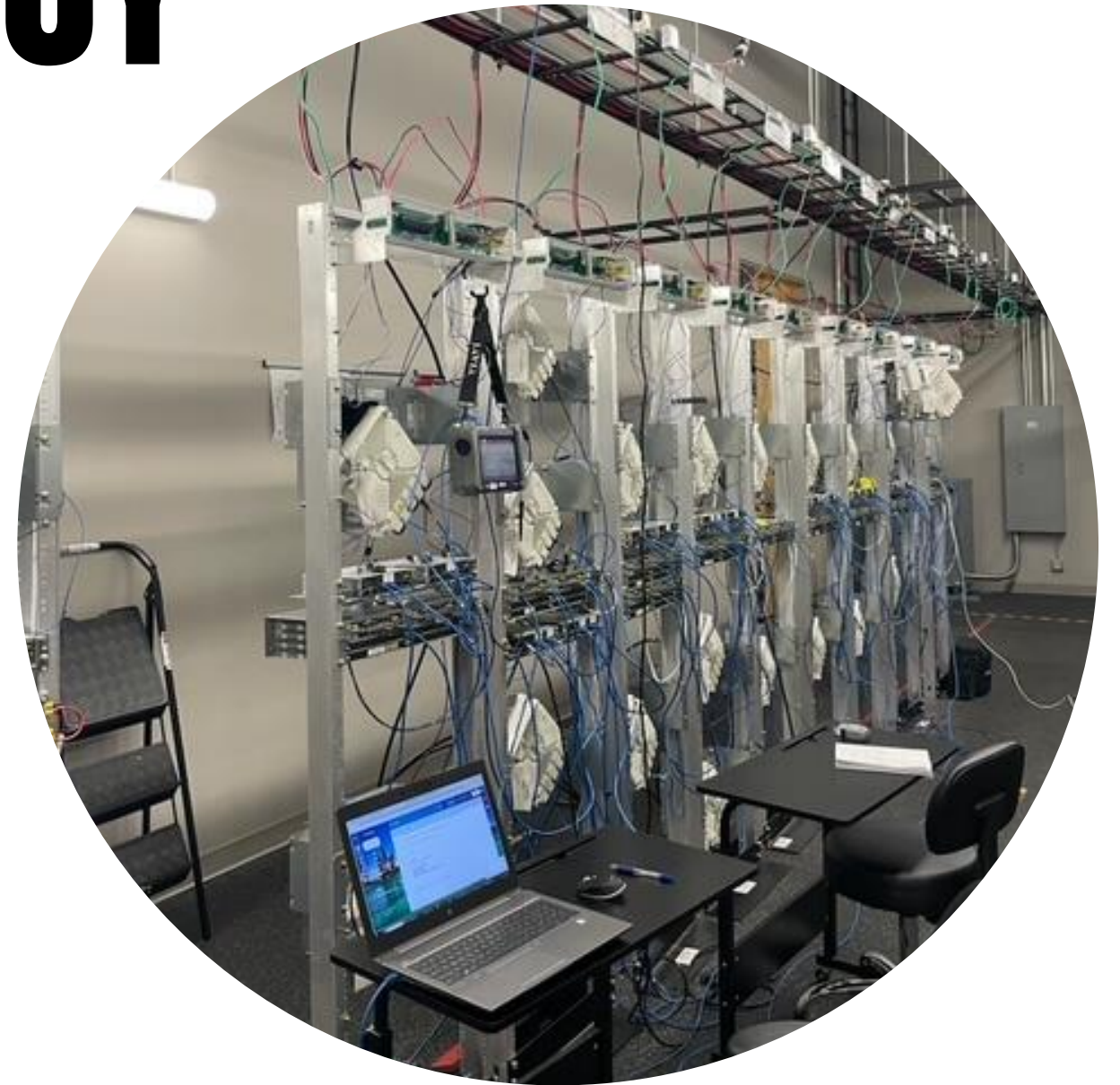
Microwave Fixed Access Transportable (FATP) units stage at Infinity's facility in Mooresville, North Carolina.
