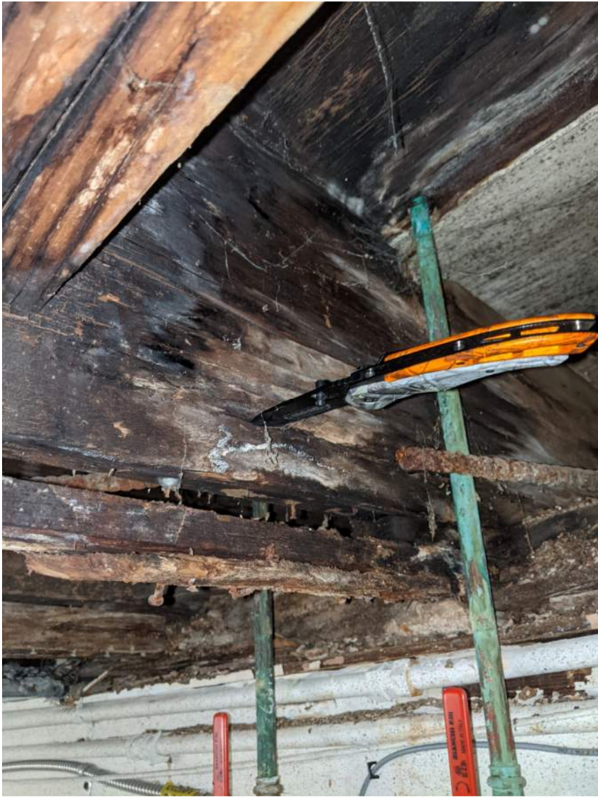
Photograph 8: Joist with Signs of Rotting
