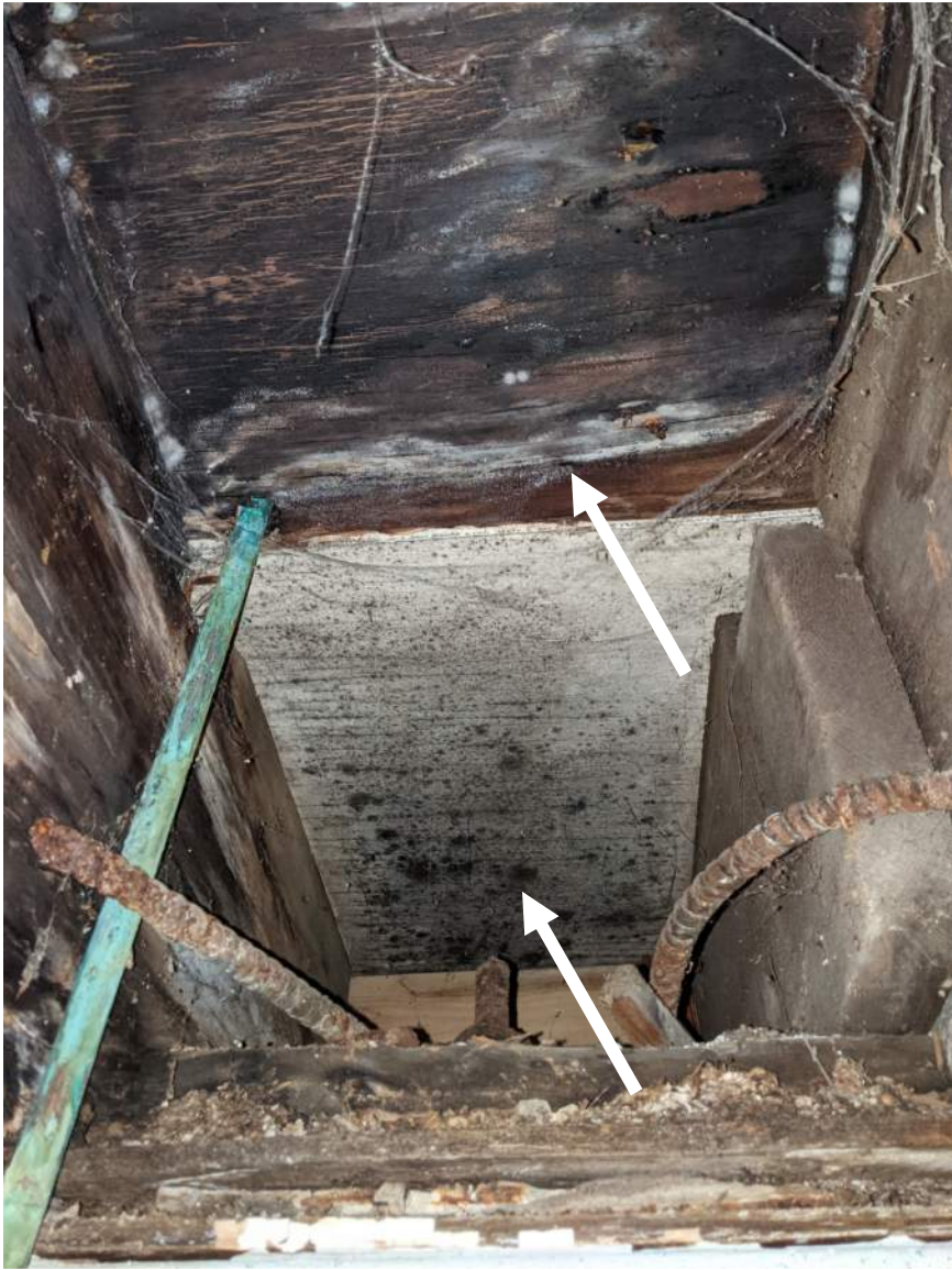
Photograph 7: Mold on Sheathing
