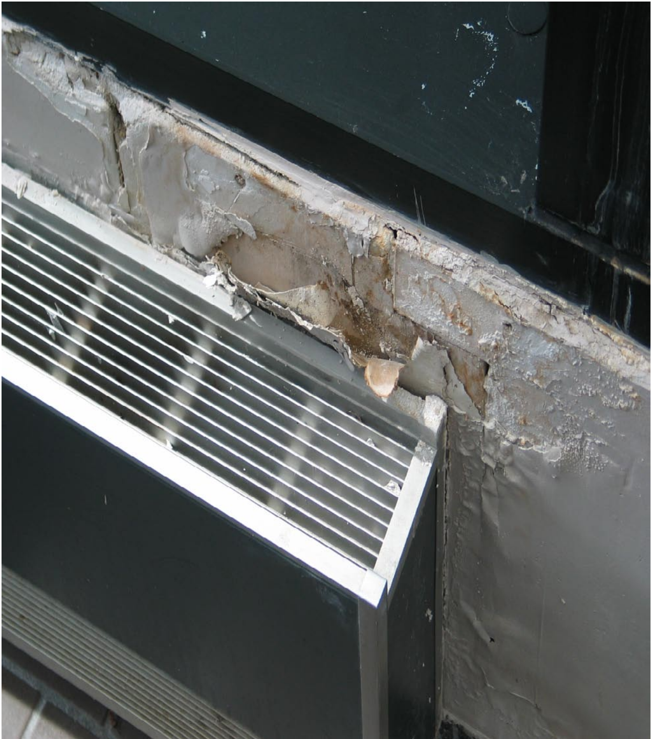
The main hall is experiencing water leakage from window due to weather stripping and sealing problems.
