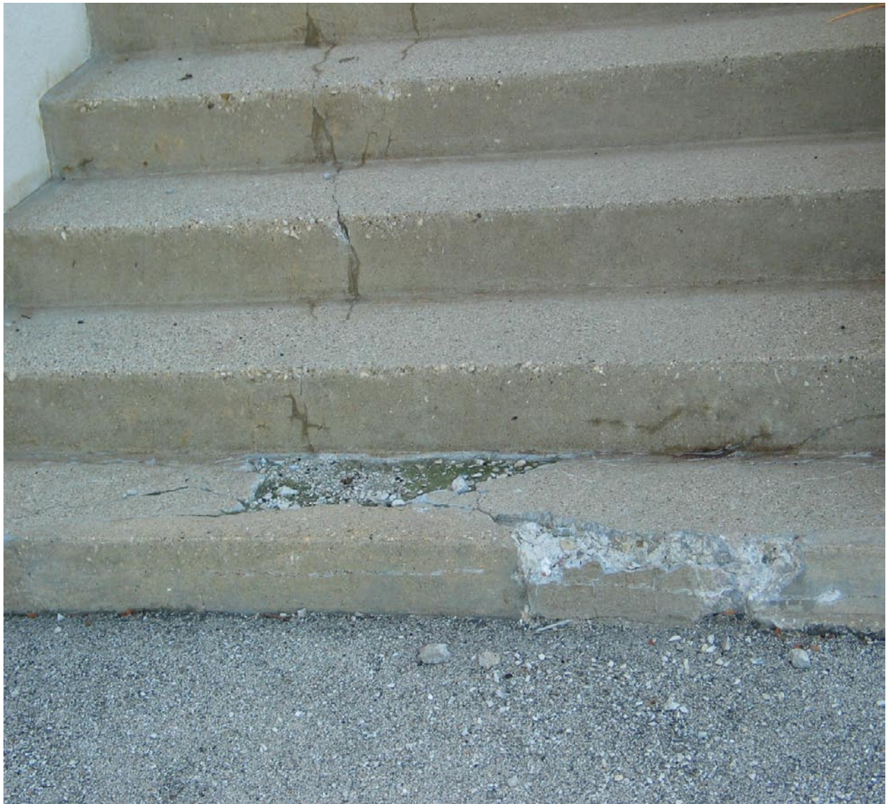
The outside staircases are in poor condition at Parks Administration Building the rear exit staircase show evidence of decaying.
