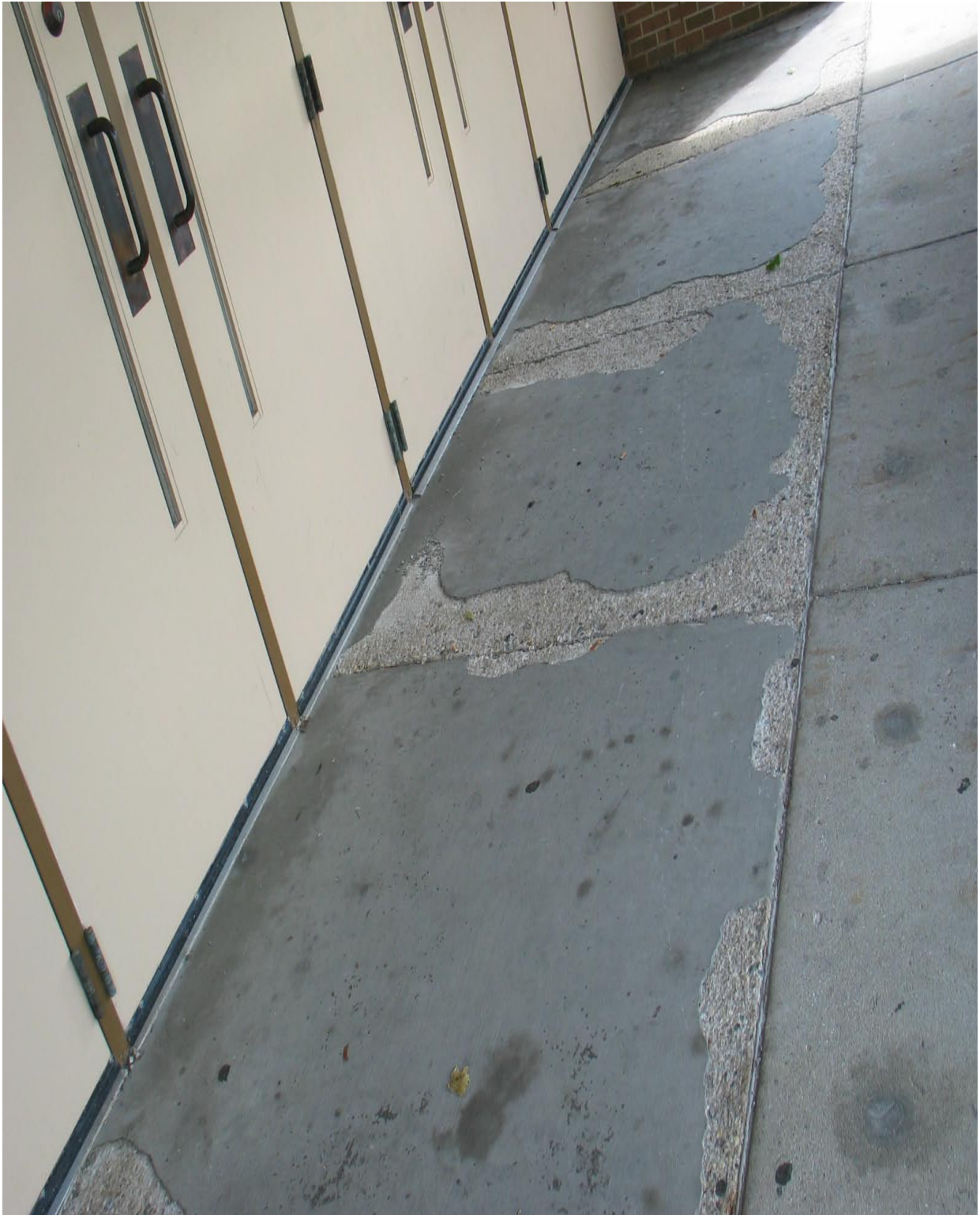
Broken concrete floor slabs at the main entrance create a potential tripping hazard.
