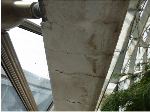
Figure 18. Transverse cracks on precast member
