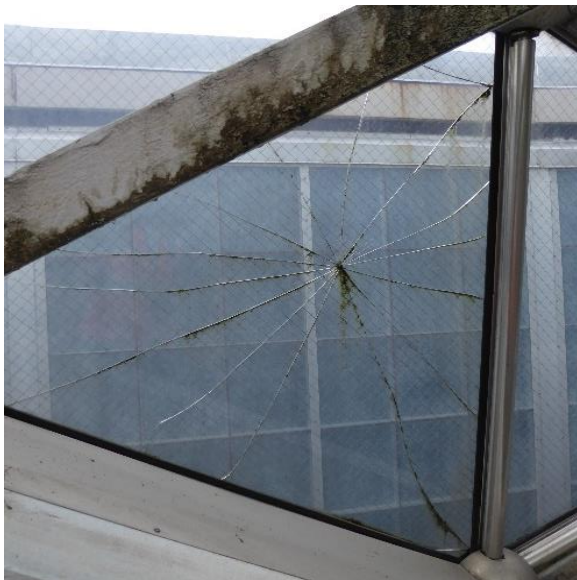
Figure 20. Cracked glass, likely from impact
