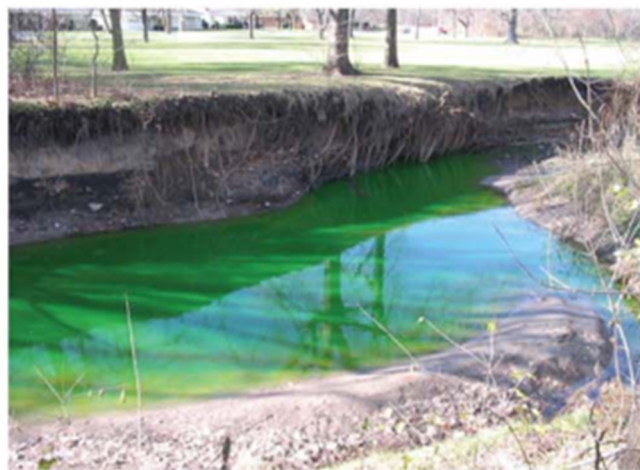
Figure 1-10. Failing Streambank (Source: SEWRPC Technical Report No. 39)
