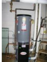
Domestic water heater
