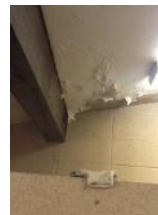
Paint peeling off the ceiling in stairwell/janitors closet area
