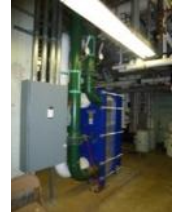
Condenser water economizer
