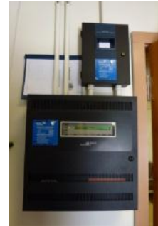
Existing fire alarm control panel
