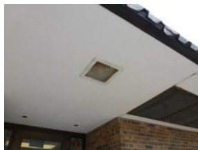
Exterior Lighting Fixture
