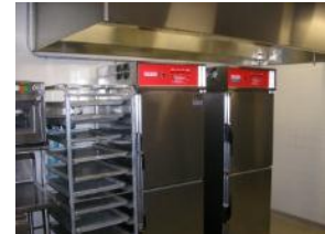
Kitchen exhaust hood
