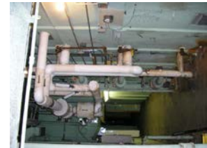
Built-up air handling unit (heating/cooling coil section)
