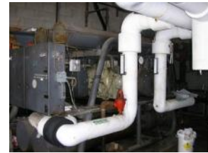
Indoor chiller (original to building)
