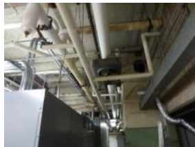
Main Switchgear with Steam Piping Overhead
