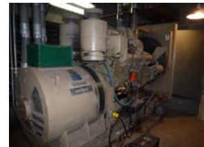
350 kW Emergency Generator
