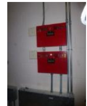
Fire Alarm Panel
