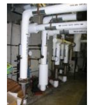
Chilled/condenser water piping & pumps
