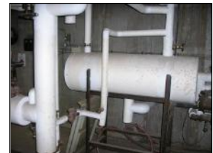
Steam to hot water heat exchanger
