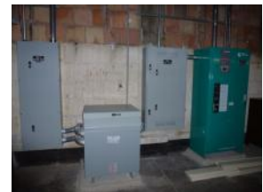
ATS for Emergency Generator
