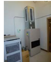
Data room air conditioning unit
