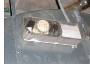
Duct smoke detector
