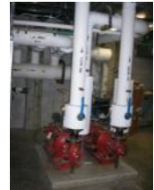
Hot water pumps
