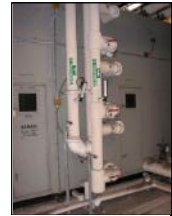
Air handling unit chilled water coil
