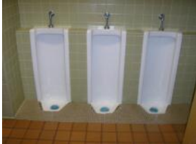
Floor mounted urinals
