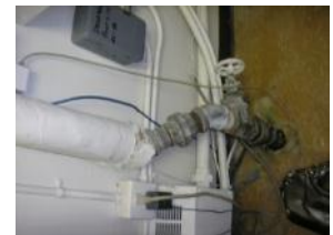
Piping insulation is damaged
