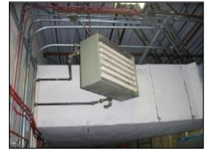
Hot water suspended unit heater (mechanical room)
