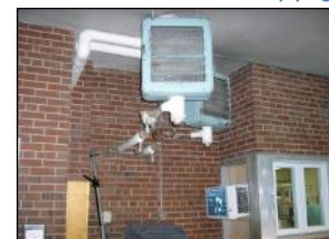
Suspended steam unit heaters
