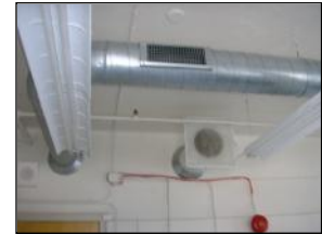
Lab supply register and exhaust grille
