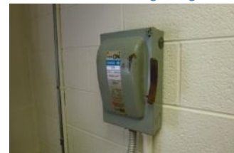
Disconnect Switch for Kiln
