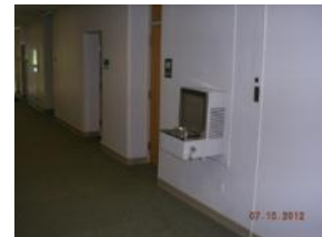
Drinking fountains non-ADA compliant – projecting hazard
