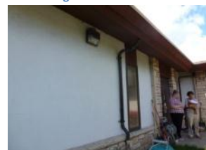
Existing Exterior Light Fixture
