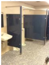
Typical restroom, stall not fully HC accessible
