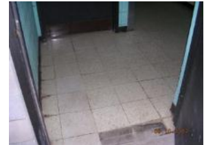
Water damage to basement floor
