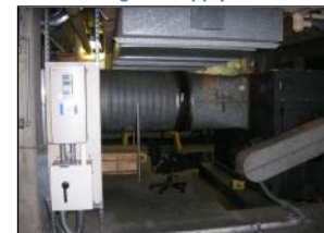
Air handling unit and variable frequency drive
