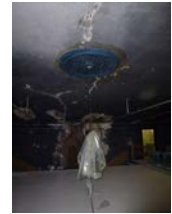
Wiring Remaining from Chandelier
