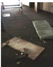
Broken ceiling tile, debris on the floor
