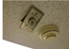
Heat Trace Connection and Existing Smoke Detector
