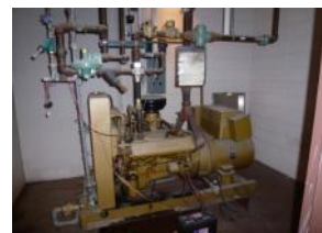
60kW Emergency Generator
