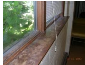
Typical wood window in poor condition
