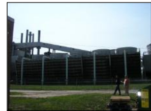
District power plant
