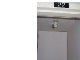
Existing Porcelain Fixture with Compact Fluorescent Lamp
