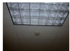
Recessed Fluorescent Fixture and Fire Alarm Strobe and Speaker
