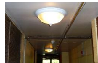
Incandescent Light Fixtures and Existing Telephone Cabling
