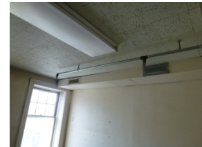
Downright sprinkler heads
