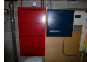
Fire Alarm Control Panel
