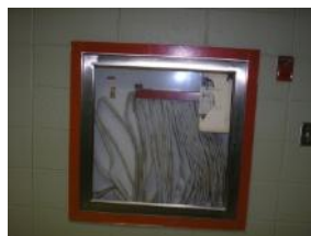
Fire hose cabinet
