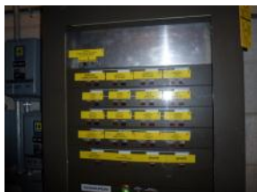
Fire Alarm Annunciator Panel
