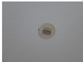
Fire Alarm Strobe and Speaker
