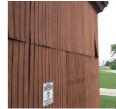
Wood siding warped, pulling away from building
