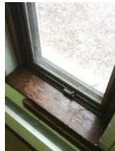
Typical window, hardware broken
