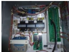
Prison Control Cabinet
