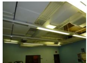
Workout Room Lighting
