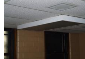
Surface Mounted Fluorescent Lights
