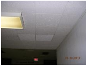
Some ceiling tiles in poor condition, replaced tiles do not match the original
