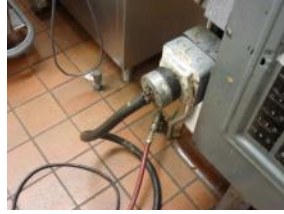
Equipment Receptacle and Panel
