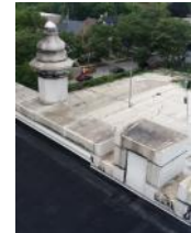
Parapet stone needs cleaning
