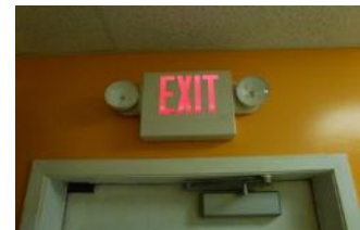
Exit Sign/Emergency Light with Battery Backup
