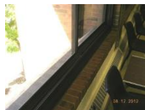
Typical storefront window, two operable single pane glass panels. Brick sills in good condition
