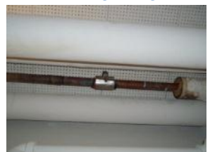
Pipe clamp on existing piping, which indicates there was a leak here
