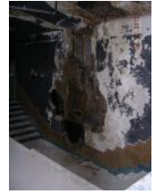
Main stairway in theater lobby. The lack of maintenance and repair has left the theater in poor condition
