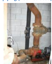
Cooling tower condenser water pump
