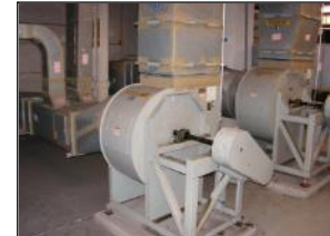
Centrifugal exhaust fans
