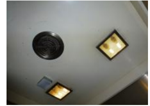
Recessed Light Fixtures
