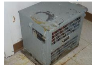
Transformer, Recommend replacement
