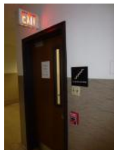
Fire Alarm Pull Station and Exit Sign
