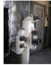
Built-up AHU heating/cooling coil sections
