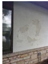
Exterior wall patched, paint peeling in some areas
