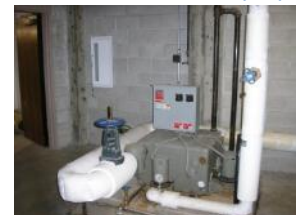
Condensate return pump
