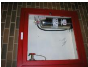
Fire extinguisher cabinet
