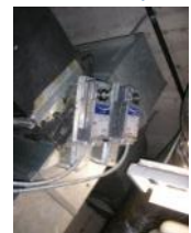
Control damper electric actuators
