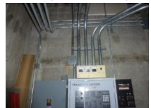
Emergency Control Panel and Transfer Switch
