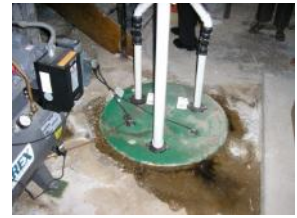
Sump pump (replaced April 1996)
