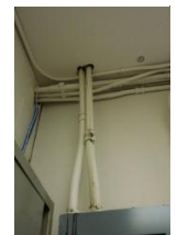
Wall and ceiling pipe penetrations not sealed
