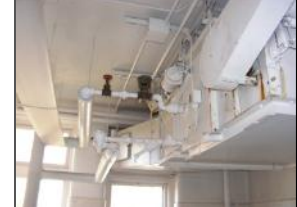
100% O.A. air handling unit
