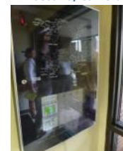
Fire Alarm Annunciator Panel
