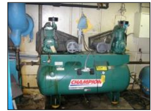
Temperature controls air compressor
