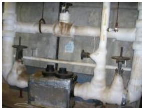
6" water meter on concrete base
