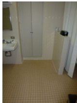
Missing floor drain
