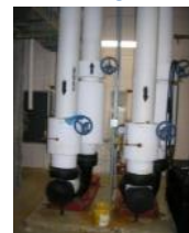
Chilled water pumps
