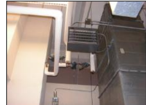
Steam suspended unit heater
