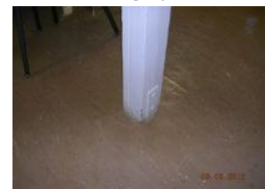
Columns in main space worn
