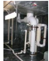
Built-up air handling unit
