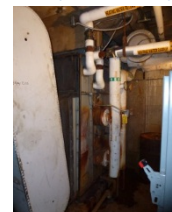
AHU heating coil section (basement)
