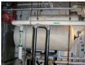
Domestic hot water heater with storage tank
