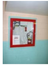
Fire extinguisher cabinet
