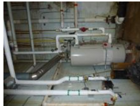
Domestic hot water heater
