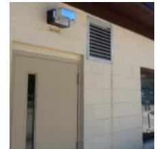
New caulking needed in expansion joints
