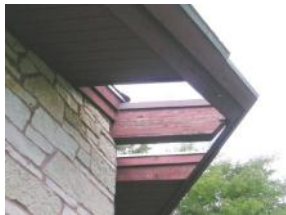
Roof overhang wood worn, weathered. Some caulking is needed at joint to wall
