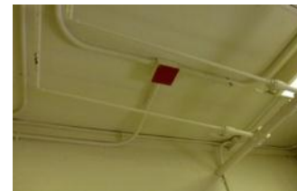
Fire alarm conduits not painted red
