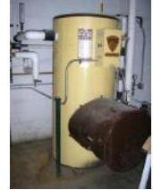
Domestic water heater
