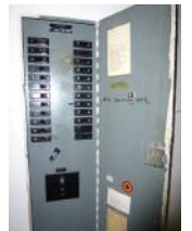
Branch Circuit Panel
