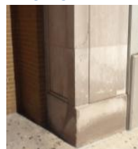
Stone deteriorating, tuck pointing needed on brick work in some spots
