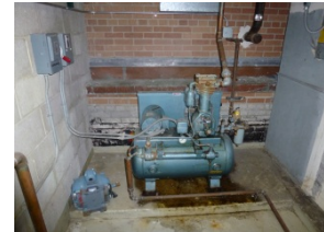
Temperature controls air compressor
