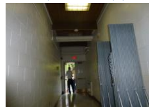
Exit Sign and Smoke Detector
