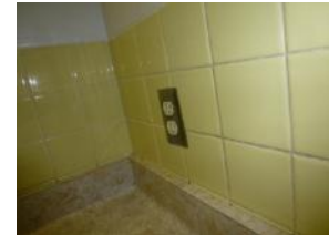
Bathroom Receptacle not GFCI
