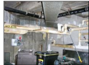
Steam, condensate, and hot water piping
