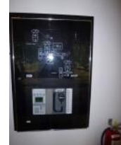
Fire Alarm Annunciator Panel
