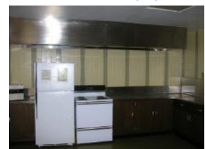
Oversized kitchen exhaust hood
