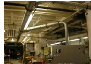
Dust collecting system
