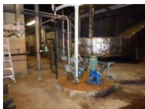
Two sump pumps
