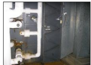
Air handling unit filter section
