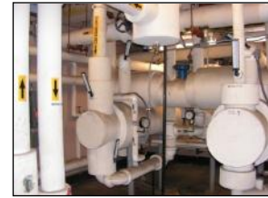
Steam to hot water heat exchangers
