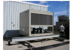
Air cooled condensing unit
