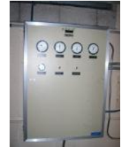
Pneumatic temperature control panel
