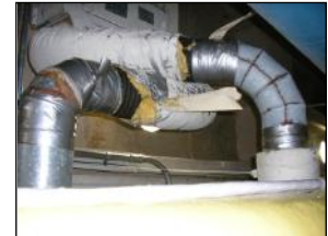
Reheat box inlet ductwork
