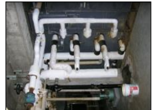
Air handling unit heating/cooling coils
