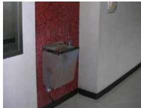
Drinking fountain non-ADA compliant
