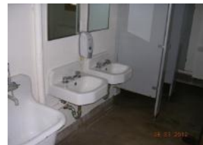
Craft hall restrooms in poor condition (women's closed), non-ADA compliant
