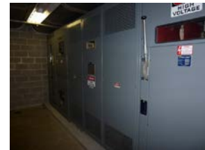
Substation USS/3 Installed 1991
