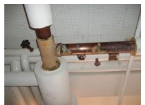
Insulation removed from sprinkler pipings maller pipe has pipe clamp
