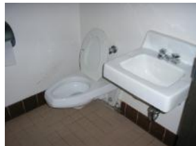
Wall - hung lavatory and sink
