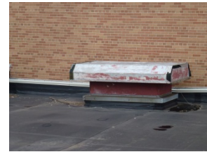
Outdoor air intake hood
