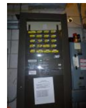
Fire Alarm Panel
