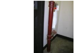
Standpipe riser with fire hose
