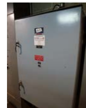
Emergency Transfer Switch ATS/2
