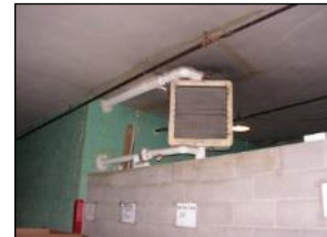
Suspended steam unit heater
