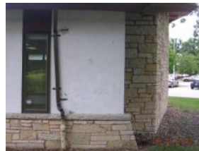
Downspouts in poor condition
