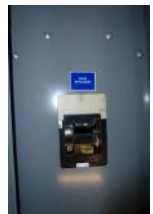
Main Service Breaker
