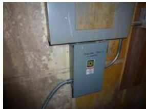
Rusted Panel BF/G
