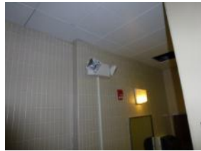
Battery Backup Emergency Light Fixture
