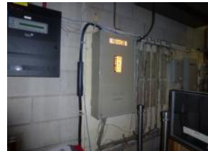
Fire Alarm Panel and Incoming Telephone Service Equipment
