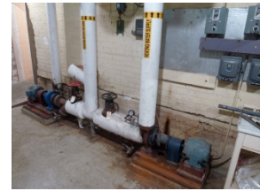
HW pumps (5th floor penthouse)
