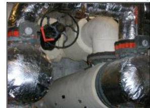
Steam to hot water heat exchangers
