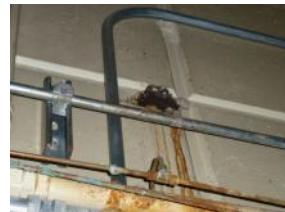
Rusted Conduits and Area of Leakage
