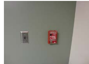
Fire Alarm Key Operated Pull Station
