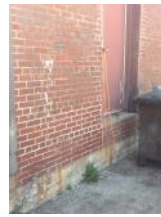
Brick work in fair condition, tuck pointing needed in some areas
