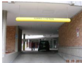
Driveway to main entrance, no separate handicap ramp or railings
