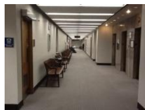
Carpet in the 7th and 8th floor corridors is worn, stained
