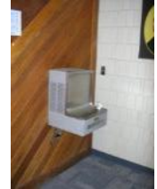
Electric water cooler
