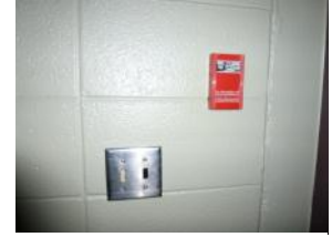
Fire Alarm Pull Station
