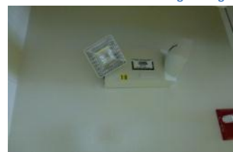
Emergency lighting battery pack
