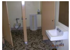
Restroom, not fully accessible
