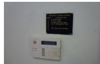
Existing Security Alarm Panel
