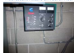
Generator Battery Float Charger
