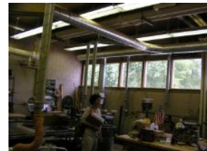
Dust collection system (woodworking shop)
