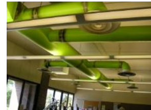
Unit ventilator supply ductwork
