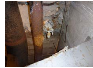
Corroded Conduit Above Piping in Basement Boiler Room
