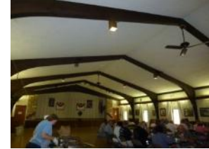
Existing Main Dining Hall Lighting
