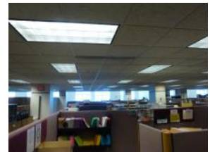
Light Fixtures with T-8 Lamps
