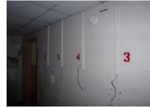
Smoke Detector and Disconnected Wires
