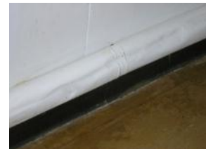
Piping insulation is damaged
