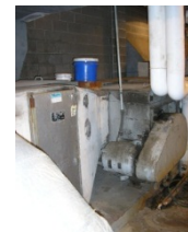
AHU supply fan section (9th floor penth.)
