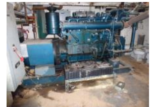
Inoperative Emergency Generator
