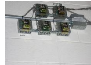
VVT system control transformers
