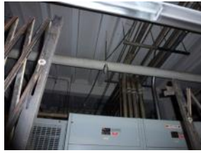
Steam Piping Over Electrical Gear
