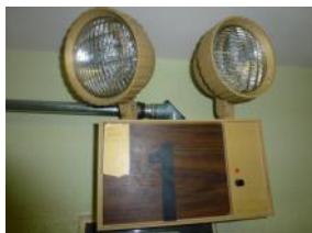
Emergency Battery Pack Light Fixture from 1970's
