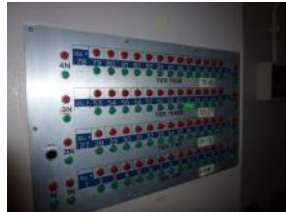
Cell Door Status Panel
