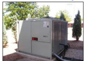
2003 air cooled condensing unit
