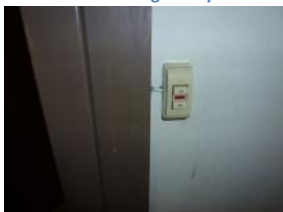
6th Floor Office Light Switch
