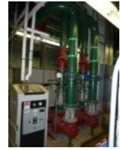
Condenser water pump
