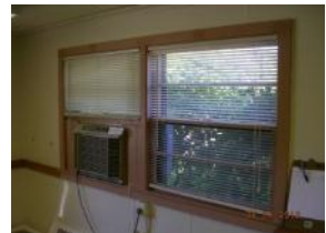
Typical window AC unit
