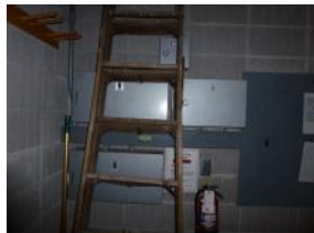
Ladder Resting Against Electrical Equipment
