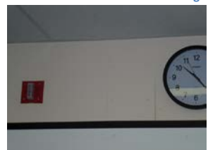
Fire Alarm Strob/Horn and Clock
