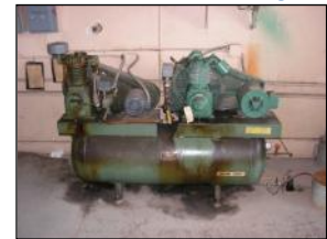
Pneumatic controls air compressor
