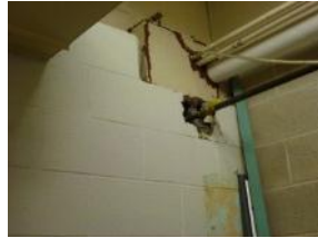
Wall damaged/sprinkler line
