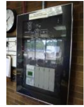
Fire Alarm Annunciator Panel
