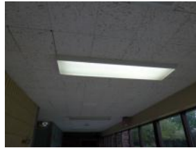
Fluorescent Light Fixture
