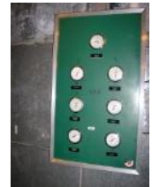
Pneumatic temperature control panel
