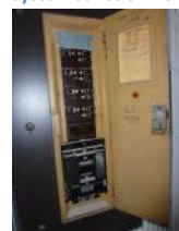
Panel LC #83A Should be Replaced
