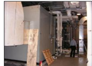
Air handling unit
