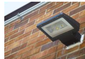
Exterior Lighting Fixture
