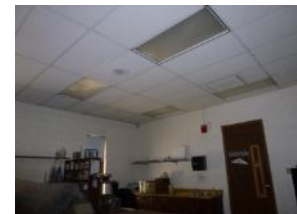
Existing Recessed Lighting and Speaker
