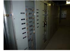
Substation USS/1 Installed in 1964
