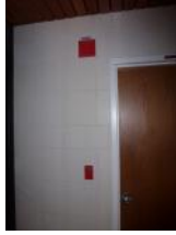
Fire Alarm Strobe, Speaker and Pull Station
