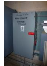
Existing main service disconnect abandoned in 2004
