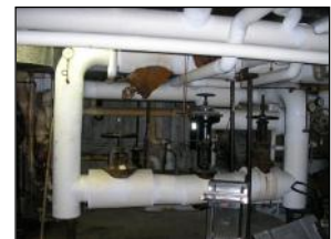
Steam piping and valving
