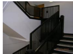
Typical stairs, with non-ADA compliant handrails
