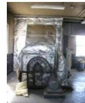
Built-up air handling unit
