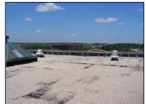
No gravity ventilators on 5th floor roof
