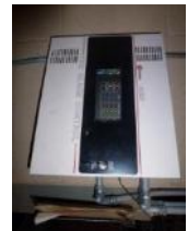
Existing Fire Alarm Control Panel
