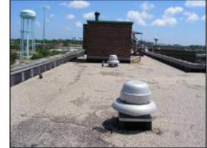
1977 power roof ventilators
