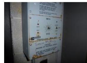
Rusted Snow Melt Panel
