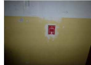
Fire Alarm Pull Station
