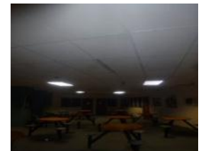
Recessed Fluorescent Lighting
