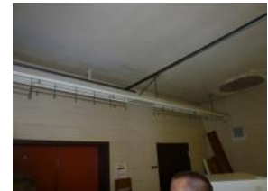
Fluorescent Light Fixture
