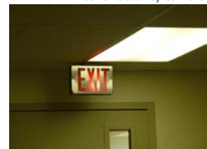
Recessed Fluorescent Light Fixture and Exit Sign
