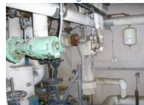
Hot water storage tank missing
