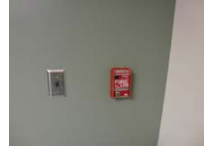
Fire Alarm Key Operated Pull Station
