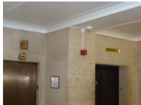
Fire Alarm Strobe and Smoke Detector in Elevator Lobby
