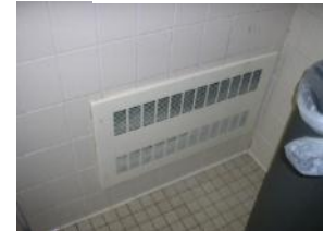
Wall hot water convactor
