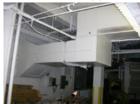
Upright sprinkler head with piping
