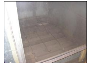
Duct mounted control damper
