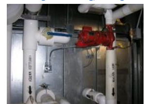
Heating coil booster pump
