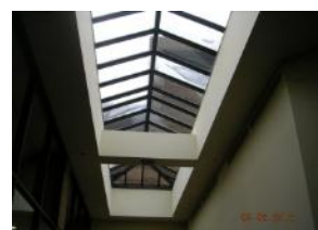
Original glass in skylight, some panes have filled with moisture
