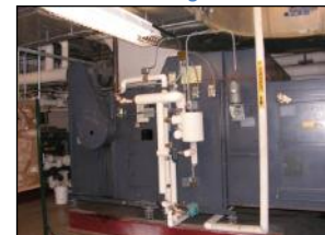
Air handling unit (mezzanine)
