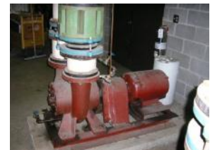
Hot water pump
