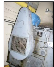
Air handling unit (supply fan section)
