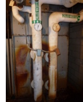
AHU cooling coil section (basement)
