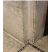
Floor and wall stone panels worn and dirty in a few high-traffic areas
