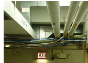
Existing ductwork and HVAC piping
