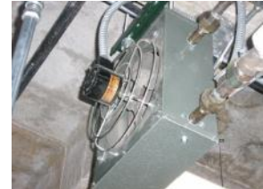
Suspended unit heater
