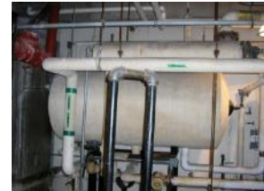
Steam to domestic hot water heater/tank
