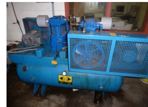
Temperature controls air compressor
