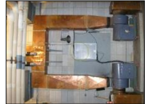
Pool exhaust fans
