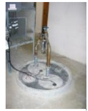
Duplex sump pump
