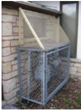
Gas meter pressure regulator & piping
