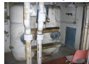
Domestic storage tanks
