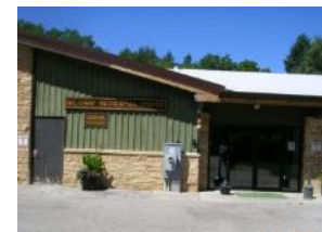
New wood fascia needs painting to match existing
