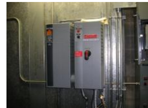
Return fan variable frequency drive
