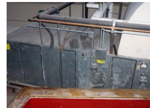
Air handling unit
