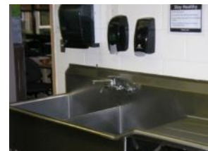
Two-compartment kitchen sink
