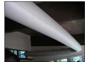
Fabric ductwork (Three-season Room)
