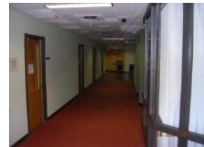
Office corridor with worn carpet and a few replaced ceiling tiles
