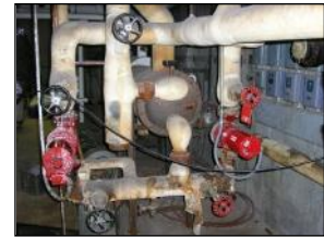
Hot water pumps
