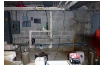
Electrical service equipment and main incoming water line and meter
