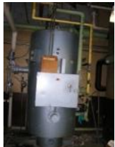
Steam to domestic hot water heat exch.
