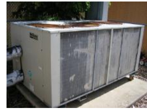
Air cooled chiller (built April 1996)
