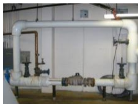
Incoming steam service
