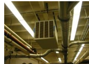
Air filtration unit
