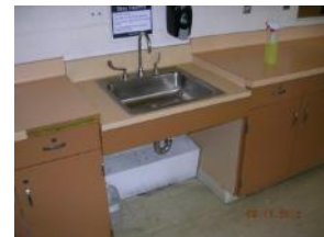
Worn casework, original floor tile in some rooms. Both at the end of their useful life
