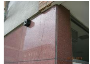
Stone panels cracked, bottom row on Wells St. sidewalk shifting from water damage, wear and tear
