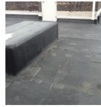
The roof membrane is patched in many spots, is not adhered everywhere. There is also damage to the roof insulation underneath
