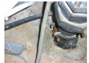
Non-compliant water fixture
