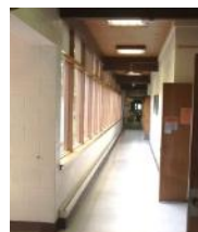
A typical corridor, doors with non-ADA compliant hardware
