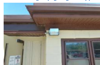
Existing exterior wall-pack lights
