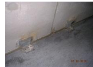
Some cracks in penthouse precast panels near shelf angles
