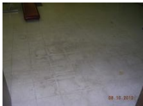
Some floors in poor condition
