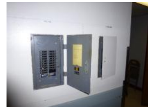
Panels PNL-1/N and PNL-1NXA
