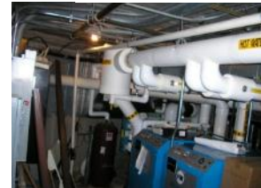
Hot water piping
