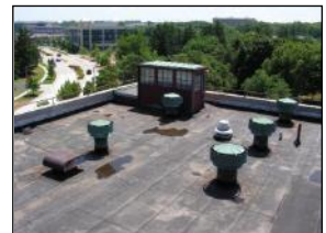
Gravity ventilators on lower roof
