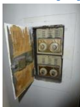
6th Floor Lighting Controls
