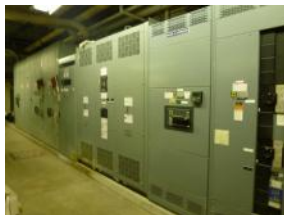
Main Switchgear Replaced in 2008
