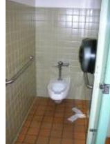
Water closet with flush valve
