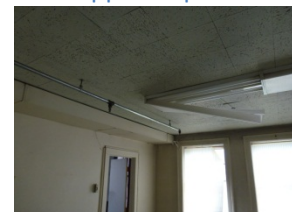
Upright sprinkler heads
