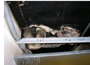
Asbestos piping insulation
