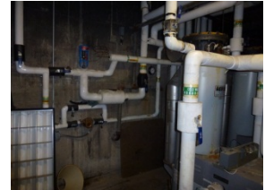
Gas-fired domestic water heater
