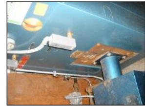
Hot water boiler
