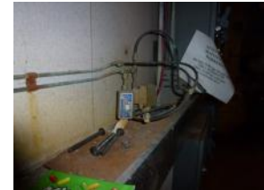
Conduits with Corrosion from Leak
