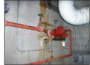
Snow melting inline pump
