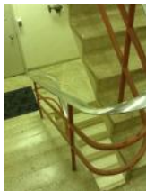
Stairwell with non-compliant railings and door hardware
