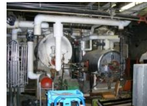
Steam to heating HW heat exchangers
