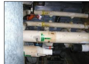
Air handling unit chilled/hot water piping
