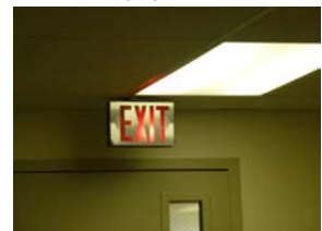
Recessed Fluorescent Light Fixture and Exit Sign
