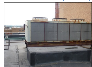
Air cooled condenser (5th floor roof)
