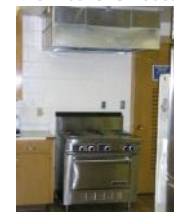
Kitchen range exhaust hood
