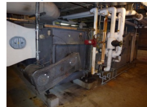
Air handling unit
