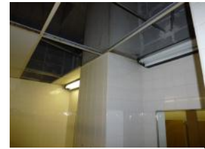
Fluorescent Lighting in Toilet Room
