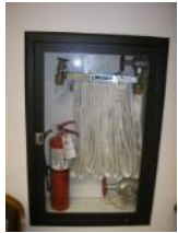
Fire hose cabinet with fire extinguisher
