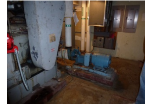
Chilled water pump (5th floor mechanical room)
