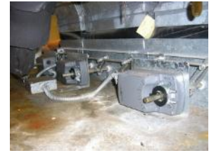
Multizone unit zone damper actuators
