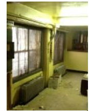
Unoccupied former jail space. Walls and windows are damaged, some space used for storage
