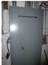
Panel LDP/SB with Improper Splicing
