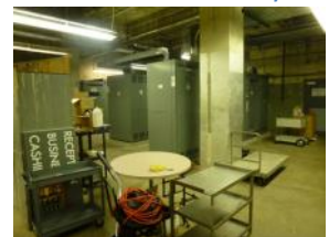
Electrical Distribution Switchboards Replaced in 2008
