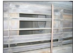
Built-up AHU supply fan section (interior)
