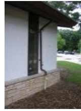
Broken vertical rain gutter
