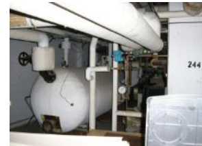
Steam to hot water heat exchanger
