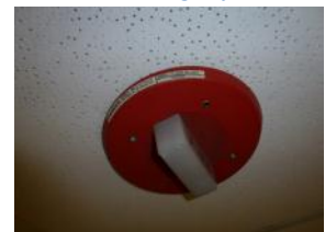
Fire Alarm Speaker and Strobe
