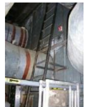
Built-up air handling unit hot/cold decks
