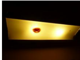
Light Fixture In Jury Room Restroom
