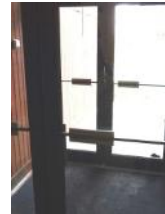
Exit doors do not have panic hardware
