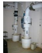
Chilled water incoming service
