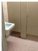
Bathrooms not HC accessible. Bathrooms, locker rooms in fair condition
