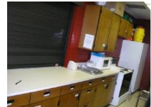
Kitchen range oven without kitchen exhaust hood
