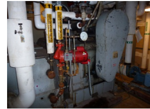
Air handling unit (5th floor mech room)
