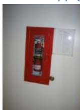
Fire extinguisher with cabinet
