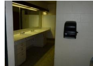
Toilet Room Lighting
