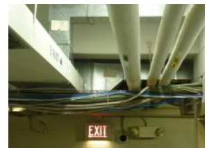
Data Cables Running Through Basement. Recommend Cable Tray System
