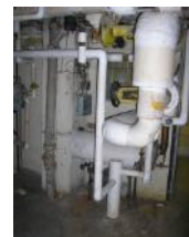
Condensate return to domestic hot water heat exchanger
