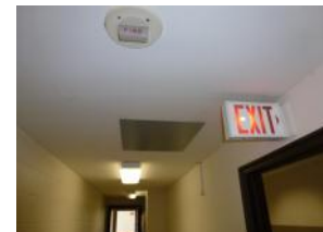
Exit Sign and Fire Alarm Speaker and Strobe
