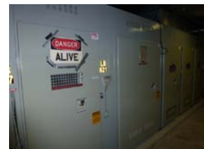
WE Energies Switchgear
