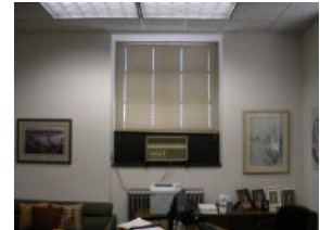
Window air conditioner
