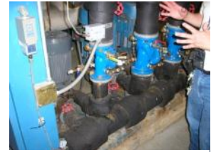
Existing water booster pump
