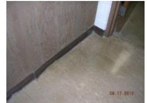
Floor and baseboard near the end of their useful life
