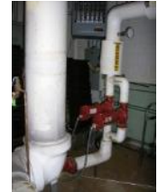
Hot water pumps
