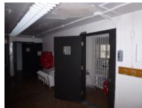
Lighting in Cell Area
