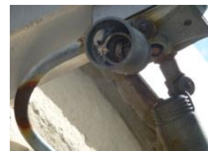
Exterior Light Fixture Empty Socket
