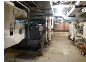
Air handling unit (5th floor penthouse)
