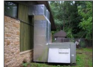
Grade mounted cooling only rooftop unit
