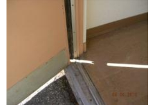
Floor slab has settled near door, creating lip at threshold
