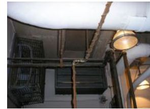
Emergency generator make-up air/exhaust
