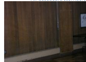
Main hall air baseboard
