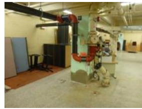
Basement is fully sprinkler protected
