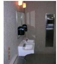
Floor, tile in good condition, restroom non-ADA compliant
