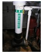
Chilled water piping and pumps
