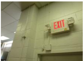
Exit Sign with Emergency Lights
