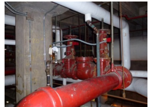
Incoming fire protection service
