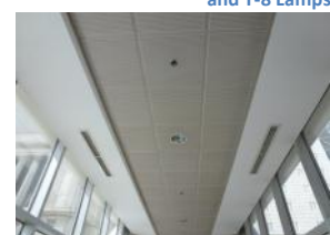
Third Floor Recessed Downlighting
