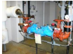
Incoming fire protection cold water line
