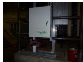
Access Control Panel
