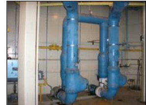
Chilled water pumps
