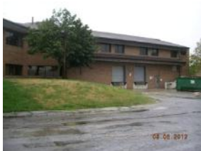
Asphalt drive to loading dock in poor condition, dock doors worn
