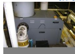
Domestic hot water heater
