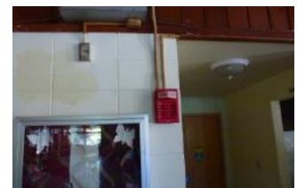
Fire alarm Strobe and Horn
