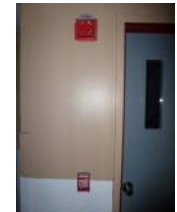
Fire Alarm Strobe, Speaker and Manual Pull Station
