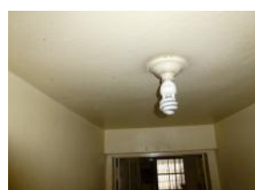
Incandescent Fixture Replaced with Compact Fluorescent Lamp
