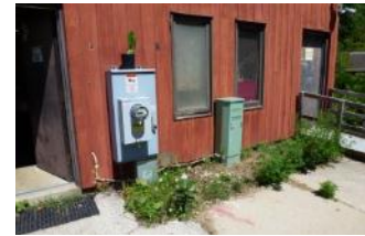
Electric Meter and Telephone Service
