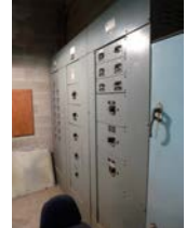
Emergency Distribution Panel P/EDP in penthouse
