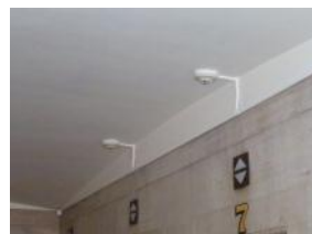
Smoke Detectors in Elevator Lobby
