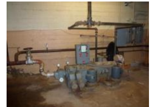
Condensate return pump
