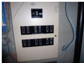
Fire Alarm Control Panel
