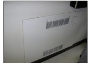
Hot water cabinet unit heater
