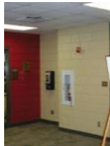
Fire extinguisher cabinet (at entrance)
