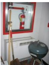
Fire hose cabinet with fire extinguisher
