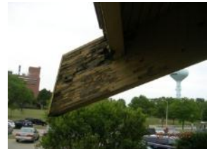
Water damage to exterior wood beam, most beams in similar condition
