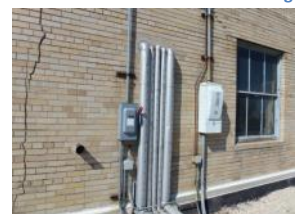
Disconnect Switches on Mechanical Penthouse
