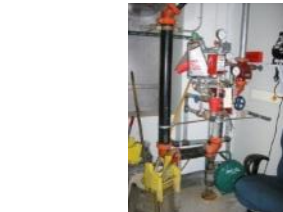
Partial fire suppression system
