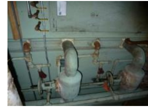
Built-up AHU steam heating coil
