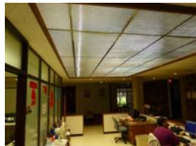
Recessed Fluorescent Lighting
