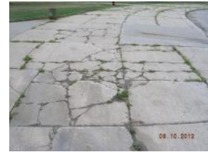
Cracks and unevenness in sidewalk create a potential tripping hazard
