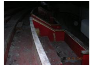
Theater seating. HVAC ductwork serving the gym currently occupies part of the seating area
