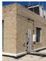
Roof penthouse exterior is in poor condition. Damaged windows, loose flashing, and large cracks in the brick wall
