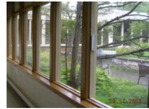
Typical storefront windows looking into the courtyard. Wood frame with single pane glazing
