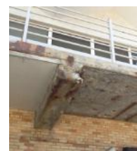
2nd floor concrete balcony by the loading dock is in poor condition
