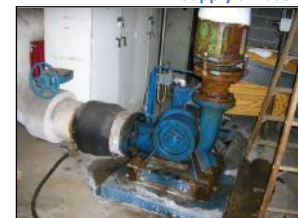
Chilled water pump
