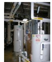
Glycol solar hot water system
