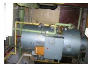
Steam to domestic HW heat exchanger
