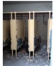
Restrooms in the theater. Peeling paint could contain lead
