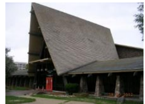
Roof shingles in fair condition, show signs of aging
