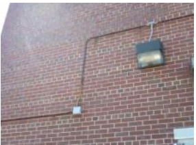
Exterior Light Fixture with Rusted Conduits
