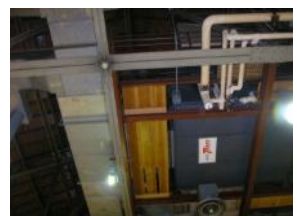
Gym air handling unit
