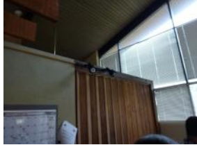
Track Mounted Lighting with Compact Fluorescent Lamps
