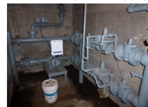
Natural gas service/gas piping
