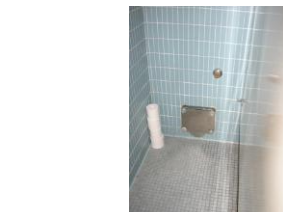
Water closet is missing
