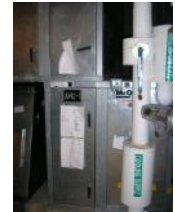
Air handling unit AHU-1 (new unit and HVAC piping)
