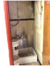
Janitors closet, deteriorated floor and wall
