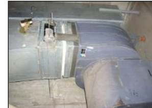
Return/relief/exhaust fan with pneumatic control dampers
