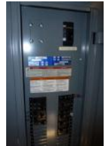
Main Distribution Panel
