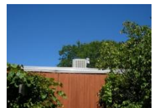
Trane air cooled condensing unit
