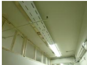
Fluorescent Strip Lighting
