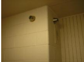
Sprinkler heads with vandal proof caps
