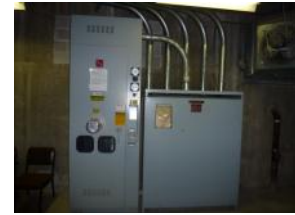
13kV Main Electrical Service
