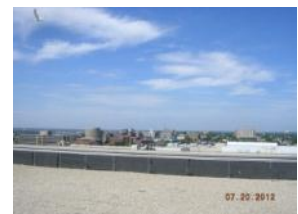
Roof, flashing generally in good condition, coping joints require tuck-pointing, sealant
