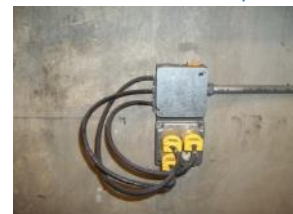
Honeywell control panel
