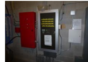
Fire Alarm Control Panel and Splice Box
