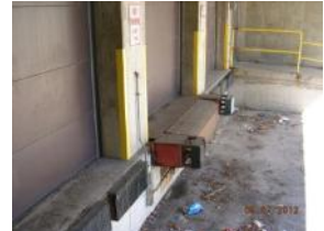
Loading dock area is filled with trash, water damage to concrete in many spots
