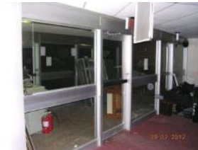
Main entry boarded up, vestibule used for storage. Ceiling and carpet are in poor condition
