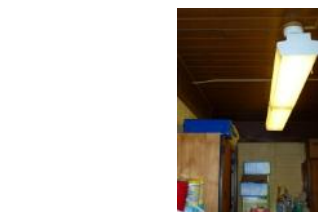
Fluorescent Fixture with T-12 Lamps
