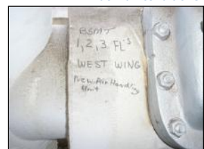
Steam main branch
