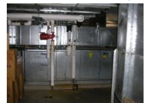
Air handling unit heating/cooling coils
