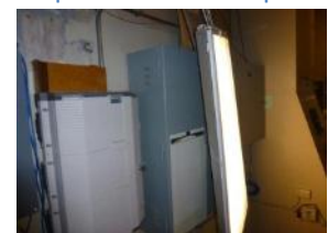
DDC temperature controls panel
