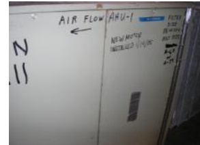
Air handling unit AHU-1
