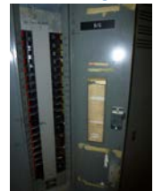
Panel B/G. Recommend Replacement
