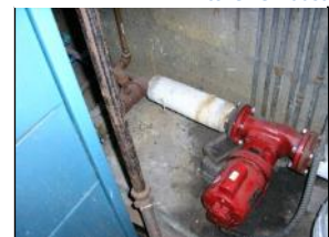
Hot water in-line pump
