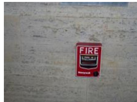
Fire Alarm Manual Pull Station
