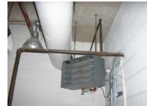
Suspended unit heater
