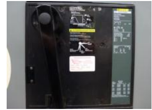
Breaker with Tested Sticker
