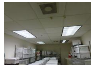
Recessed Fluorescent Fixtures
