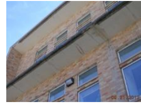
Concrete overhangs cracked, paint peeled on the underside
