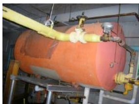
Domestic water storage tank
