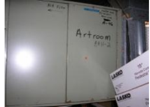
Air handling unit AHU-2
