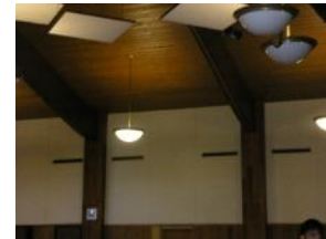
Main hall sidewall registers
