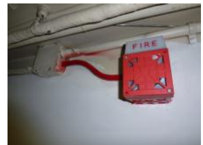
Fire Alarm Strobe and Speaker
