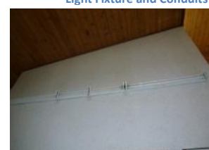
Fluorescent Light Fixture
