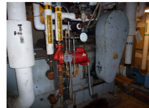
Air handling unit AHU-5
