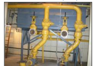
Abandoned piping and pumps
