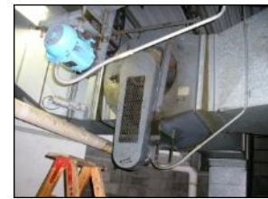
Mechanical room filtered makeup air
