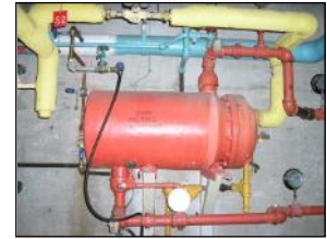
Snow melting heat exchanger
