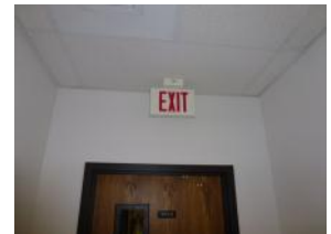
Third Floor Exit Sign
