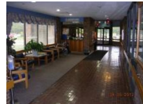
Corridor brick floors in good condition, carpet in poor condition
