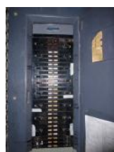
Panel B/P Located in Basement by Compressors Should Be Replaced
