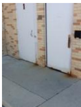
Door frames, loading dock equipment rusting
