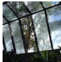
Condensate present in many of the greenhouse glass panels
