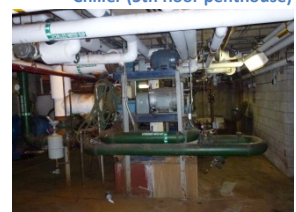
Chilled/condenser water pumps
