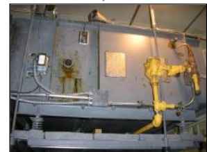
Air handling unit (steam heating coil)
