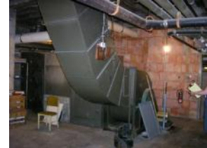
Entrance air handling unit
