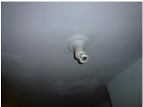
Broken Fluorescent Light Bulb
