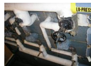
Built-up AHU steam coil
