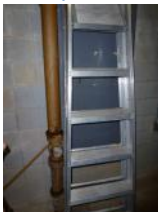
Panel with Waste Pipe and Ladder
