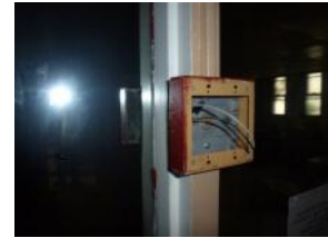
Junction Box with Exposed Wires
