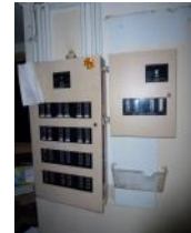
Johnson Controls Fire Alarm Control Panel
