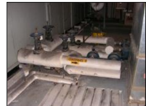
AHU condensate return piping
