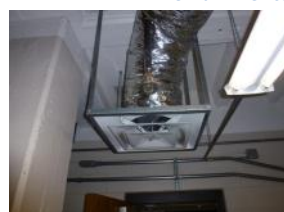
Wet Sprinkler Head in Data Room
