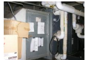
AHU cooling and heating coils
