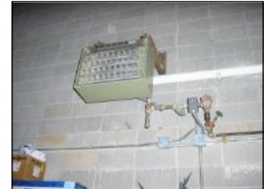
Steam suspended unit heater
