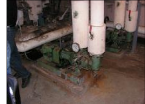
Hot water pumps
