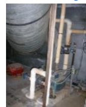
Condensate return pump
