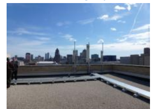
Verizon Antennas and Cabling System
