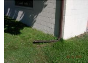
Downspouts bent at base of building
