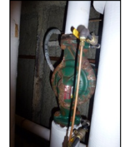
Heating coil booster pump
