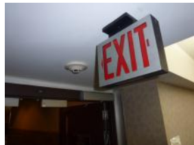
Exit Sign and Smoke Detector
