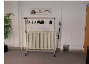
Steam radiator w/ space relief opening (original building)
