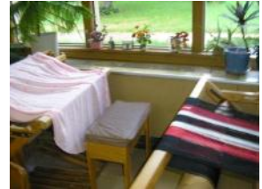
Floor mounted unit vent (original to building)
