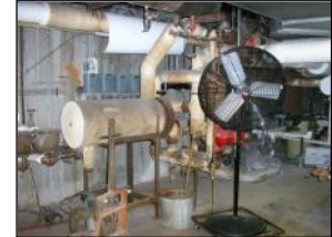
Steam to hot water heat exchanger
