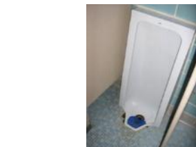
Floor mounted urinal (installed probably 1990)
