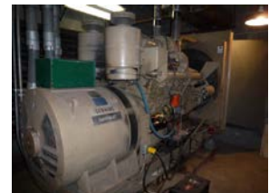
Existing 350 kW Emergency Generator
