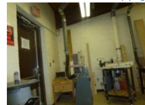
Exit Sign and Lighting
