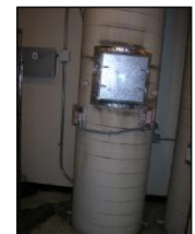
Airflow measuring station
