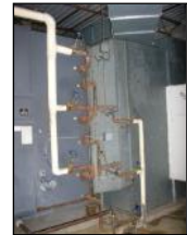
AHU steam coil section
