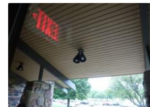
Exterior Light Fixtures with Compact Fluorescent Lamps
