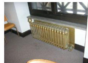
Cast iron radiator
