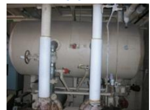
Oversized water tank
