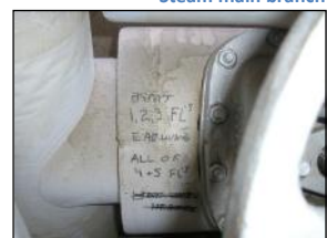
Steam main branch
