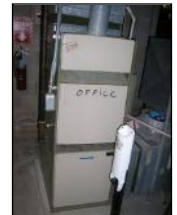
Gas furnace unit
