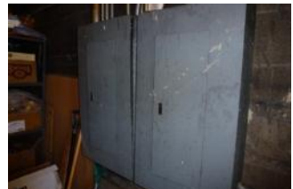
Subpanels B (right and left)
