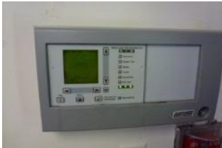
Fire Alarm Annunciator Panel
