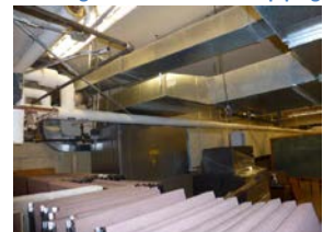
Existing ductwork and HVAC piping
