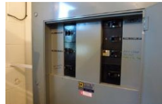
Main Electrical Panel
