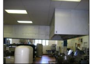
Kitchen exhaust hood (installed most probably 1980)
