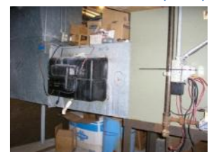
Inline humidifier and gas fired section (AHU-2)
