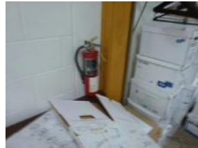
Hand held ABC type fire extinguisher
