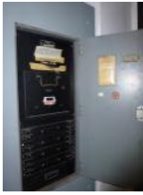
Branch Circuit Panel LC/88
