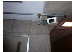
Exterior Security Camera
