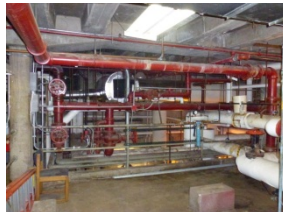
Fire protection system
