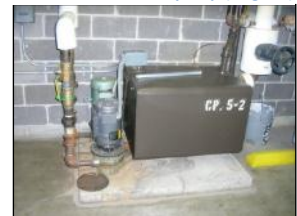
Condensate return pump (recently replaced)
