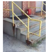
The main entrance is in poor condition: concrete steps damaged and railings rusting. The entry is not HC accessible
