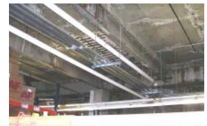
Basement structure with parking lot above. Water damage has caused corrosion of steel beams, deterioration of concrete slab
