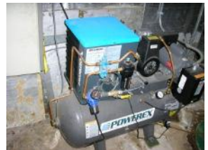
Temperature control air compressor (new)
