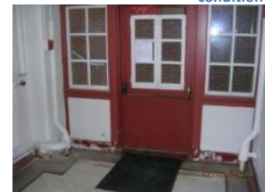
Wood doorway to exterior worn, water damage
