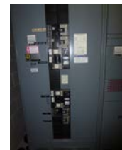
Substation USS/3 Installed 1991
