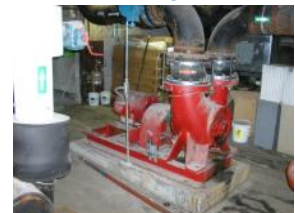
Condenser water pump
