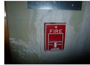
Fire Alarm Pull Station on 6th Floor
