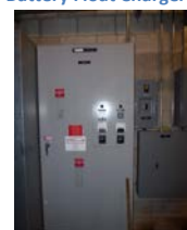
ATS-1 in Room 142 for 250kW Generator
