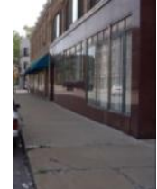
Stone panels cracked, shifting from water damage, wear and tear. The sidewalk is also damaged
