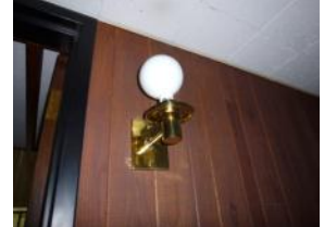
Wall Mounted Light Fixture
