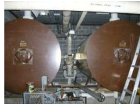
Storage tanks with circulation pumps
