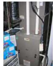
Lennox gas furnace unit (upflow)
