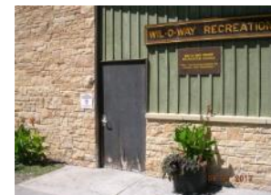
Exterior doors are in poor condition
