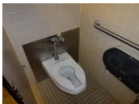
Lavatory with flush valve
