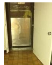
Most doors are worn, do not have non-ADA compliant hardware
