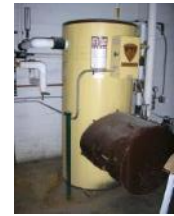
Steam to domestic HW heat exchanger
