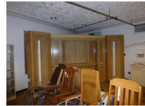
Upright sprinkler heads
