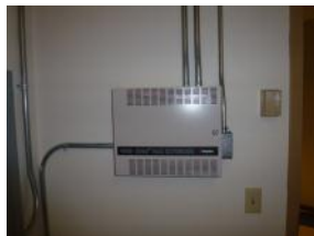
Simplex Fire Alarm NAC Panel
