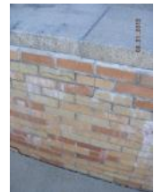
Brick walkway walls have incurred water damage
