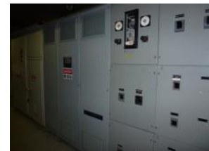
4160V Substation USS-23A
