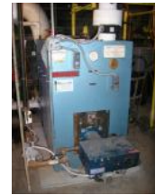
Hot water boiler
