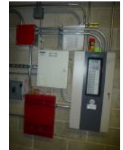
Fire Alarm Panels
