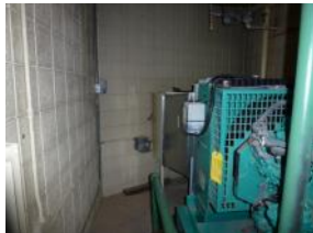
30kW Diesel Generator
