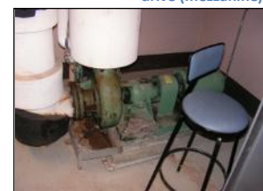
Chilled water chiller pump
