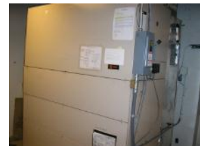
Self contained AHU
