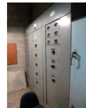
Emergency Distribution Panel P/EDP in penthouse
