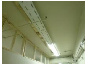
Upright sprinkler head with piping
