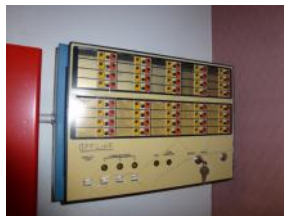
Cell Door Status Panel
