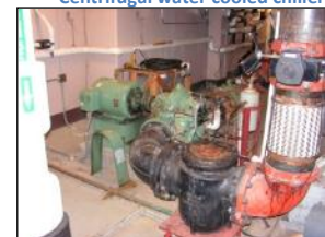
Cooling tower water pump
