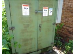
Incoming Electrical Service
