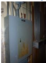
Panel BF/G with Rust
