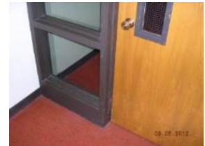
Door and frame in poor condition, non-ADA compliant door hardware
