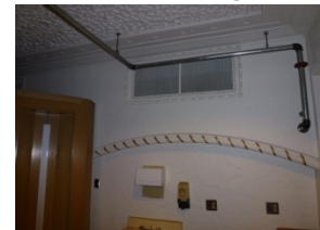
Fire piping with sprinkler heads
