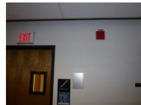
Exit Sign and Fire Alarm Strobe
