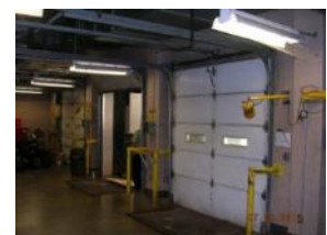
Loading dock doors in poor condition
