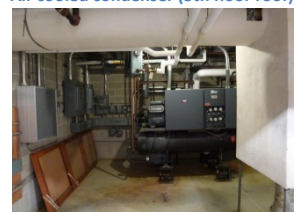
Chiller (5th floor penthouse)
