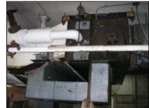
Air handling unit (appears original to building)
