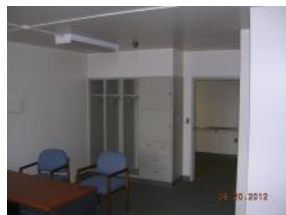
Typical office with individual bathrooms, non-ADA compliant hardware
