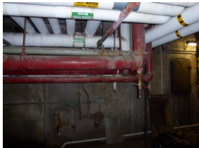
Fire protection piping
