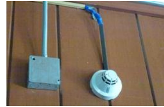
Smoke Detector Wiring Taped
