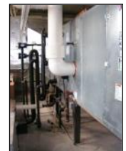
2003 air handling unit
