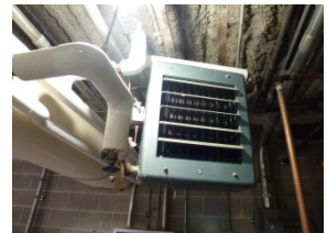
Suspended unit heater
