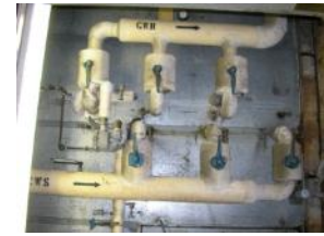
Modular AHU cooling coil
