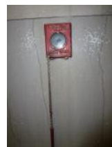
Fire Alarm Device
