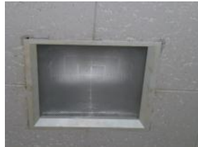
Recessed Fluorescent Light
