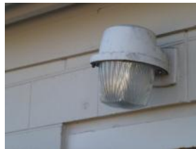
Exterior Light Fixture
