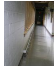
Air baseboard (corridor)
