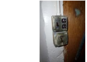
Basement Light Switches and Receptacles
