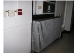
Cast iron radiator
