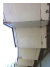
Water hasn't dripped properly off the edge of the concrete roof overhang, causing damage
