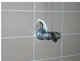
Plumbing check valve in damaged wall
