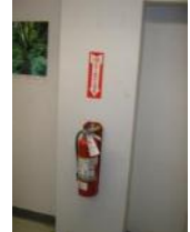
Wall mounted fire extinguisher
