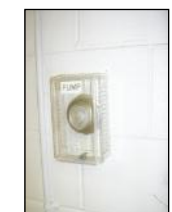
Thermostat (in-line pump/valve control)
