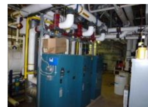
Hot water boilers
