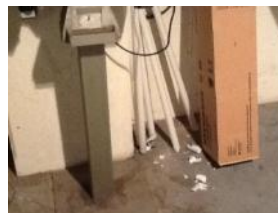
Broken fluorescent lamps found in a few places in the basement mechanical rooms and hallways
