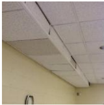
Some ceiling tile in dining hall beyond useful life, stained from mechanical pipe leaks above
