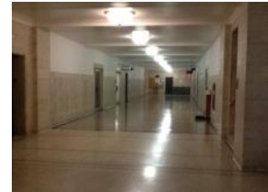
Typical upper floor corridor. Floor, walls, ceiling generally in good condition, wear and tear evident in a few areas
