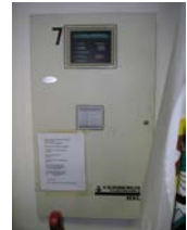
Fire Alarm Annunciator Panel
