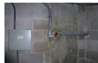
Corroded existing electrical conduit
