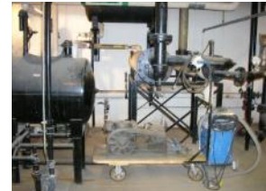
Steam to heating HW heat exchanger
