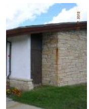
Exterior stone stained in a few areas, generally in good condition
