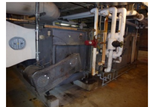
Air handling unit AHU-4
