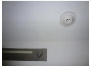
Smoke Detector Near Elevators
