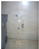
Missing drinking fountain
