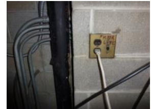
Light Switch and Receptacle
