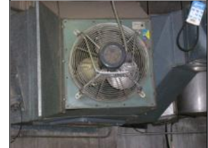
District heating/cooling plant
