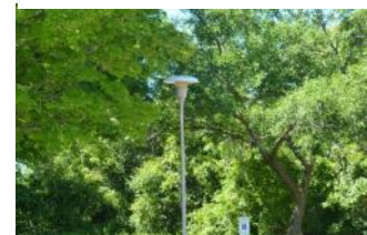
Parking Lot Light Pole
