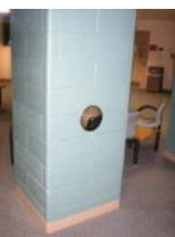
Wall cleanout cover plate
