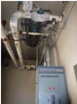
MCC Section with Tank Above
