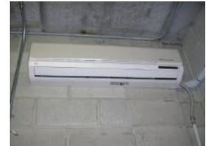
Ductless split system indoor unit
