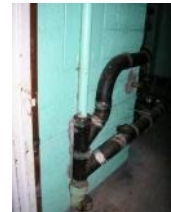
Sanitary & vent piping
