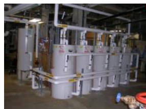
Hot water tanks for roof-mounted solar hot water system
