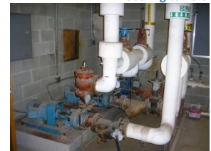
Chilled water pumps (9th floor penthouse)
