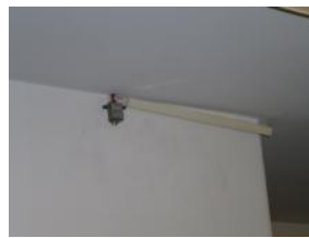
Wire mold and Box
