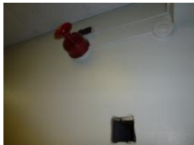
Fire Alarm Horn in Basement
