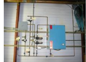
Temperature control refrigerated air dryer
