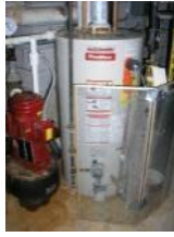
Domestic water heater
