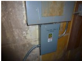
Rusted Panel BF/G
