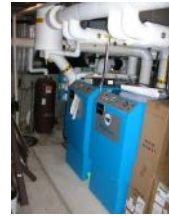
Hot water boilers
