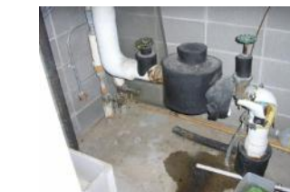
Water meter for the building
