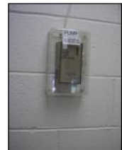
Thermostat (in-line pump/valve control)
