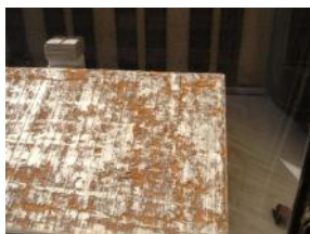
Gymnasium roof in poor condition
