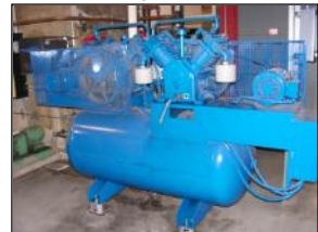
New air compressor (roof penthouse)
