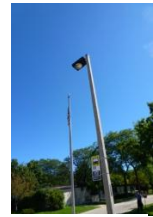
Existing parking lot light
