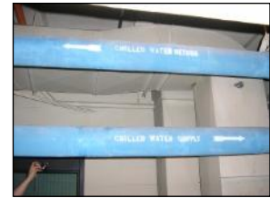
Chilled water piping
