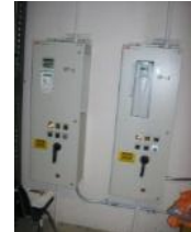
Return air fan variable frequency drive
