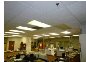
Fluorescent Light Fixtures
