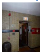
Fire Alarm and Exit Sign in Gymnasium
