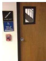
Stairwell door. Many of the building's doors do not have ADA-compliant hardware.
