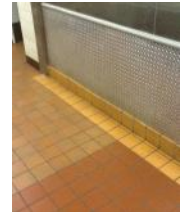
Floor is generally in good condition, tile has been replaced in various areas over time
