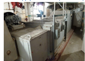
Air handling unit (3rd floor mech room)
