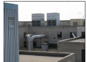
Cooling towers/exterior ductwork
