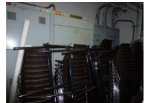
Main Switchboard and Distribution Section
