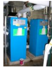
Hot water boilers
