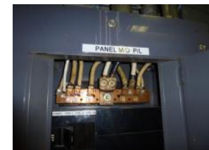
Panel MD/PL with Exposed Bus and Lugs
