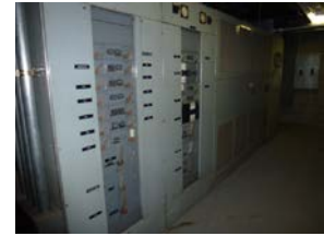
Substation USS/1 Installed 1964
