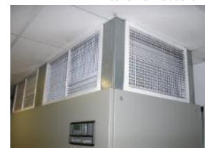
Data room self-contained air conditioner
