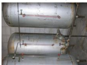
Hot water expansion tanks
