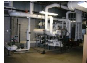
Steam to heating HW heat exchangers
