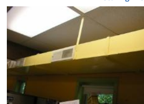
Supply ductwork and registers
