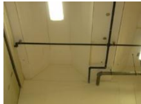
Upright sprinkler heads and piping
