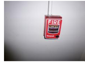
Fire Alarm Pull Station
