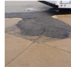
Handicap ramp patched over with asphalt, in poor condition
