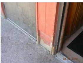
Exterior wood panels, doors worn in some areas, particularly south façade
