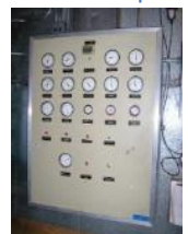
Pneumatic temperature control panel
