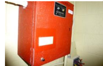
Existing fire alarm control panel
