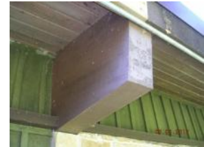
Cleaning and paint needed on exterior, otherwise in good condition
