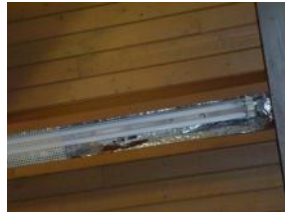
Fluorescent Light Fixture
