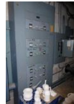
Existing main distribution section
