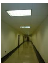
Recessed Fluorescent Lighting
