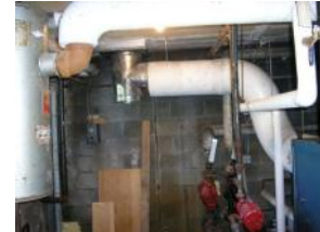
Zone hot water in-line pumps
