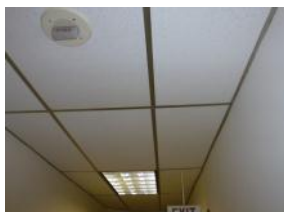
Fourth Floor Fire alarm Devices and Lighting
