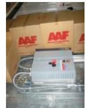
Return fan variable frequency drive
