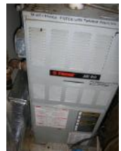
Trane gas furnace unit
