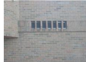
Unit ventilator outdoor air intake louver
