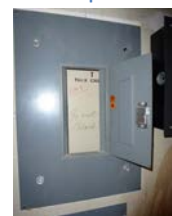
Emergency Panel. Recommend Replacement
