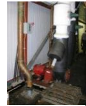
Chilled water pump
