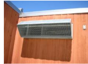
Outdoor air intake
