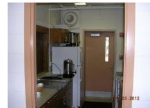
Kitchen non-ADA compliant, poor condition
