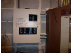
Johnson Controls Fire Alarm Panel
