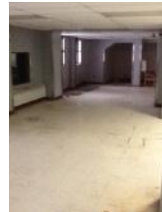
Floor, ceiling, and walls deteriorated
