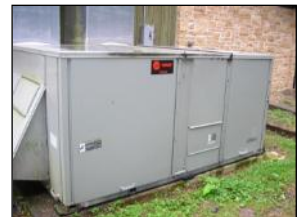
Grade mounted cooling only rooftop unit
