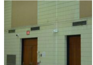
Gym Life Safety Equipment without Wireguards
