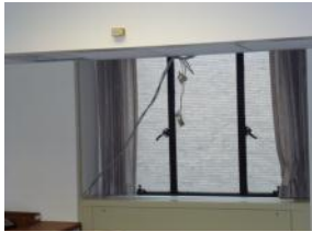
Wires Hanging From Ceiling
