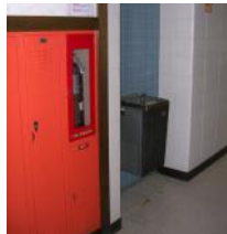
Non-ADA compliant drinking fountain
