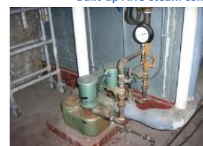
Condensate return pump
