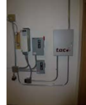
AHU-2 variable frequency drive
