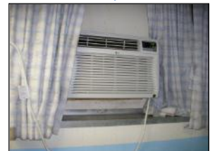
Window air conditioner
