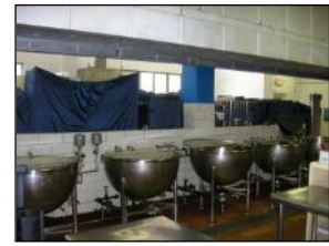
Steam powered kitchen equipment
