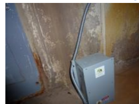
Equipment Not Mounted to Wall
