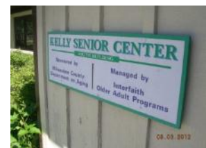
Exterior wood siding in poor condition
