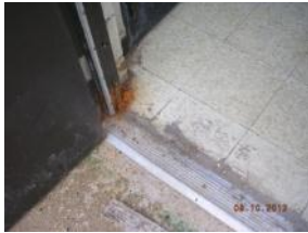
Exterior door and frame in poor condition, damage to threshold and floor
