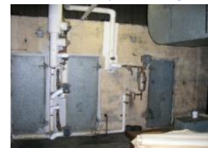
Built-up air handling unit
