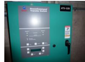
Automatic Transfer Switch
