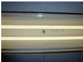
Light Fixture with T-8 Lamps
