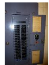
Existing Sub Panel A
