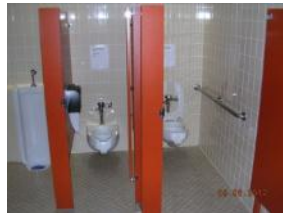
Restroom floor and wall tile typically in good condition, HC stall, vestibule non-ADA compliant
