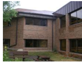
Façade appears to be in good condition, along with the windows and brick sills
