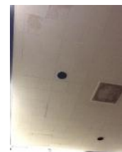
7th floor children's courtroom ceiling tile, wall panels, and carpet are aged
