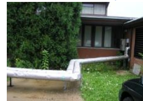
Condenser water piping
