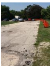
Asphalt drives and parking lot are beyond their useful life
