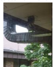
Snow Melt Cable Receptacles
