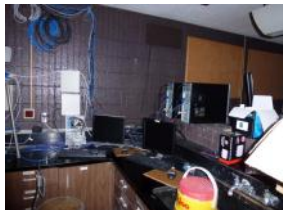
Computer and Network Cabling in Dark Room
