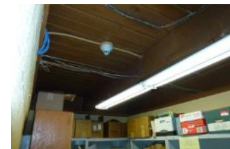
Lighting, Heat Detector and Telecom Cables
