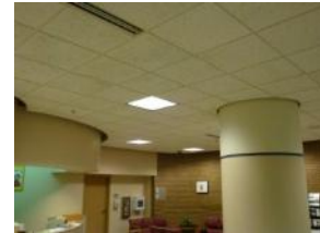
Ceiling linear slot diffusers
