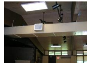
Supply ductwork (Main Hall Room)
