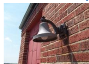
Incandescent roof light fixture
