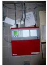
Fire Alarm Panel
