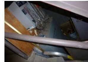
Telephone Service Equipment
