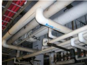
Cold water piping
