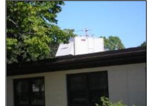
Cooling only rooftop unit (west)
