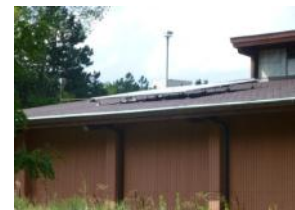
Roof Mounted Solar Panels
