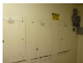
Electrical Branch Panels
