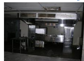
Kitchen exhaust hood
