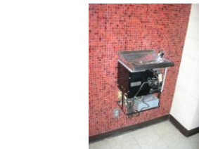
Cover is missing for electric water cooler
