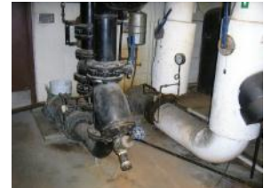
Chilled/condenser water pumps
