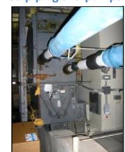
Air handling unit (cooling coil)
