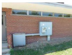
Incoming Electrical Service Meter
