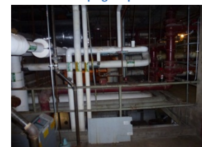
Fire protection: Wet pipe riser
