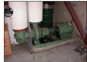
Heat recovery loop pump
