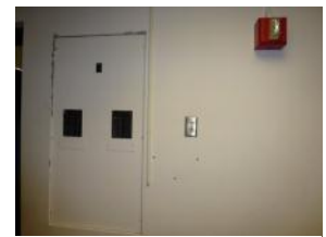
Basement Branch Circuit Panel Missing Cover
