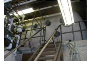
Hot water storage tank
