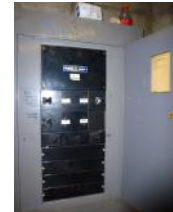
Panel Located in Basement Should Be Replaced
