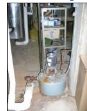
Condensate return pump
