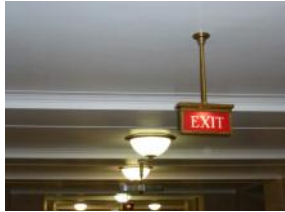
Decorative Lighting and Exit Sign
