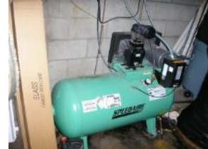
Temperature control air compressor (new)
