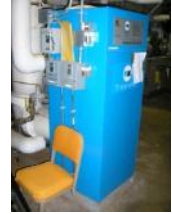
Hot water boiler
