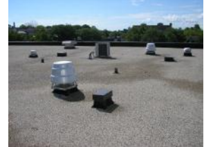
Exhaust fans & split system outdoor unit
