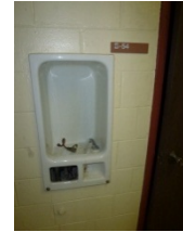
Abandoned drinking fountain
