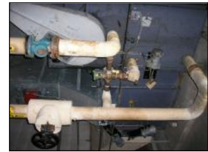
Air handling unit
