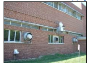
Kitchen sidewall/dishwasher fans
