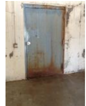
Loading dock entrance door to the basement. Extensive water damage to the floor slab, wall, and door
