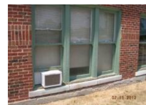
Air conditioning units are common throughout the building in wood windows that are deteriorating and should be replaced with energy efficient aluminum type
