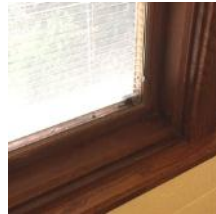
Typical storefront window. Wood frame with integral louvers, hardware on some windows broken
