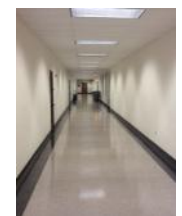
Typical corridor. Floor, walls, and ceiling generally in good condition, wear and tear evident in some areas
