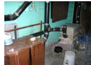
Indoor grease trap
