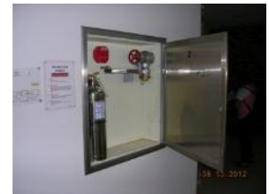
Fire hose cabinets converted to portable extinguisher cabinets
