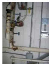
Non potable water
