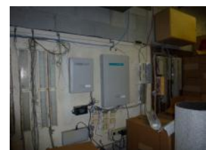
Incoming Telephone Service Equipment
