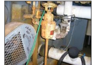
Air handling unit valving
