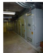
WE Energies Switchgear
