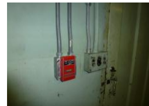
Johnson Controls Fire Alarm Device
