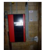
Fire Alarm Panel
