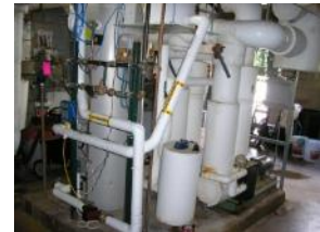
Glycol solar hot water system
