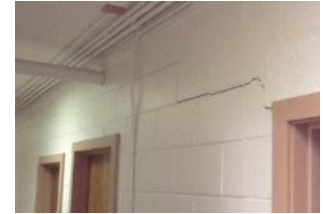
Growing cracks in multiple walls
