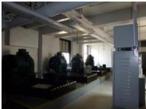
Elevator Equipment Room
