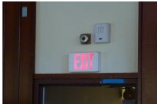
Exit Sign without Battery Backup
