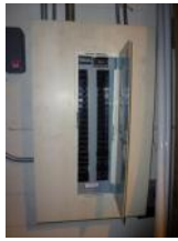
Branch Circuit Panel
