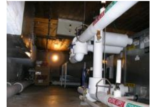
Air handling unit AHU-2 (new unit and HVAC piping)
