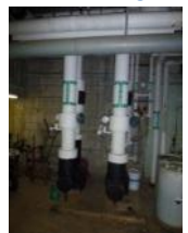
Chilled water pumps
