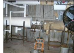
Steam to hot water heat exchangers
