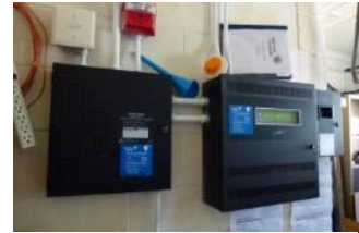
Fire Alarm Control Panel
