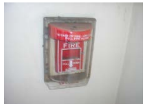
Fire Alarm Pull Station
