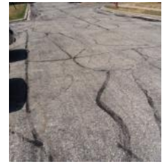
Parking lot in poor condition
