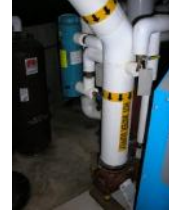
Hot water piping/pump
