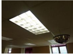
Office Lighting and Security Camera
