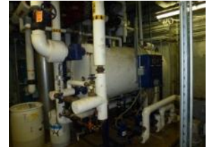
Steam boiler feed system
