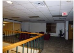
Exit Sign and Ceiling Lights
