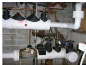
Incoming cold water service
