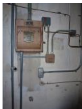
AHU Disconnect Switch. Recommend Replacement
