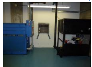
Elevator machine room air conditioner
