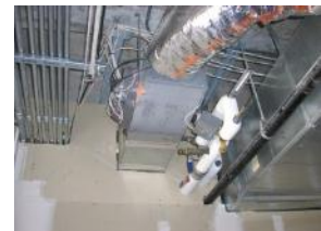
Variable air volume box with reheat coil
