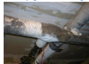
Asbestos pipe insulation
