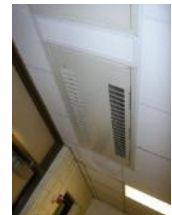
Ceiling cabinet unit heater (at entrance)
