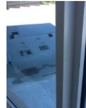
Circular roof is patched in various areas
