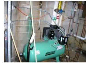
Temperature control air compressor (new)
