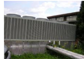
Air cooled chiller with remote evaporator
