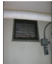
Makeup air louver (kiln room)
