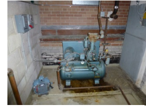
Temperature controls air compressor
