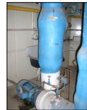
Chilled water pump
