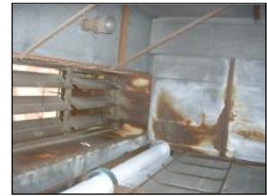
Built-up AHU outdoor air intake section (interior)
