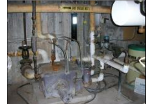
Condensate return pump
