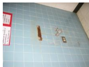
Plumbing fixture is missing
