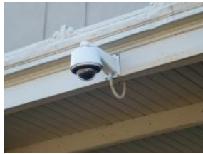
Exterior Security Camera
