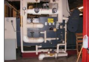
Air handling unit steam coil
