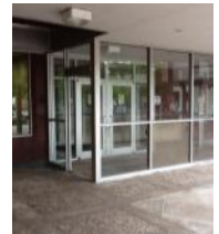
Storefront entrance beyond useful life, sidewalk is worn
