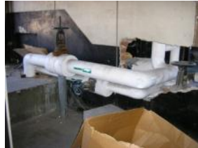
Incoming cold water service
