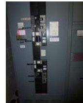
Substation USS/3 Installed 1991
