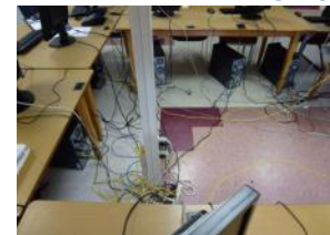
Computer Lab 2102-13 Power Wiring
