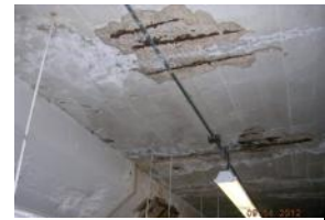
Basement in generally good shape, some areas have salt, water damage
