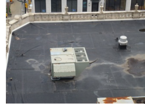
Rooftop unit/exhaust fan
