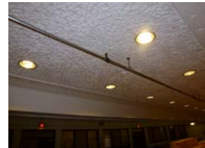
Recessed Down Lights
