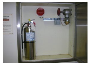
Fire Extinguisher with Cabinet
