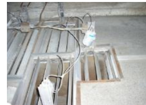
Outdoor air intake pneumatic control dampers
