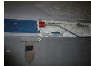
Fire Alarm Junction Box
