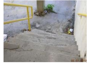
Loading dock stairs are cracked, large pieces have broken off. Not safe to use
