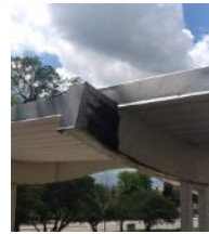
Entrance canopy in poor condition: wood rotting & metal rusting. Canopy scheduled to be replaced
