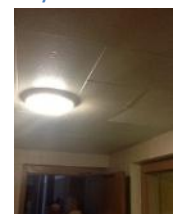
Concealed spline ceiling tile in kitchen and stage area nearing end of useful life
