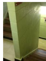
Stairwell handrails only on one side, paint worn off the wall in a couple areas
