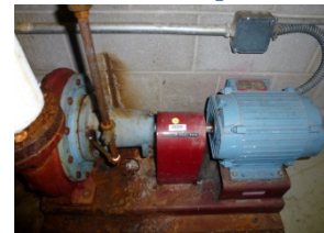
Cooling coil pump
