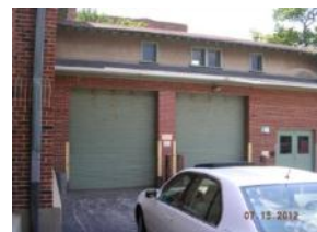
Rolling doors are non-insulated, worn
