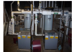
Gas fired water heaters for 5-story and 9-story buildings
