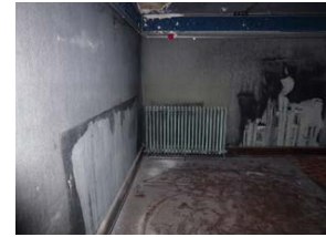
Cast iron radiator
