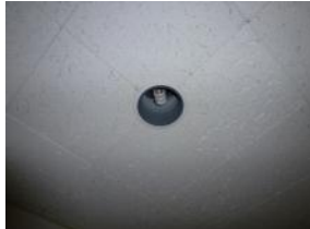
Recessed Light Fixture with Compact Fluorescent Lamp
