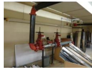
The sprinkler main, 6" size
