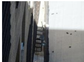
Flood Lights in Courtyard Area
