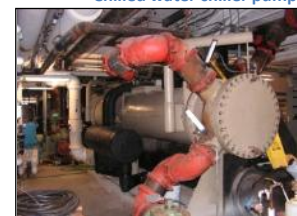
Centrifugal water cooled chiller
