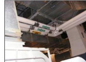
Steam and chilled water piping
