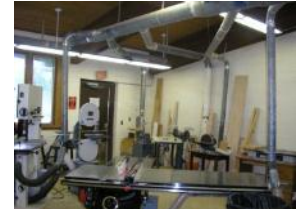
Woodshop dust collection system
