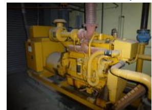
205kW Emergency Generator
