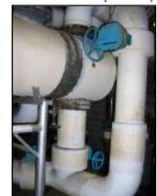
Steam to hot water heat exchanger
