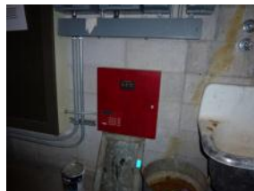
Fire Alarm Panel
