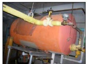
Steam to DHW heat exchanger
