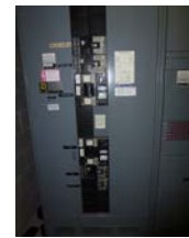
Substation USS/3 Installed 1991
