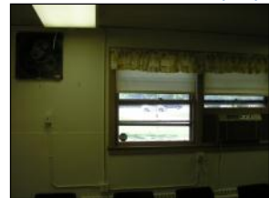
General exhaust (wall propeller exhaust fan)
