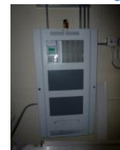
Fire Alarm Panel
