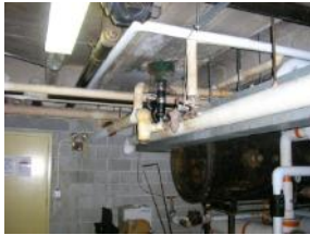
Galvanized plumbing piping
