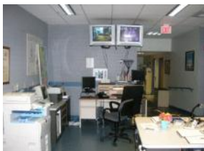
Fire sprinkler (concealed type)
