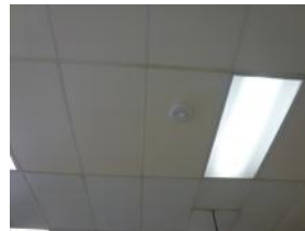
Lighting and Fire Alarm Device
