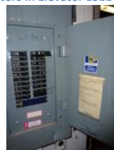
SquareD Branch Panel
