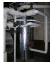
Steam to domestic HW heat exchanger
