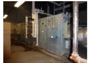
Air handling unit
