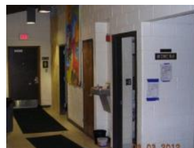
Drinking fountain non-ADA compliant – located too high
