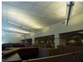
Remodeled Floor Lighting
