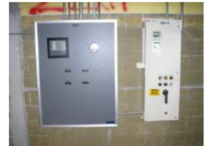
DDC/pneumatic control panel and VFD
