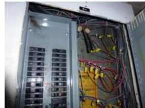
Panel BE/G is Missing Internal Cover
