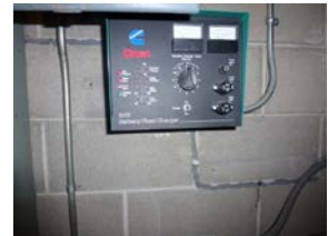
Generator Battery Float Charger
