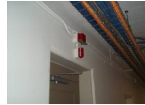
Fire alarm conduits, junction boxes, cable tray in corridors
