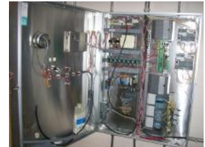
DDC/pneumatic temperature control panel
