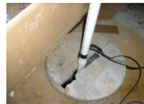
Drain tile & elevator sump pump
