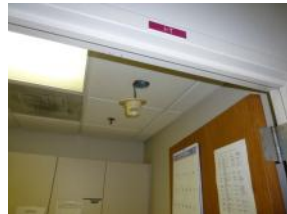
Smoke Detector Detached from Ceiling
