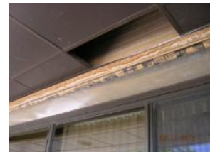
Missing soffit tiles on south façade
