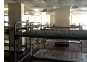
Ceiling tiles sagging, carpet worn & in poor condition
