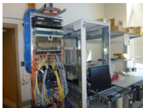
Existing Racks in Data Room
