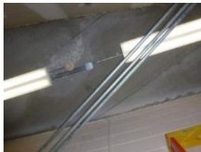
Electrical Room Lighting
