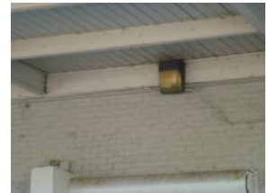
Exterior Light Fixture
