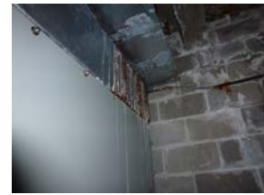
Corrosion on WE Energies Switchgear
