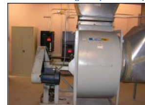
Centrifugal return fan and VFD drive (mezzanine)
