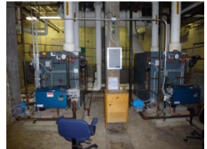
Hot water boilers for domestic water
