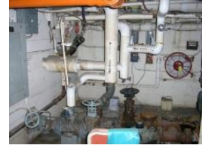
Incoming cold water service
