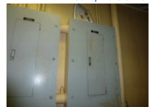
Branch Circuit Panels
