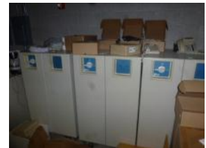
UPS system for Comm. System
