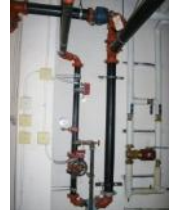
Fire protection piping
