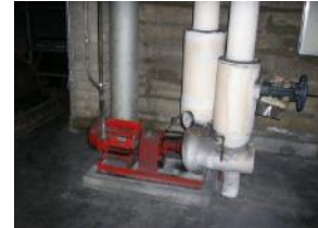
Hot water pump
