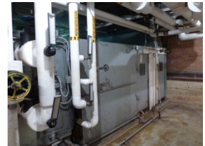
AHU-4 heating/cooling coil/filter sections
