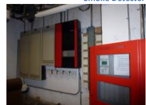
Fire Alarm Control Panels
