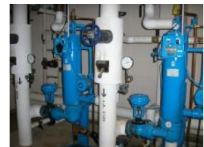
Steam to domestic HW heat exchangers
