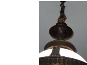
Corridor Light Fixture with Wire Splice
