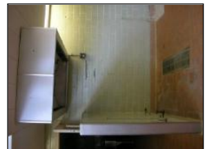
Kitchen exhaust hood (kitchen equipment underneath removed)
