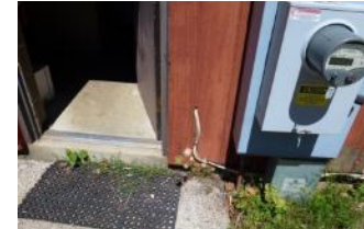
Incoming Telephone Lines
