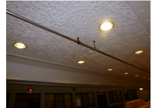
Exposed fire piping with sprinkler heads
