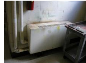
Hot water cabinet unit heater
