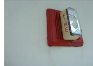
Fire Alarm Strobe
