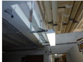
Fluorescent Light in Basement
