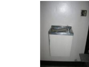
Wall mounted drinking fountain
