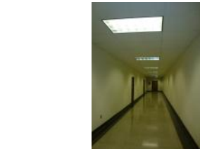
Recessed Fluorescent Lighting
