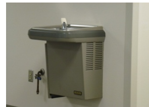
Disconnected drinking fountain
