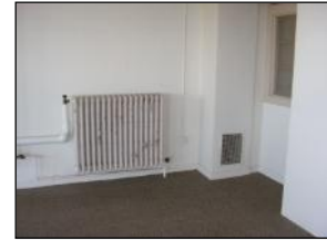
Steam radiator w/ space relief opening (4th and 5th floor)
