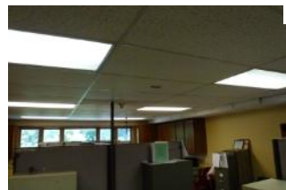
Fluorescent Lighting with T-12 Lamps
