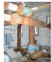
Condenser water piping (not insulated)
