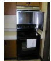
Kitchen range oven with kitchen exhaust hood
