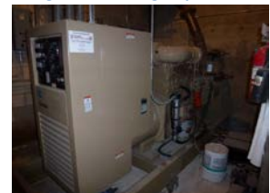
Original 250kW Backup Generator
