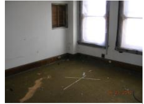
Floors, walls, ceilings, and windows in many of the 2nd floor rooms are in poor condition
