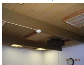
Wood plank ceiling is in good condition, some light fixtures are near the end of their useful life
