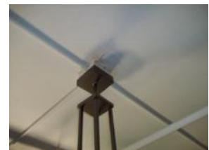
Light fixture in vacant tenant space with rust on junction box due to leak in ceiling
