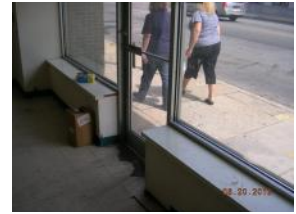
Typical storefront door on 27th street in vacant space. The floor is in poor condition, door does not have panic hardware
