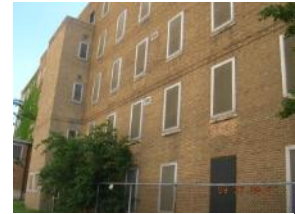
Metal screens over windows rusting, other windows boarded up. Brickwork, window sills stained
