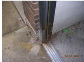
Some exterior door frames are worn or corroded, main entrance doors to be replaced
