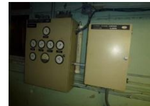
Pneumatic temperature controls panel
