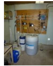
Chemical feed system
