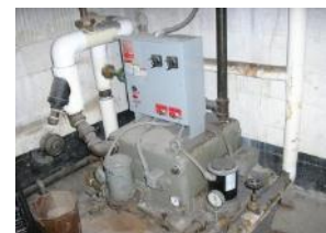
Condensate return pump
