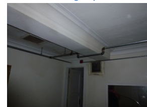
Fire water pipes with sprinkler heads
