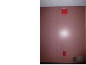
Fire Alarm Strobe, Speaker and Pull Station
