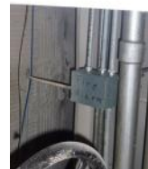
Fire Alarm System Junction Box
