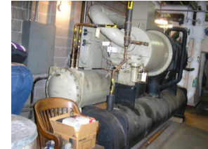
Chiller (9th floor penthouse)
