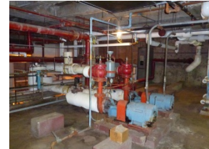
Hot water pumps (basement)
