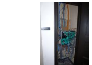
Closet MU6-8 Converted to Network Closet
