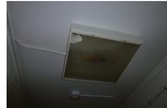
Light Fixture with Cracked Lens
