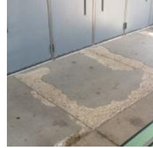
Sidewalk in poor condition in front of entrance doors
