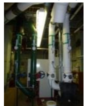
Chilled/condenser water piping (at indoor chiller)
