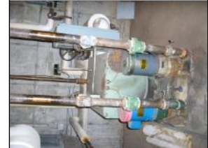
Condensate return pump
