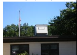
Cooling only rooftop unit (east)
