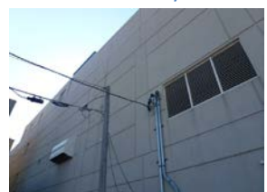
Intake/relief wall louvers
