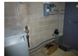
Transformer and Panel MD/PL
