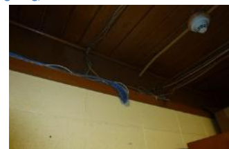
Heat Detector and Telecom Cables
