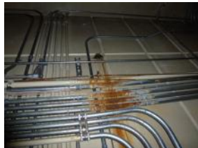
Rusted Conduits in Building F
