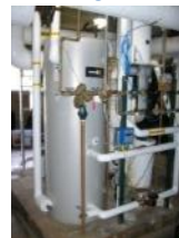
Solar DHW tank
