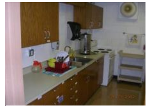
Kitchen non-ADA compliant, casework worn
