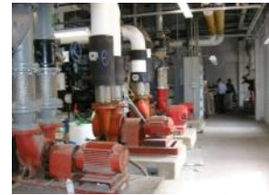
Chiller/cooling tower/chilled water pumps
