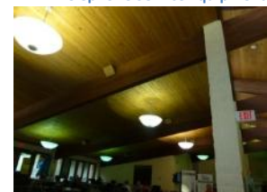
Main Hall Lighting
