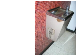
Electric water cooler
