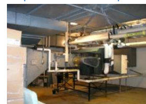
Central station air handling unit
