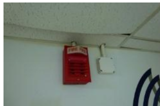
Fire alarm Strobe and Horn
