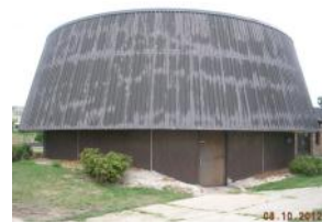
Paint on corrugated metal worn throughout the façade
