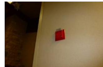
Fire alarm horn and strobe
