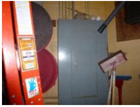
Existing Electrical Panel
