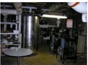
Domestic hot water storage tank
