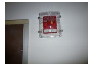
Fire Alarm Horn and Strobe
