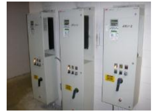
Air handling unit variable frequency drive
