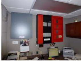
Fire Alarm Control Panel
