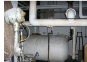
Steam to domestic HW heat exchanger
