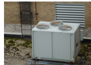
Air cooled condensing unit and wall louver
