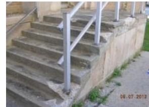
Concrete exterior stairs deteriorated, railings potentially unstable
