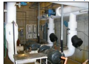
HW/CHW pumps and variable frequency drives
