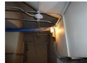
Smoke Detector and Network Cabling
