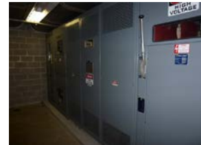
Substation USS/3 Installed 1991
