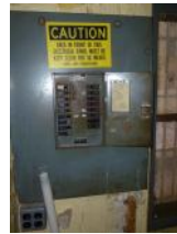
Third Floor Branch Circuit Panel
