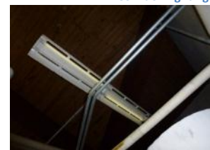
Light Fixture and Conduits
