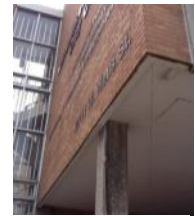
Steel beams rusting significantly on exterior
