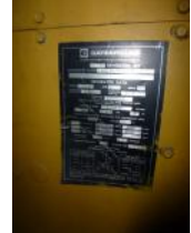
205kW Generator Nameplate
