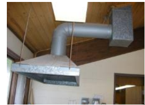
Kiln exhaust hood
