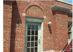
Missing light fixture on roof
