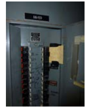
Federal Pacific Branch Panel
