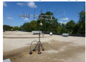
Roof Mounted Antenna
