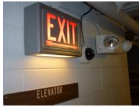
Exit Sign, Security Camera and Emergency Battery Pack Fixture
