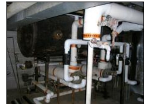
Steam to domestic HW heat exchangers
