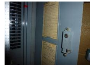
Existing Branch Circuit Panel
