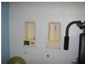
Old plumbing fixtures
