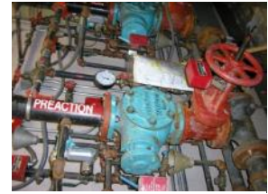
Performance of better maintenance needed
