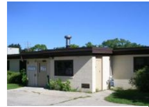
South entrance in poor shape
