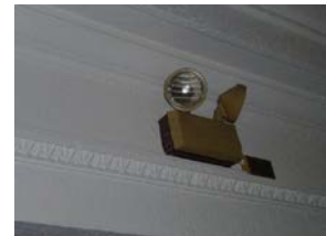
Emergency Battery Pack Light Fixture
