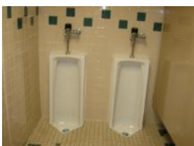
Floor mounted urinals
