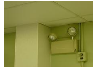
Emergency Lighting Fixture
