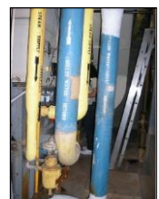
Steam/chilled water piping
