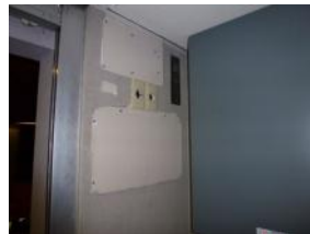
Wall Plates with Connectors Removed
