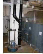
Central station AHU steam heating coil and condensate return pump
