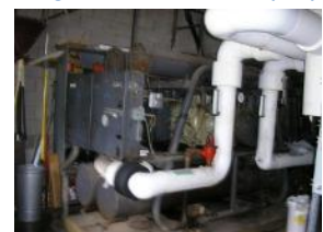
Chilled water piping
