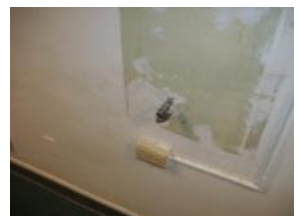
Missing drinking fountain
