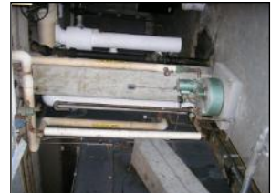
Condensate return pump
