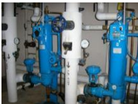
Steam to heating HW heat exchangers
