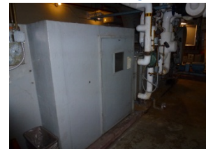
Air handling unit AHU-5
