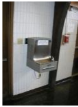
Electric water cooler
