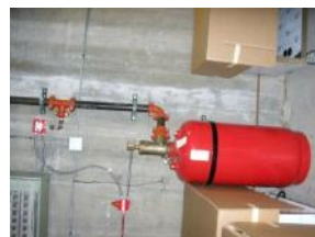
Electrical room Halon system
