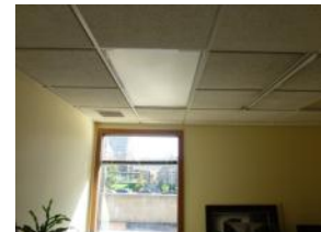
Recessed Fluorescent Lighting
