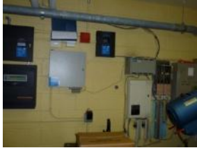
Fire Alarm Control Panels
