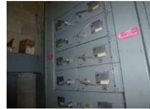
Main Distribution Panel
