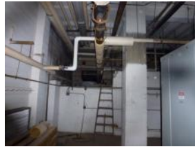
Condensate and Steam Piping Over Electrical Gear
