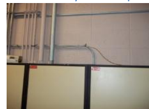
Sensor wiring is not in conduit
