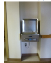
Electric water cooler
