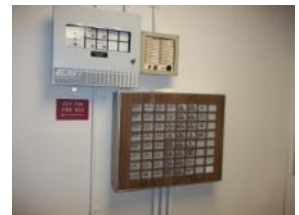
Fire alarm annunciator panel
