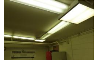
Existing light fixtures
