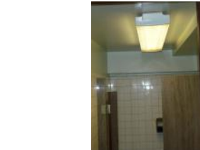
Fluorescent Lighting in Toilet Room
