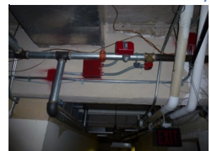
Fire pipe with tamper switch
