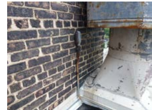
Corroded Conduit on Roof
