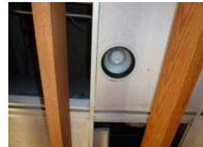
Recessed Light Fixture with Incandescent Lamp
