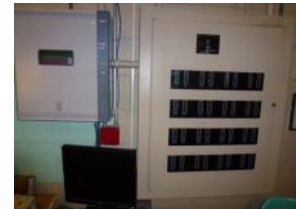
Fire Alarm Panels
