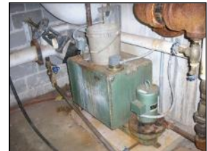
Condensate return pump (original)
