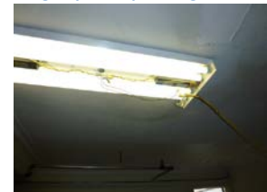
Light Fixture with Temporary Wiring. Recommend Wiring be Replaced
