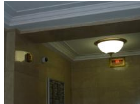
Security Camera, Exit Sign and Lighting
