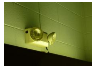
Emergency Battery Pack in Pool
