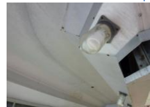
Compact Fluorescent Lamp in Kitchen Hood
