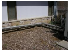
Chilled water piping (outdoor)
