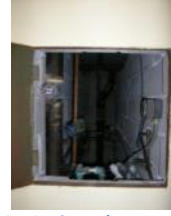
Plumbing piping in chase (appears original to building)
