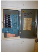
Panel in Sheriff's Office Need Replacing
