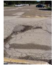
Asphalt pavement near end of useful life. Driveway is in especially poor condition
