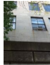
Visible staining on stone cladding from windows, retention wall dirty. Window AC units on the 2nd & 4th floors
