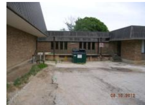
Asphalt drive is beyond useful life, landscaping and overall appearance of loading dock area is poor
