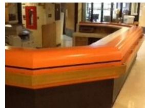
Original control desks in patient units, door lock control system outdated, new paint desirable
