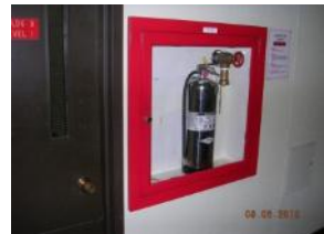
Fire hose cabinets converted to house extinguishers, fire stair door hardware non-ADA compliant, original signage
