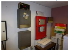
Fire Alarm Panel
