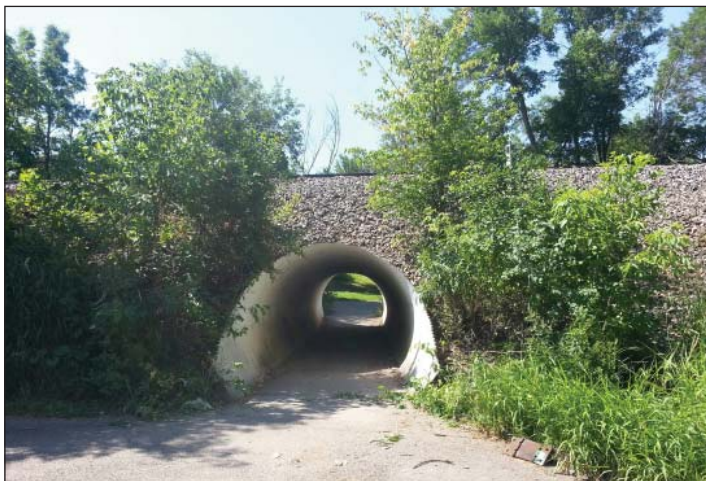
Existing tunnel at Hansen Golf Course is too short for bicycle users.
