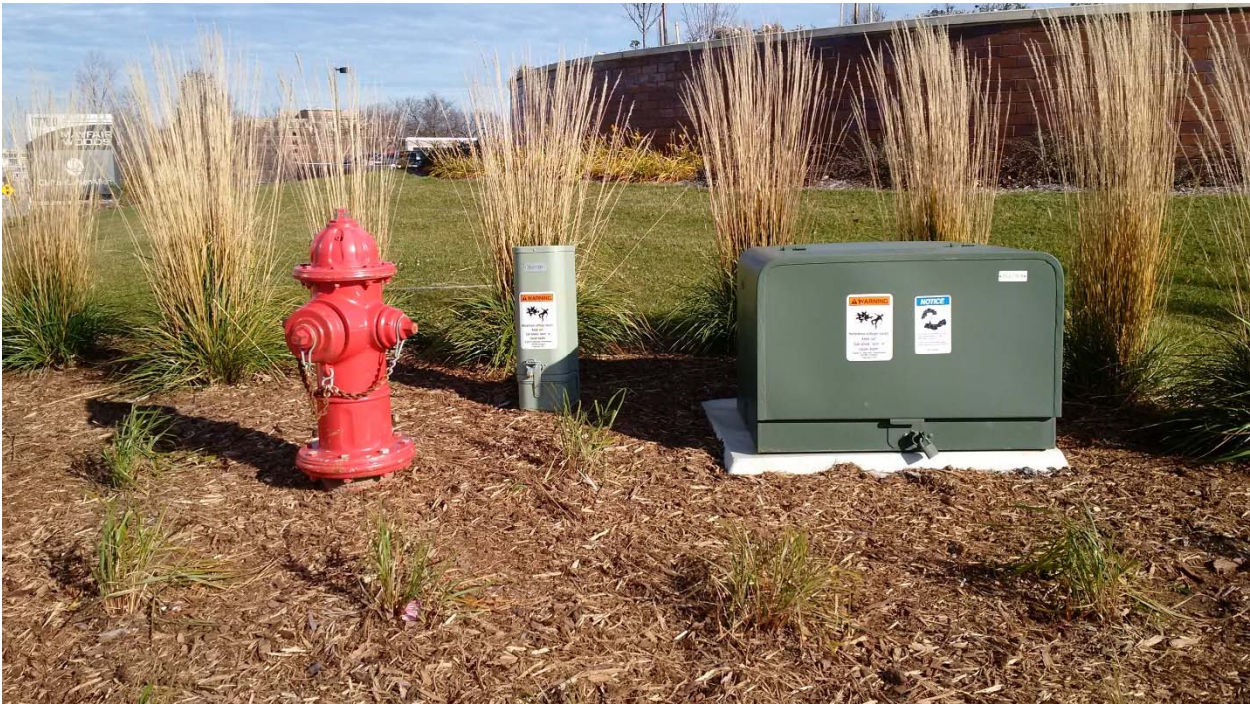
Single-Phase Transformer and Distribution Pedestal
