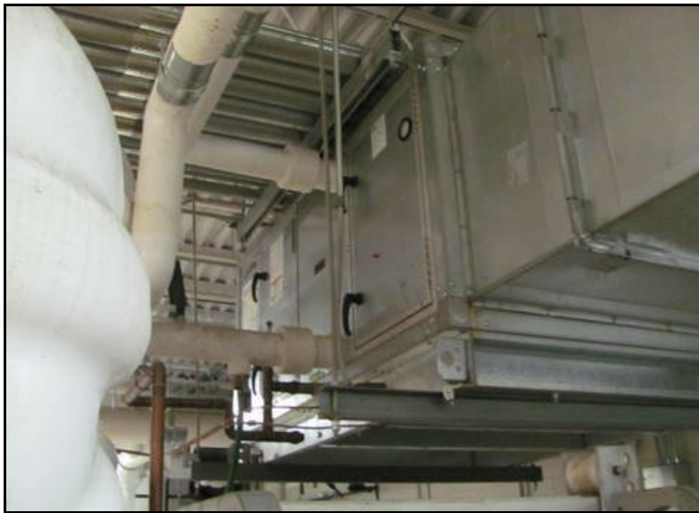
Air handling unit serving War Memorial electrical room
