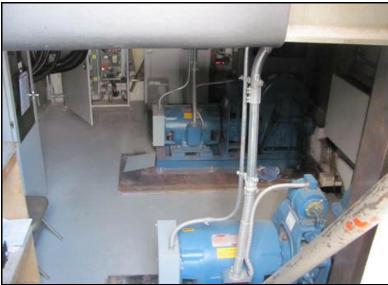
War Memorial traction elevator equipment
