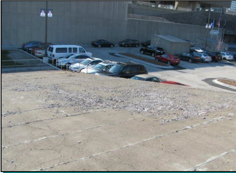
Significant concrete deterioration
