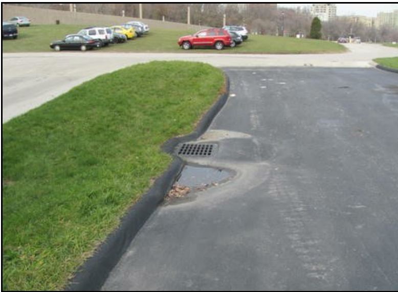
Settlement at catch basin
