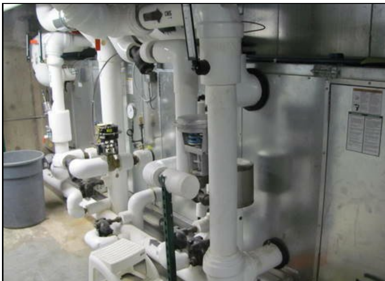
Make-up air unit serving offices
