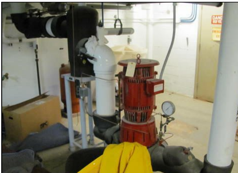
Heat recovery pump
