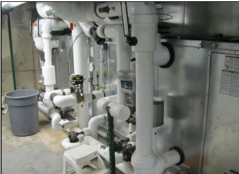
Recently replaced air handling unit serving Kahler offices
