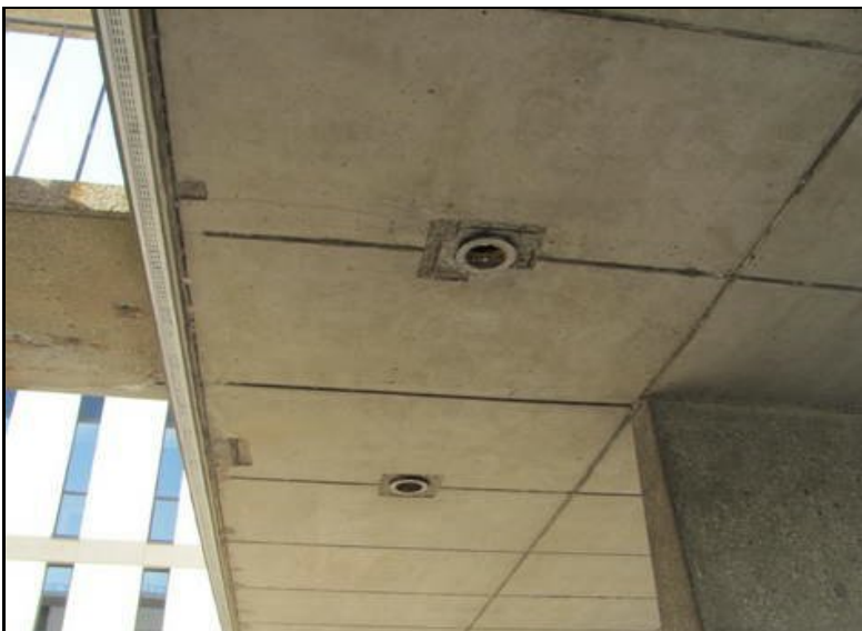
Light fixtures illuminating Veterans Courtyard
