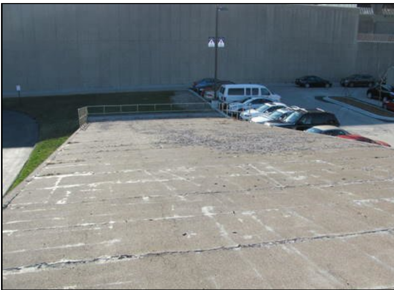
Significant concrete deterioration
