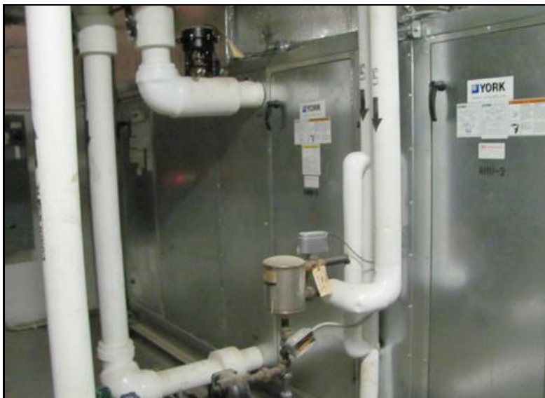
Recently replaced air handling unit serving Kahler museum
