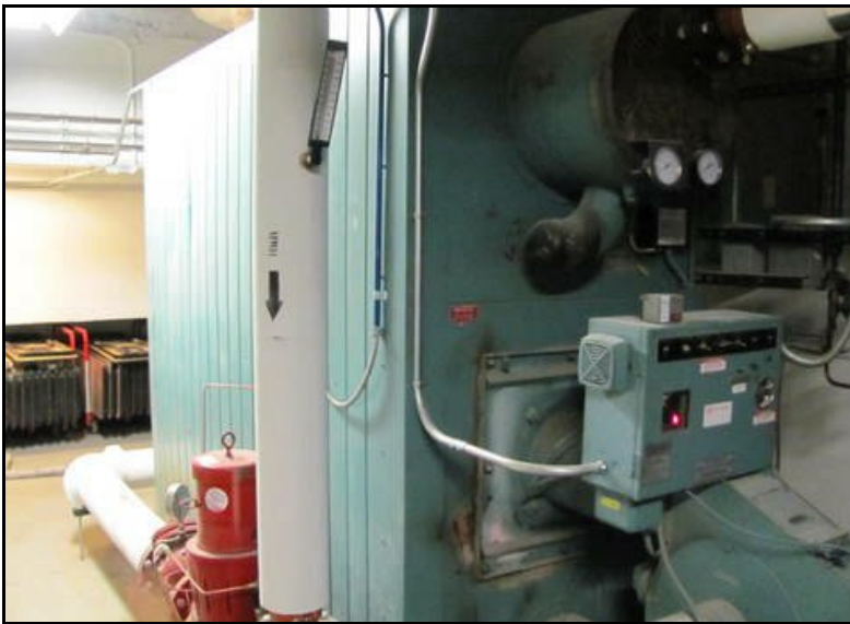
Domestic water boiler
