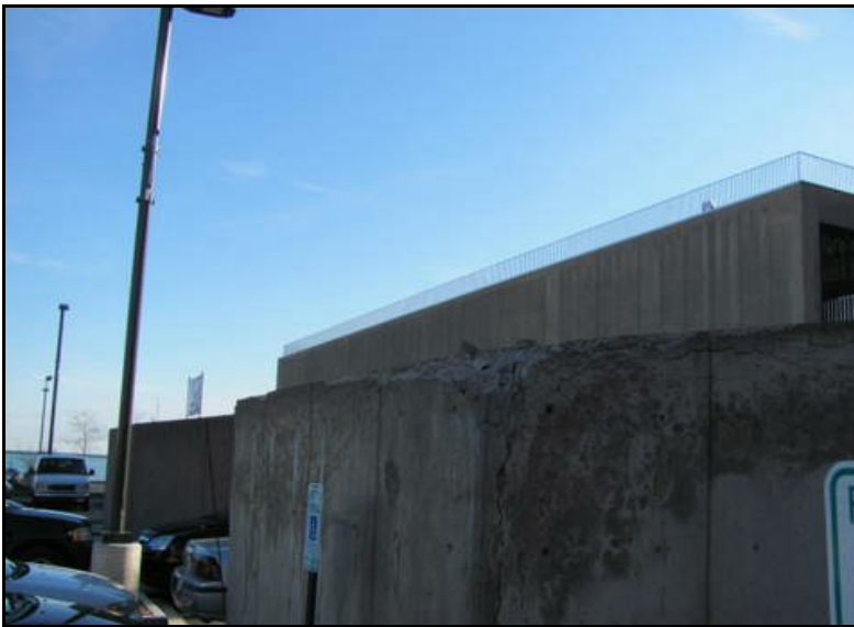
Significant concrete deterioration
