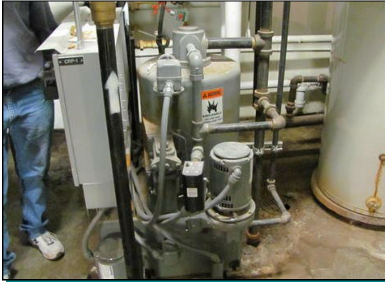
Condensate return system
