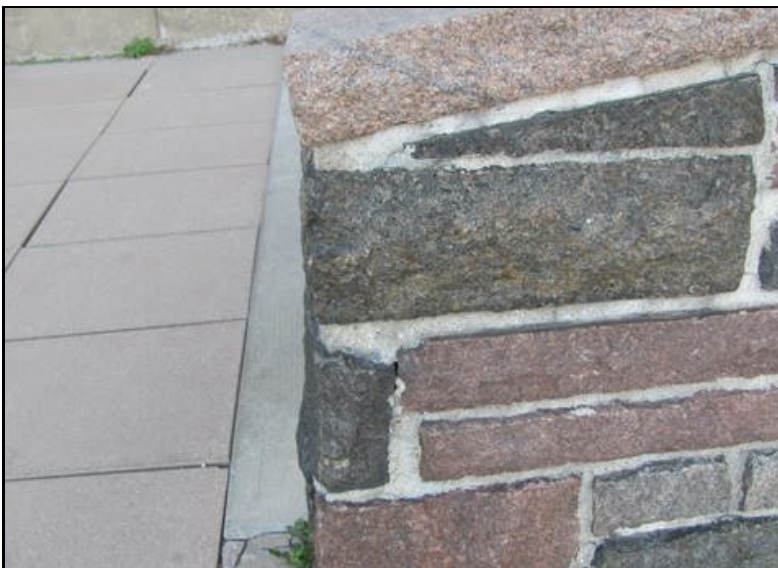
Mortar with voids
