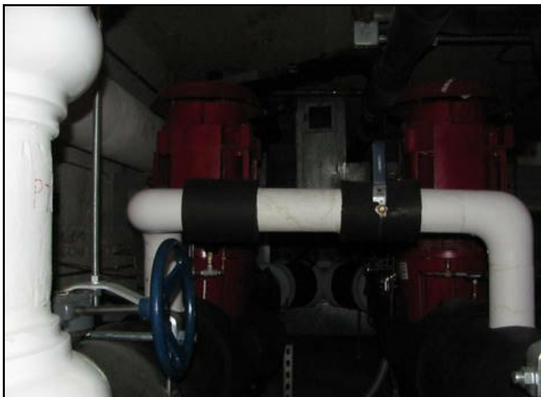
Lake water pumps
