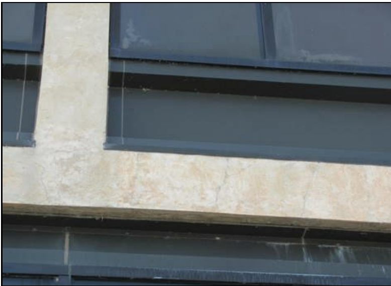
Minor cracks in Kahler concrete
