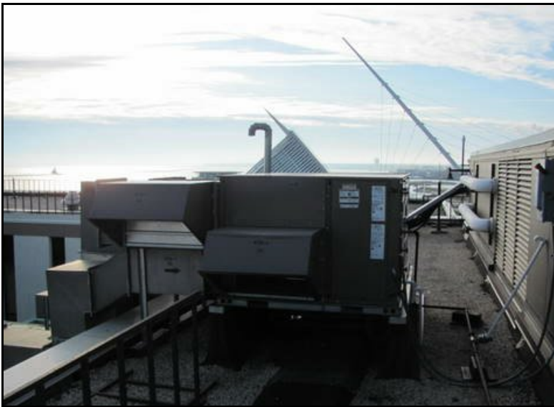
Rooftop heating and cooling unit serving bird cage stairs
