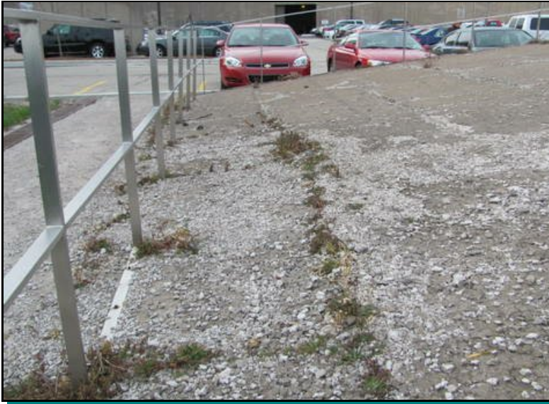
Significant concrete deterioration
