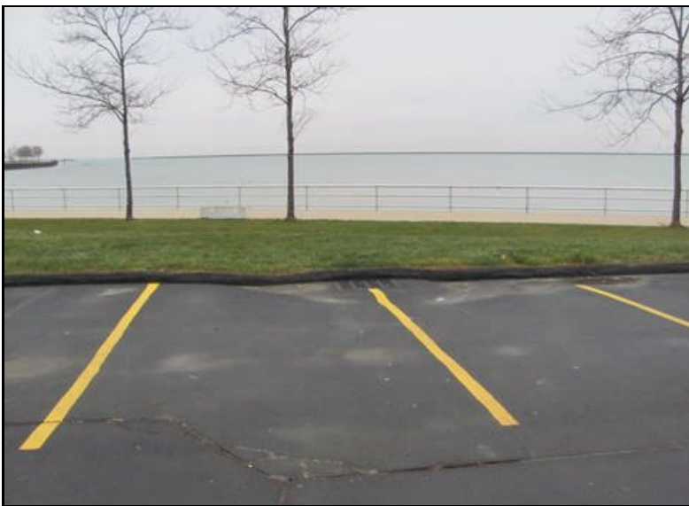
Settlement at catch basin
