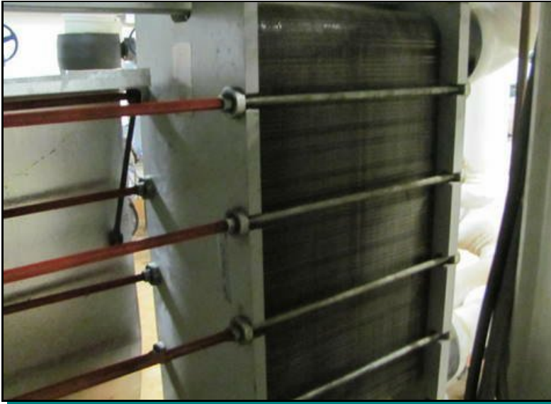
Lake water heat exchanger
