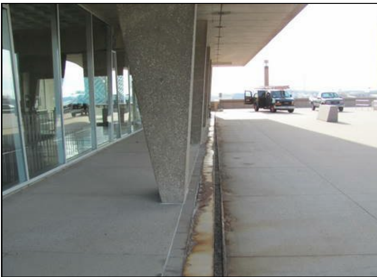
Deterioration at west expansion joint
