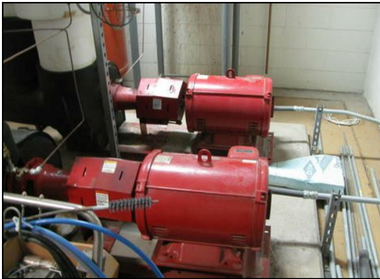
Chilled water pumps
