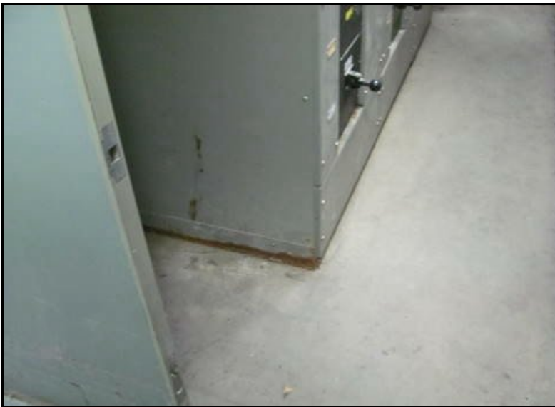
Rust at electrical equipment shell
