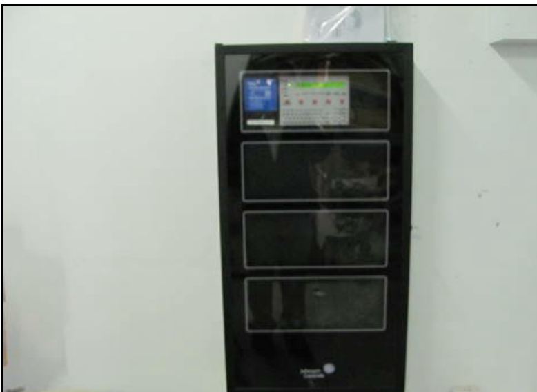
Fire alarm panel
