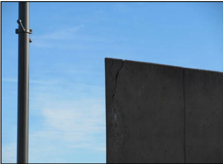
Significant concrete deterioration
