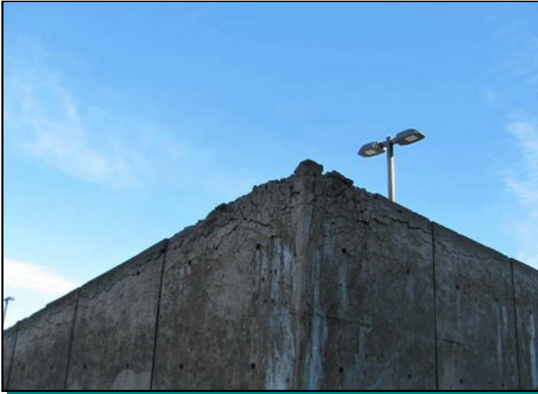
Significant concrete deterioration
