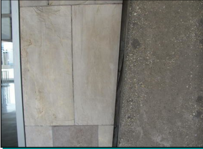
Mortar deterioration at Veterans Gallery stone panels
