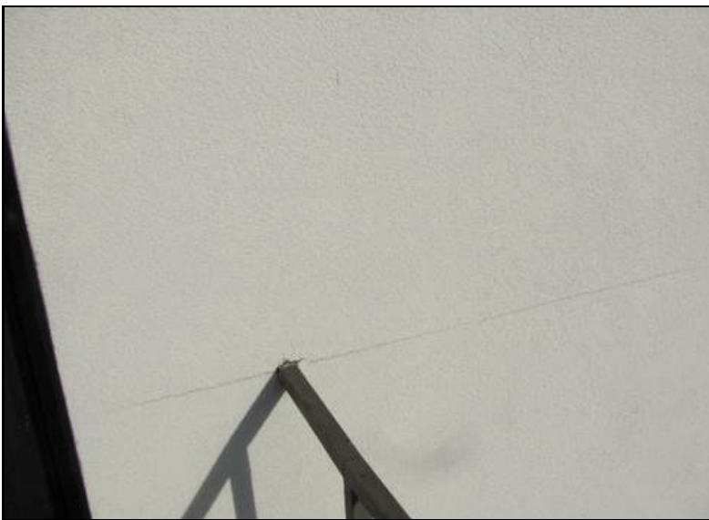
Crack in EIFS
