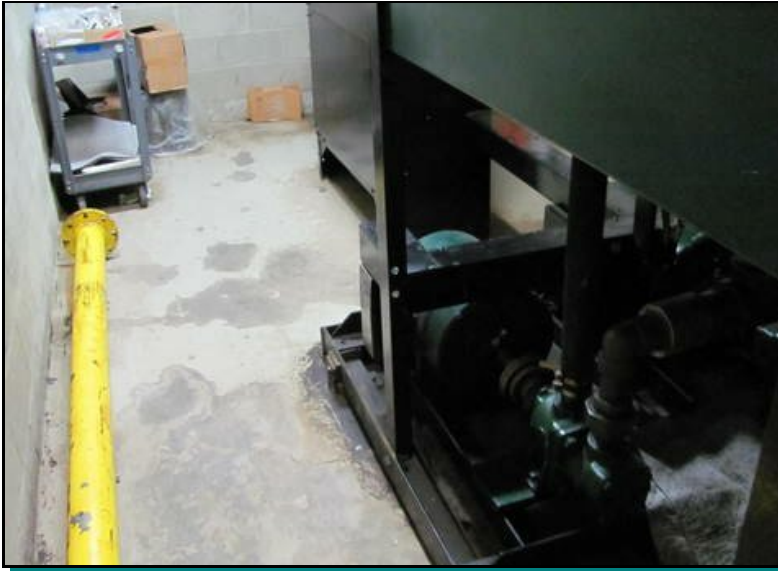
War Memorial freight hydraulic elevator equipment
