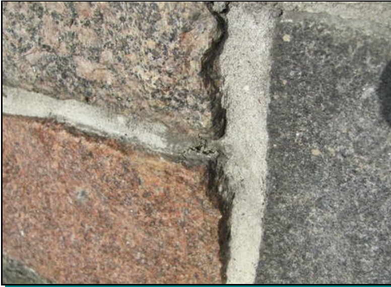
Mortar with voids
