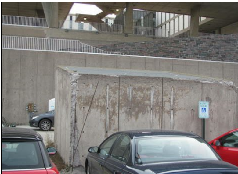
Concrete deterioration at exhaust chamber
