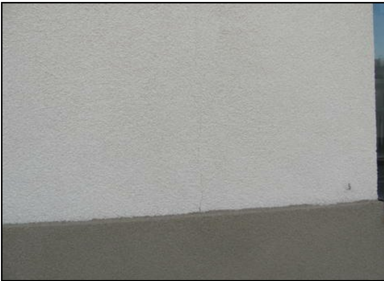
Crack in EIFS
