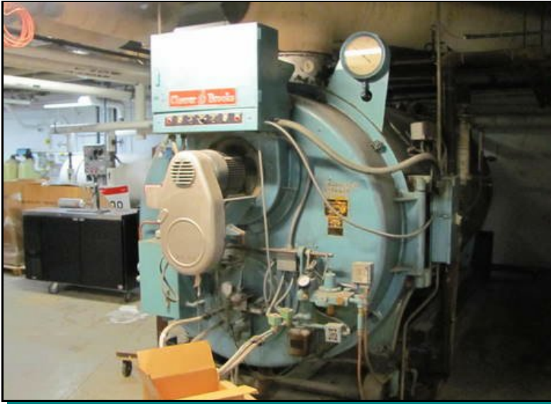
Building heat boiler
