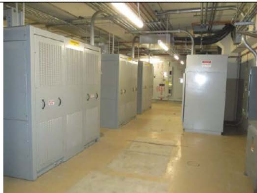
New Electrical Switchgear
