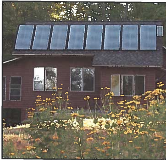
Residential solar hot water collectors
