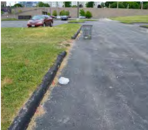
Incomplete and Deteriorating Curb
