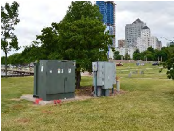
Electrical power transformer
