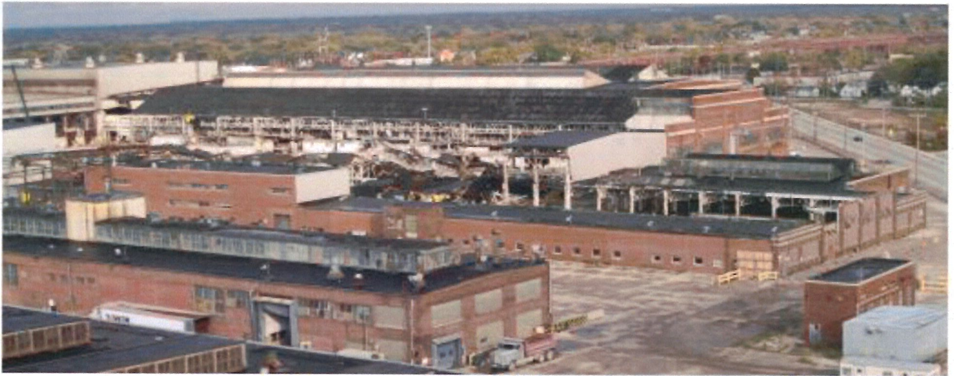
Former Tower/ A.O. Smith site in October 2009. Note Building 37 (center) is collapsing. (City of Milwaukee)
