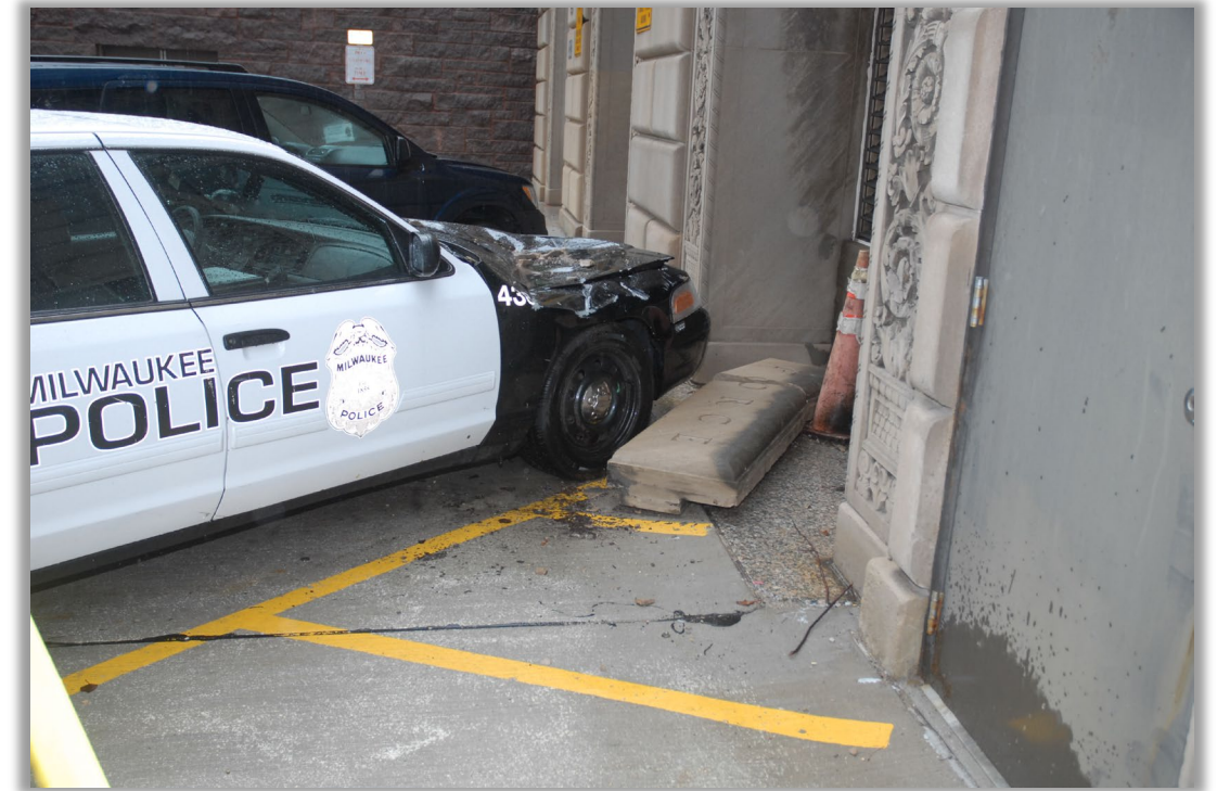
Example of deferred maintenance impacts at the Public Safety Building
