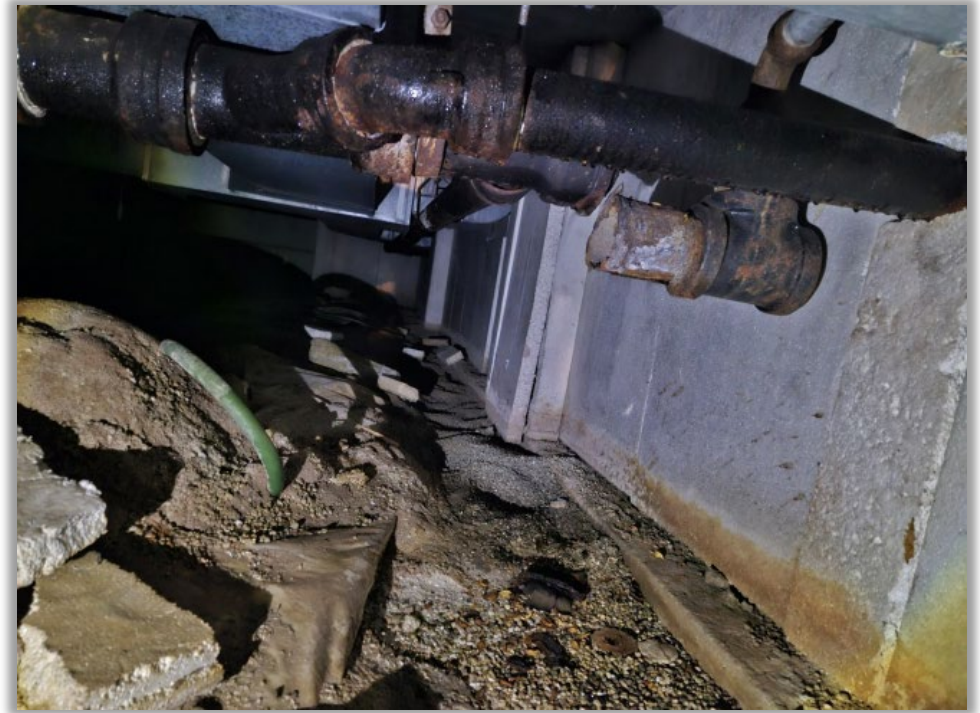
Failed internal storm sewer system at McGovern Senior Center
