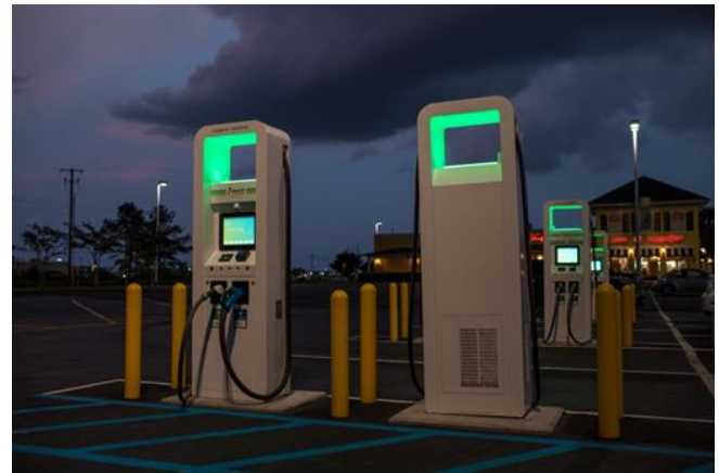
Figure 4 - DC Fast Charging Station
