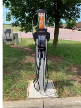
Figure 2 - Level 2 Public Charging Station
