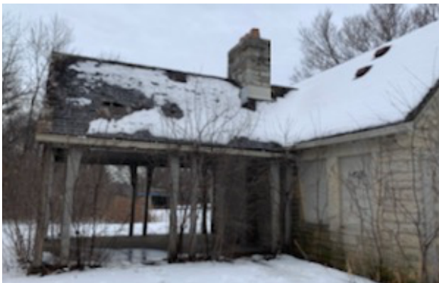
Milwaukee County Parks are home to a number of dilapidated pavilions that cannot be used
