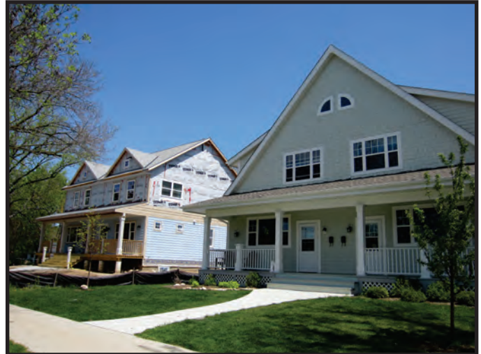
A new duplex and a second nearing completion on a redevelopment site in the City of Waukesha. Construction of the duplexes was sponsored by Habitat for Humanity.
