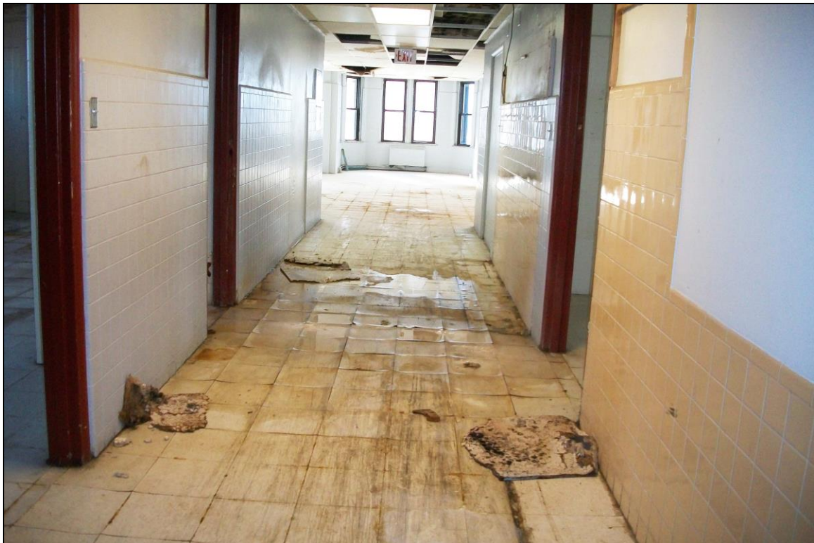
Damage On 5 th Floor From Leaking Roof
