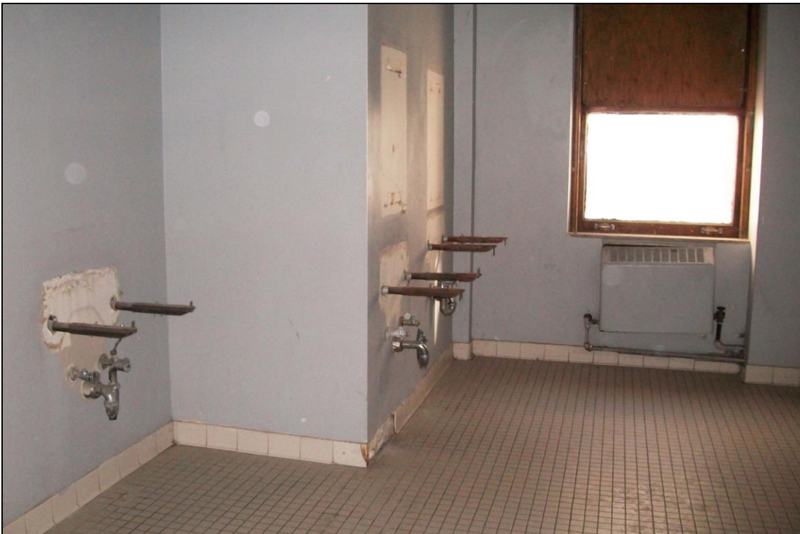
Shared Bathroom With Missing Plumbing Fixtures
